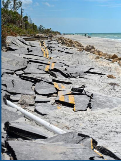
Roadway Damage after Hurricane Idalia
