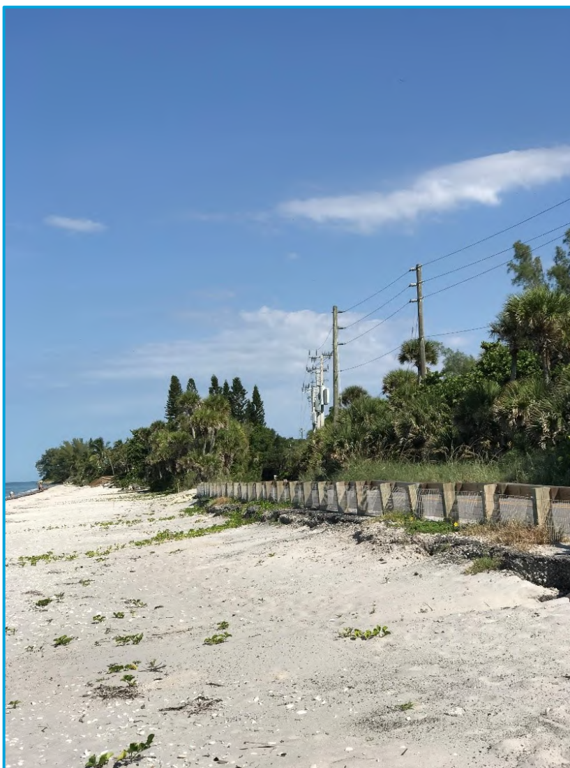
Figure 3-7 - Erosion along beach front side of Manasota Key Road (September 2019).
