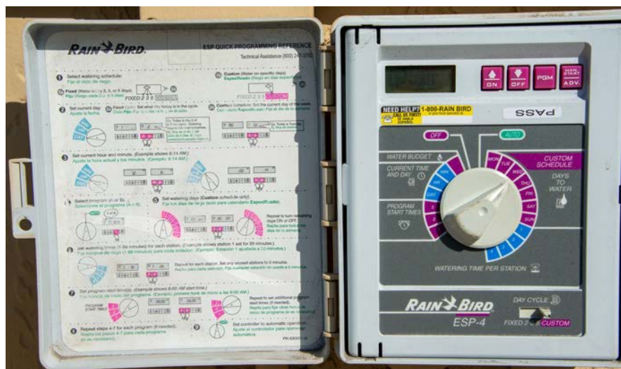
▲ Irrigation control box | David Shafer.
