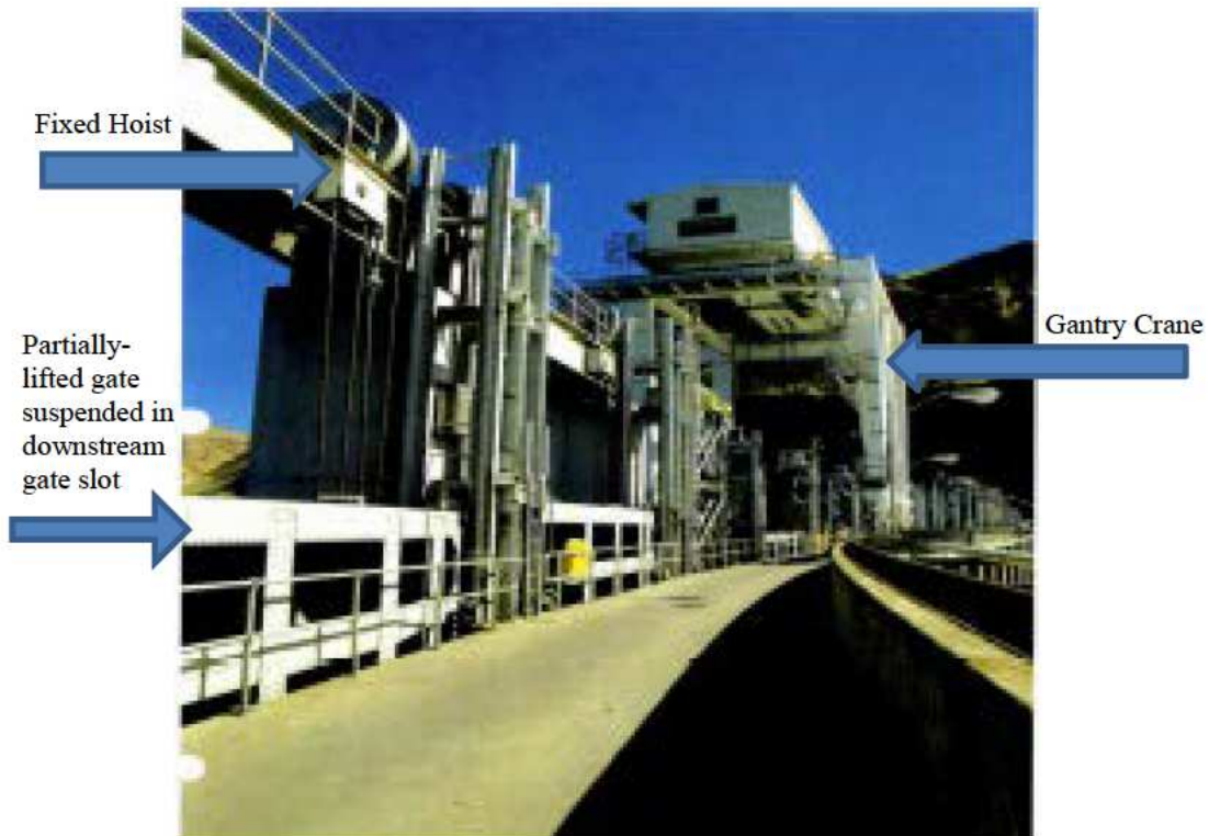
Photo No. 1 - View of spillway bays along spillway deck. The spillway bay in foreground is outfitted with a fixed hoist while a gantry crane is positioned over bay/gate in background.
