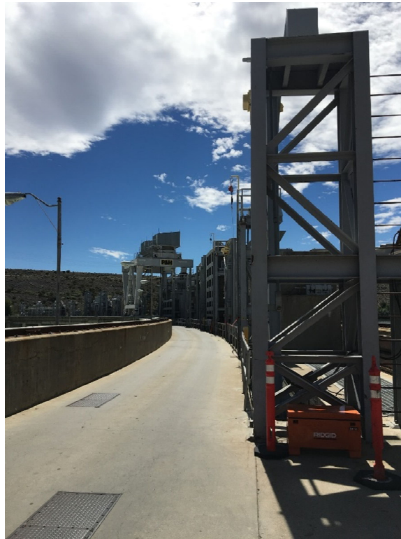
Photo 1: Rock Island Dam Deck Supports Multiple Stanchions for Removal and Storage of Segmented Lift Gates
