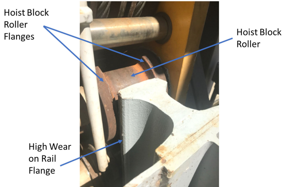
Photo 8: Gate Bay 17 North Stanchion After Incident (Gantry Crane 3 Hoist block Is Not Engaging the Downstream Fixed Rail)
