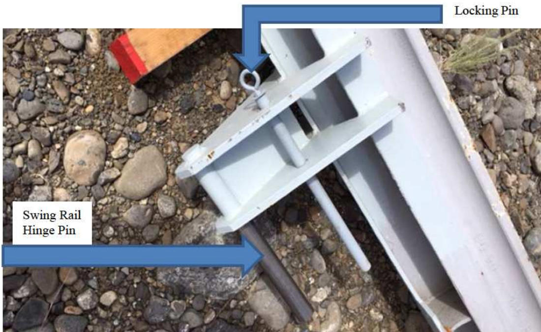
Photo No. 4 - Gate 17's north swing rail lower hinge assembly with hinge pin (left) and locking pin (right). The swing rail was removed from the spillway after the incident and relocated to a maintenance yard adjacent to the Dam.
