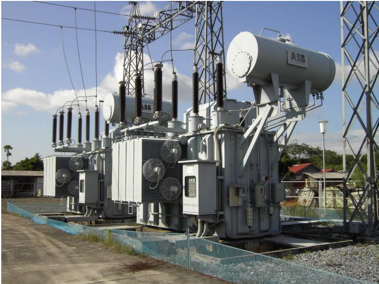
Picture (6) Substation Transformer 6
