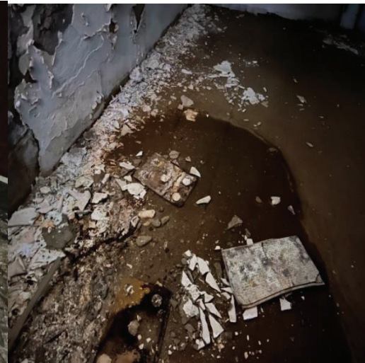
Photo #4 – Water Infiltration
