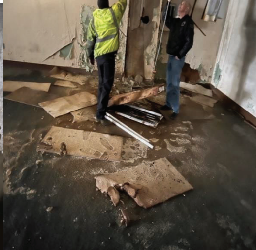
Photo #2 – Water Infiltration
