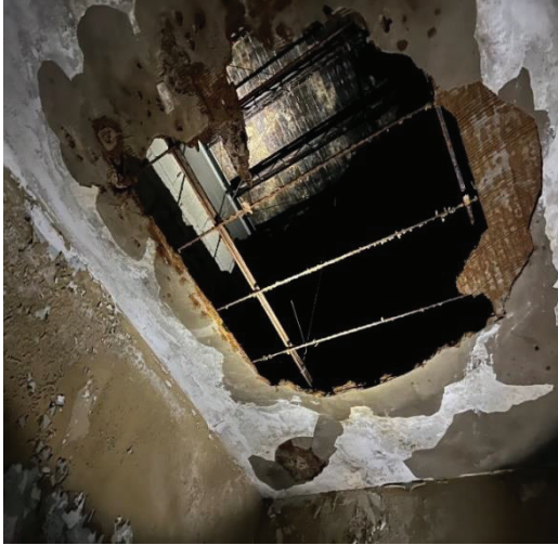
Photo #1 – Water Infiltration
