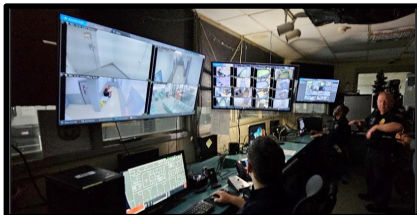
Exhibit 40: Central Control CCTV System
