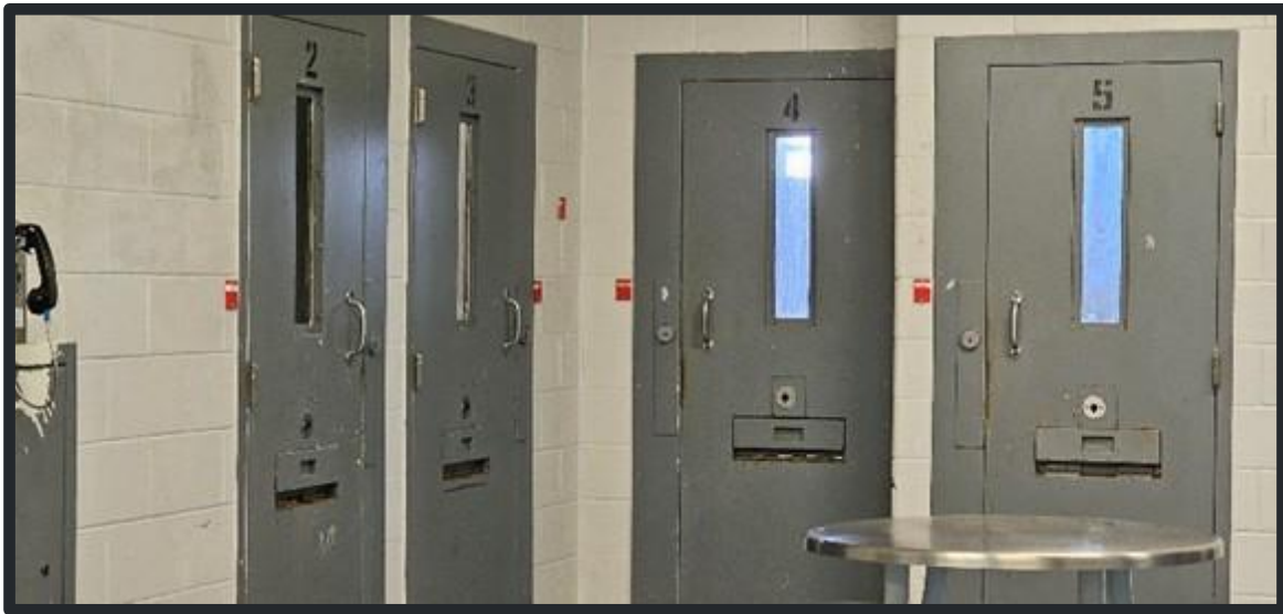
Exhibit 38: Automated Accountability System Placed at Cell Door Fronts
