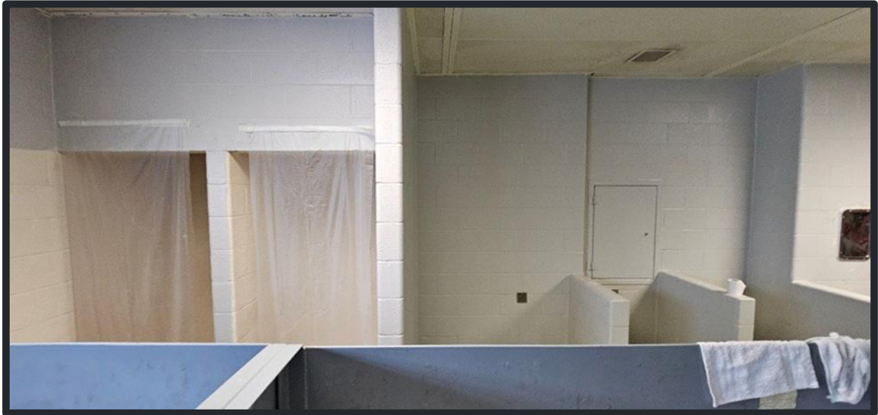
Exhibit 45: Proximity of Showers and Toilets to Bunk Beds
