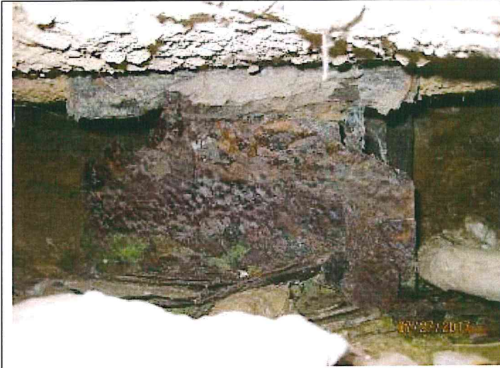
Photo 1: Approximately 30% section loss in south most pile under west abutment. The front flange is corroded through with the back flange and web with minor section loss. Remaining piles have minor section loss.
