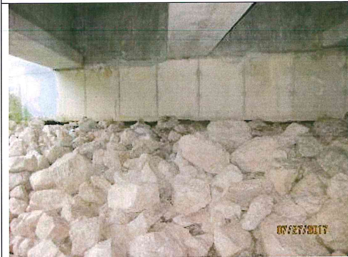
Photo 2: Settlement of rip rap on south west side exposing piles under the abutment.
