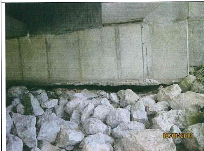
Photo 3: Settlement of rip rap on north west side exposing piles under the abutment.
