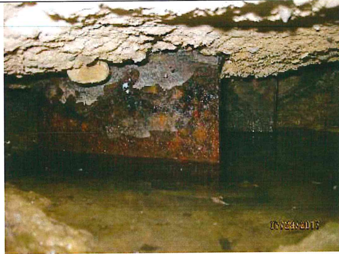
Photo 5: 1 st pile on north side, east abutment. Flaking rust with minor section loss. Standing water.
