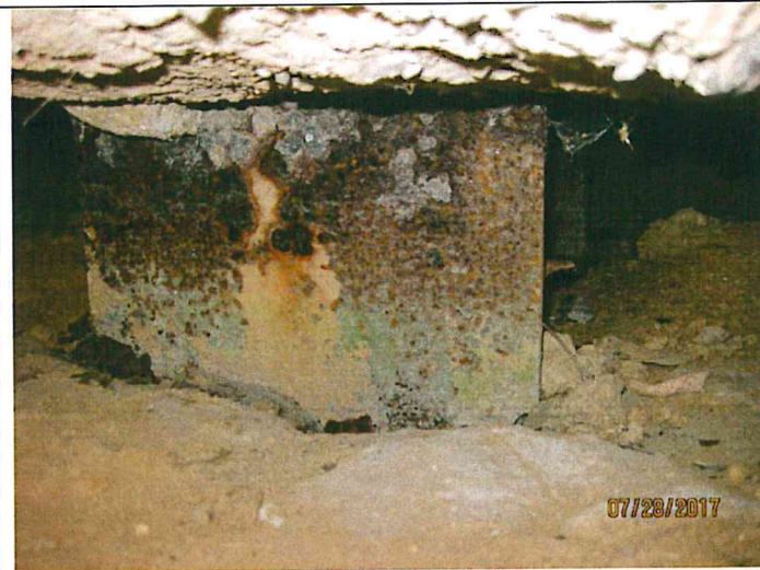
Photo 6: 2 nd pile on north side, east abutment. Flaking rust with minor section loss.
