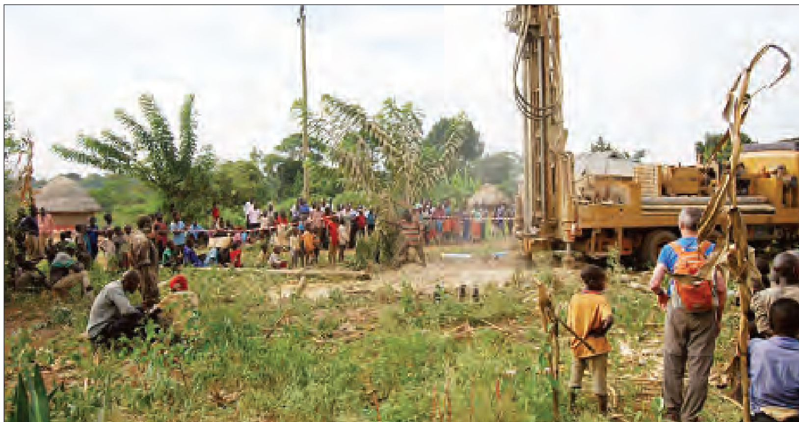
Villagers look on during the drilling a bedrock supply well in Uganda.
