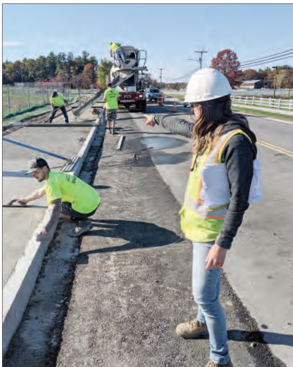
Engineers spend significant time in the field ensuring designs are built safely, accurately and in full compliance with codes, permits and funding requirements.
