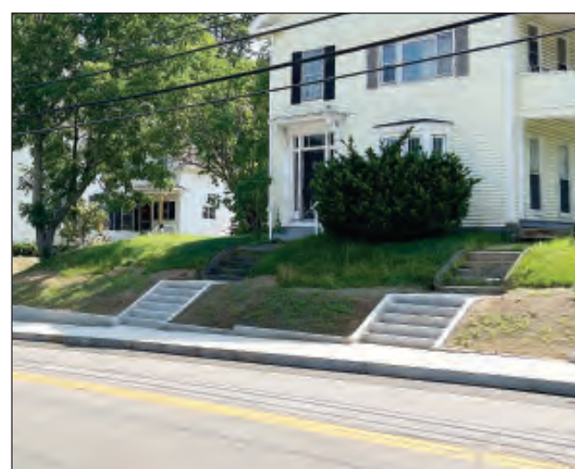
Before and after: Engineers helped turn this aging sidewalk, top, into a safer, more accessible route for pedestrians, improving everyday mobility in the community.
