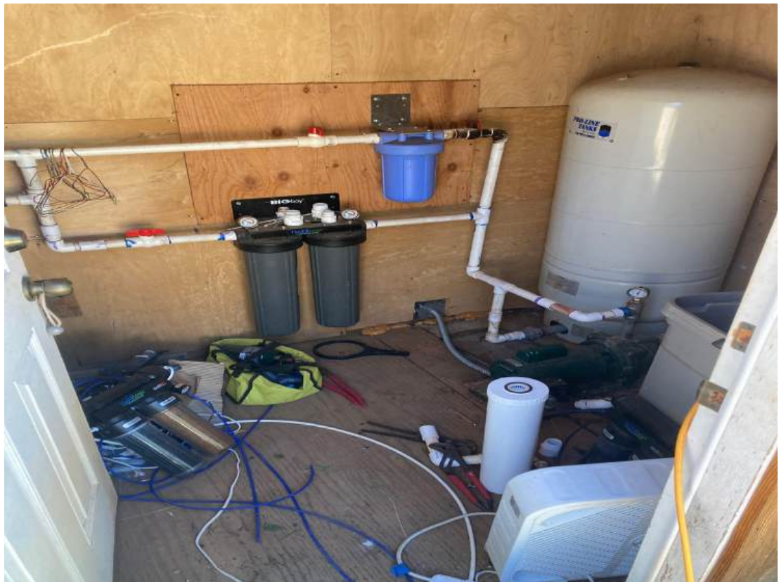
Figure 1: The Water System On-Site That Delivers Water to the Storage Tanks.
