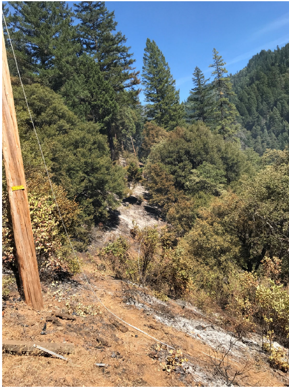
Figure 1: A portion of the downed TPUD south line between poles #012497 and #012498
