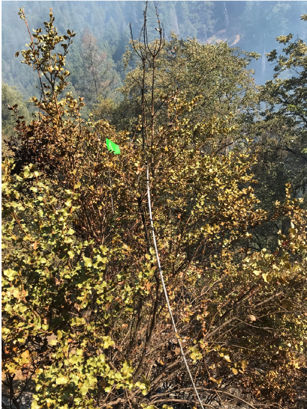
Figure 2: The downed TPUD powerline on bush with electrical resistance scar
