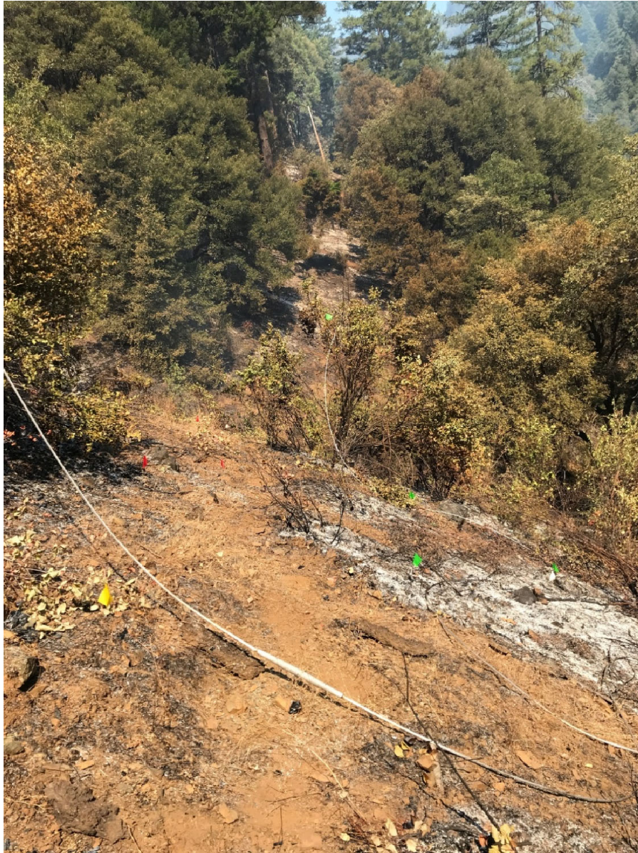
Figure 3: Downed TPUD powerline with green flags marking probable ignition sources
