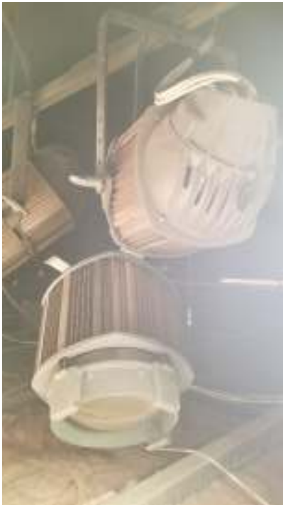
1. Several Fixtures unusable
