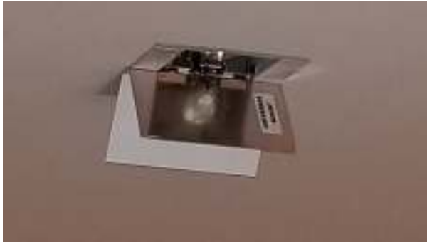
Emergency Light w/ doors open
