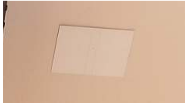
Emergency Light w/ doors closed
