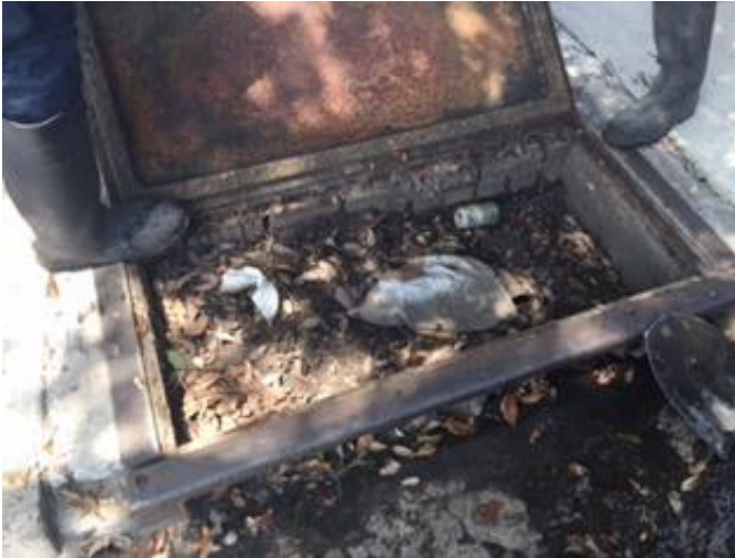
Catch basin in need of an interior clean
