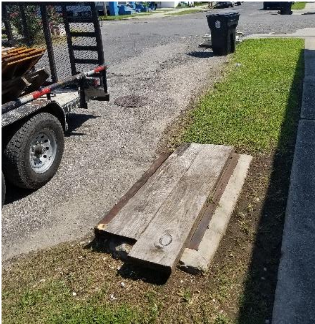
Catch basin missing a lid, replaced with plywood
