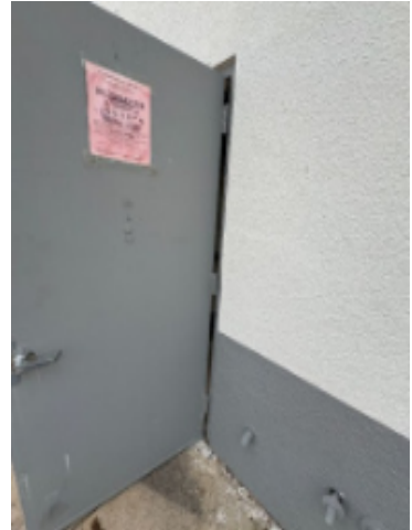
Riser 3 Knox Box Needed
