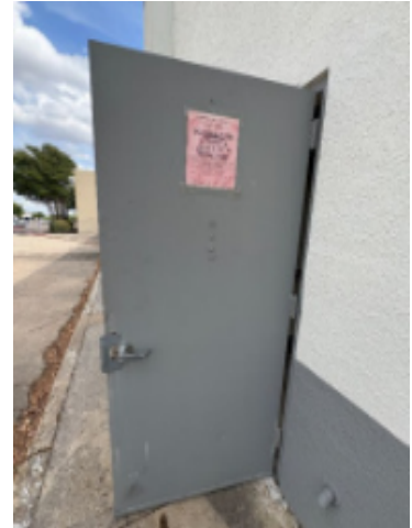
Riser 3 Signage Needed
