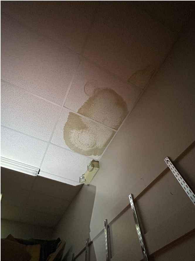
Photo 9 - Staining across ceiling tiles near lighting and an emergency light. Source: IMG_2648.JPEG.
