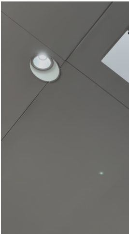
Photo 5 - Interior ceiling and recessed light.
