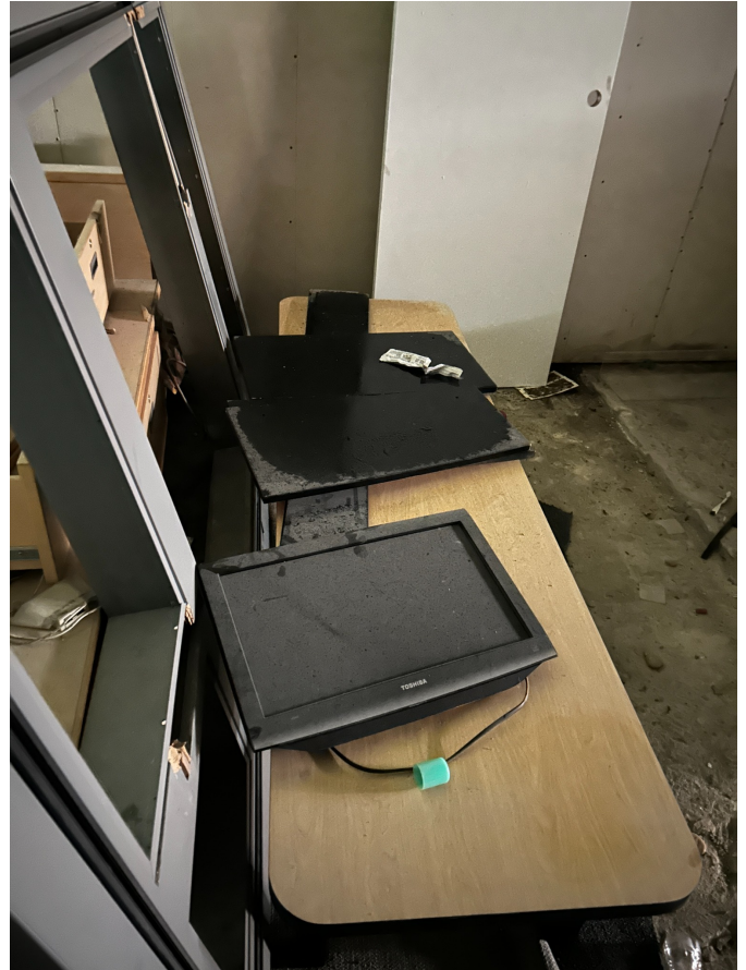
Photo 8 - Moisture visible on equipment and surfaces in an interior storage area. Source: IMG_2643.JPEG.
