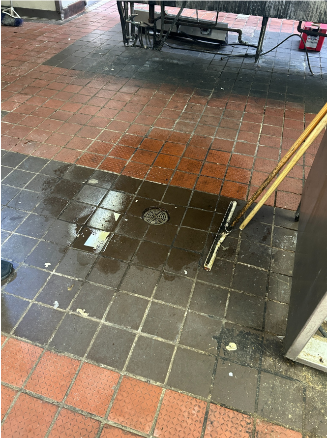
Photo 7 - Water on the tiled floor around a floor drain. Source: IMG_2639.JPEG.
