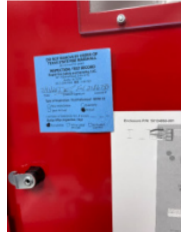
FACP has active alarms
