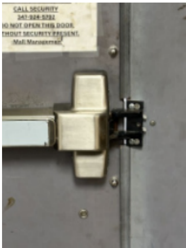
Exit door not operable near Riser 1
