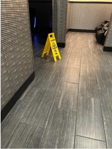
Photo 3 - Wet-floor warning in an interior circulation area.
