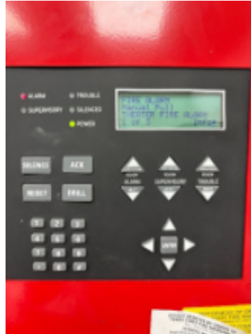
FACP has active alarms
