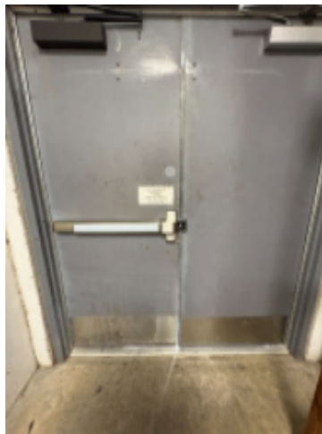
Exit door not operable near Riser 1
