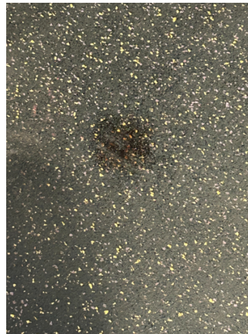
Photo 2 - Darkened area on flooring.
