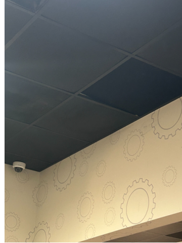
Photo 4 - Interior ceiling with an open ceiling panel area.
