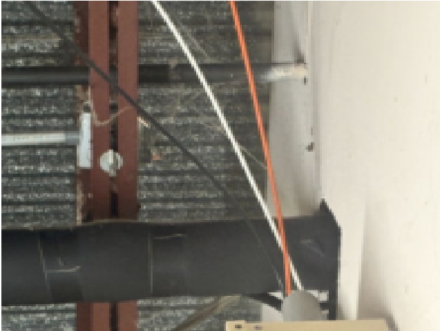
Extension cord in service hallway
