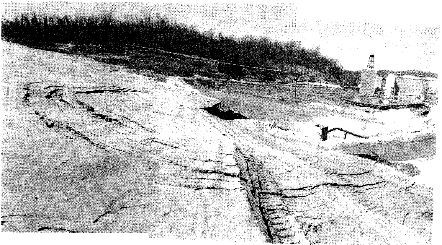
Photo No. 2 – Photo of sinkholes and depression that formed on April 4, 2014, taken on April 5, looking northwest. Note the muddy mine water discharge into pond with similar color as residual soil exposed on hill in background.
