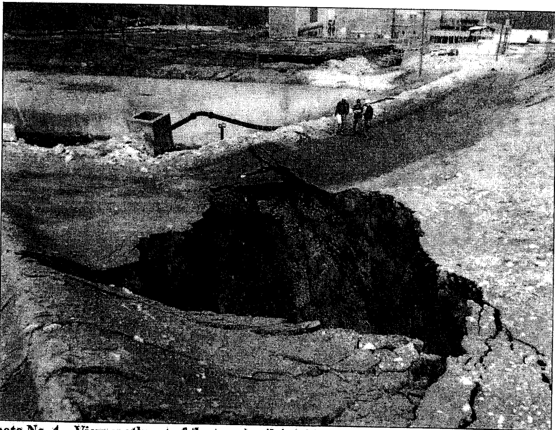
Photo No. 4 – View southeast of the two April 4 sinkholes, photo taken late April 6.
