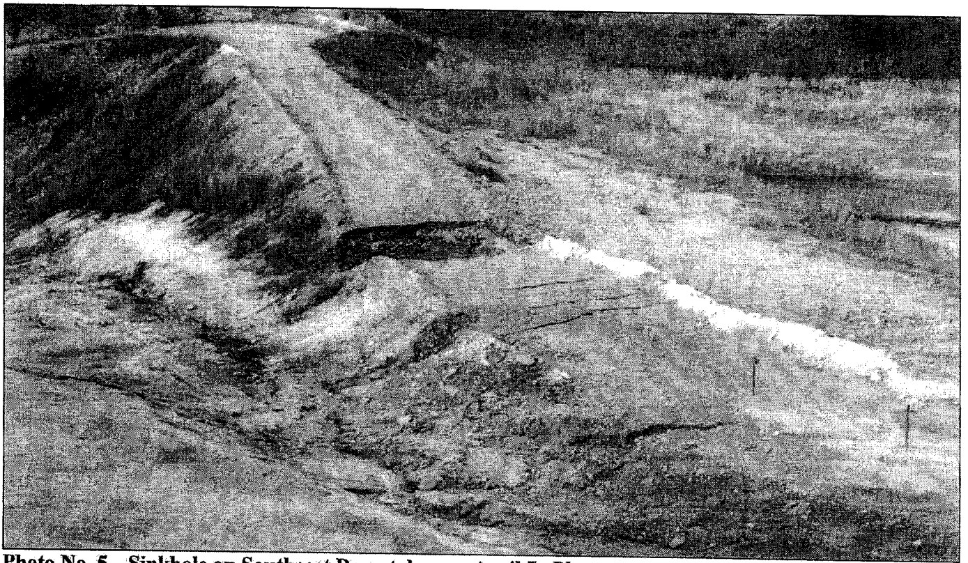
Photo No. 5 – Sinkhole on Southeast Dam, taken on April 7. Photo courtesy of J. Knudsen, Tierra Group
