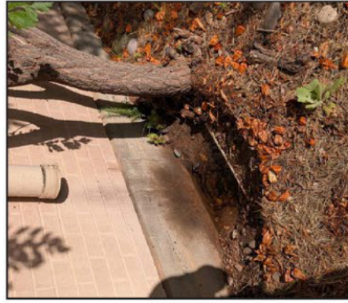
2) Roof Water Infiltration into Foundation
