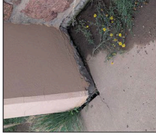
5) Settlement of Exterior Slab
