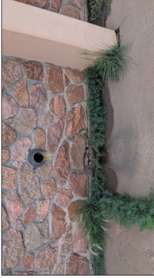
1) Roof Water Infiltration into Building Foundation
