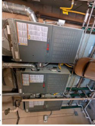
5) Mechanical Room Equipment
