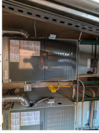
6) Mechanical Room Equipment
