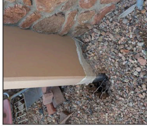
4) Exposed Building Foundation
