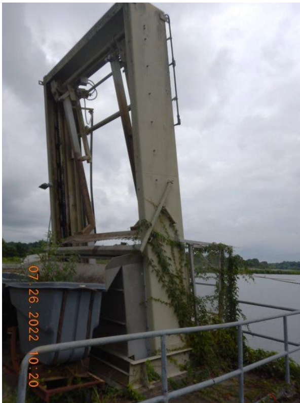
Photograph 4. Bar screens and vegetation growing alongside the structure.
