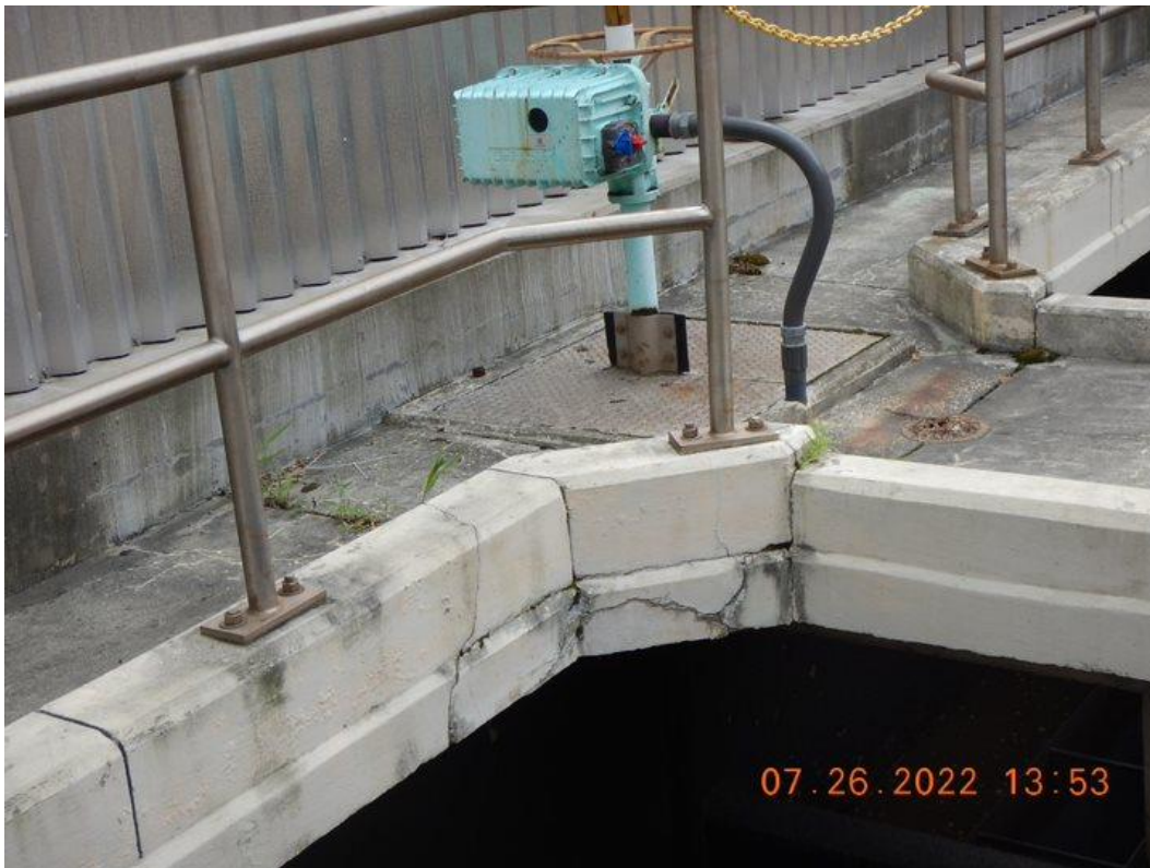
Photograph 29. Cracking above influent valve of Filter 16.
