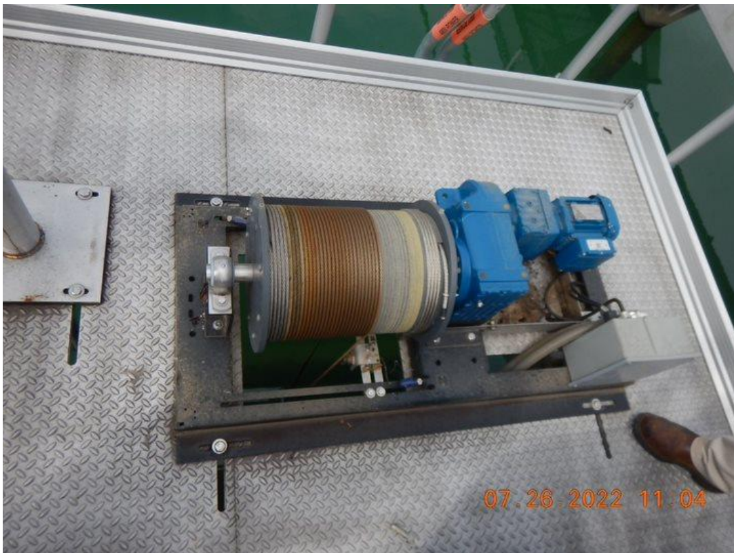
Photograph 21. Solids residual collection system, cable for the collectors.
