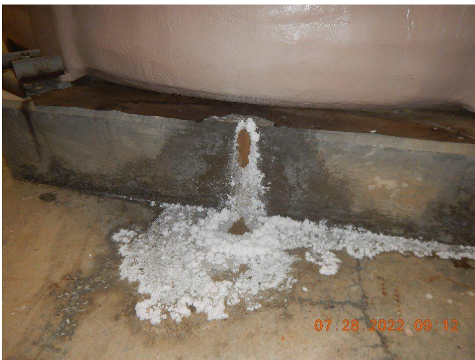
Photograph 118. Floor below active sodium hypochlorite leak at Tank T-SH-1-3 at the West Chemical Building.
