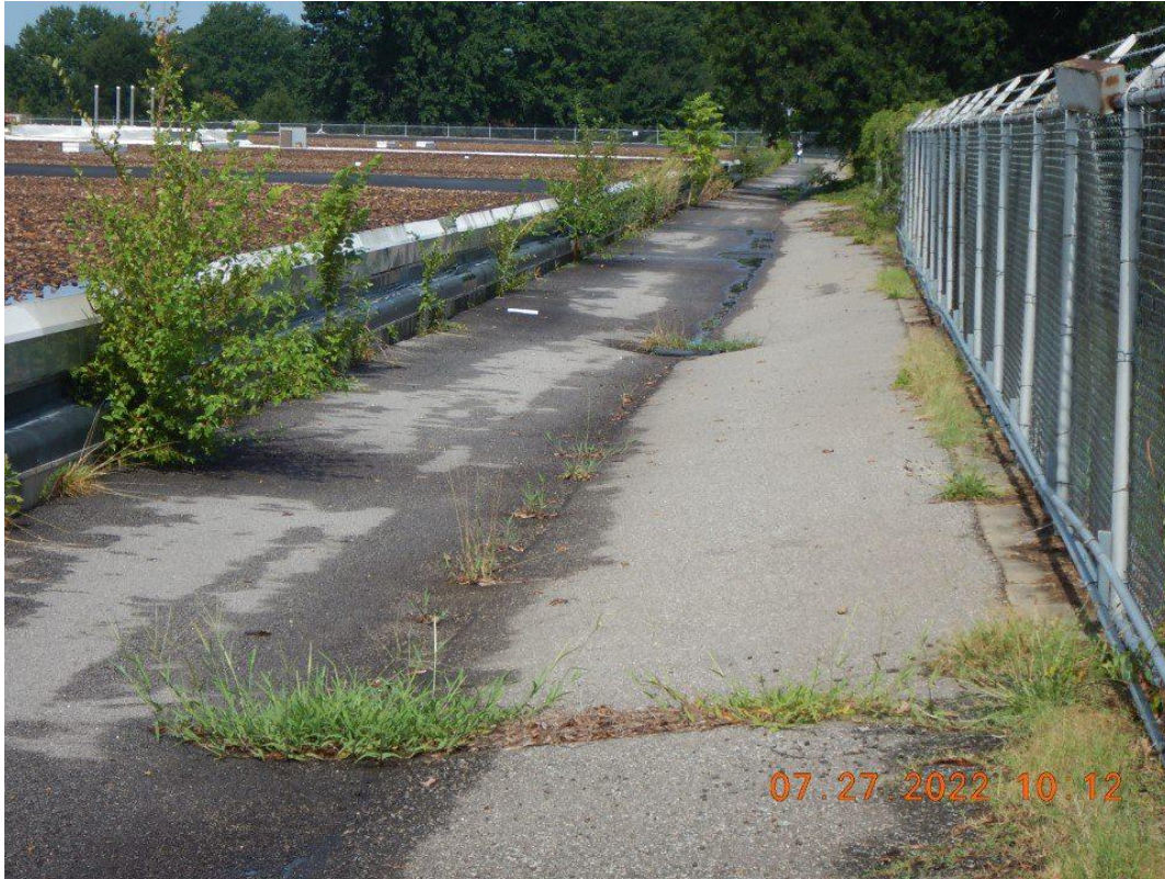
Photograph 63. Plant growth at base of Byrd Park Reservoir.
