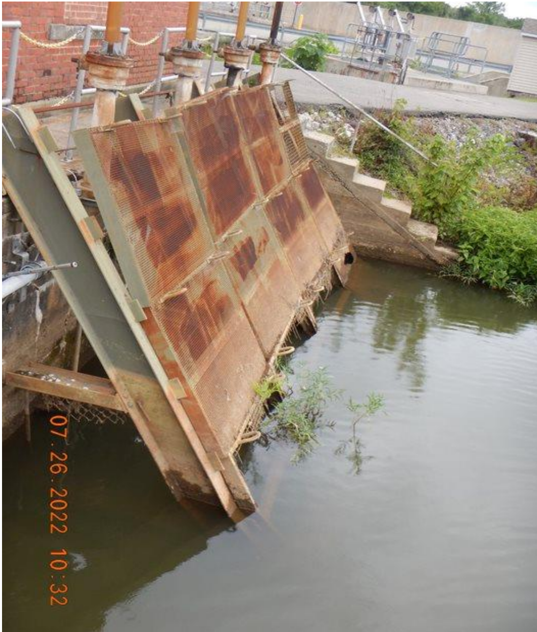
Photograph 11. Out of service screens at raw water intake area.
