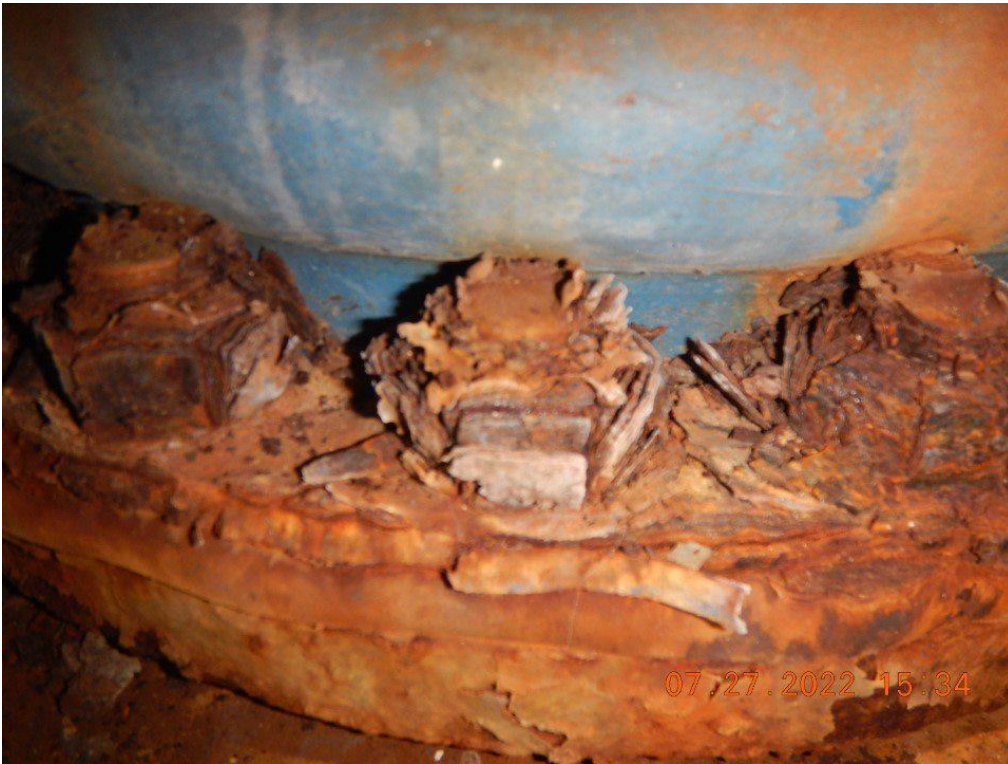
Photograph 115. Corrosion on pump 2 that takes water from the Plant 1 clearwell to the finished water basin.
