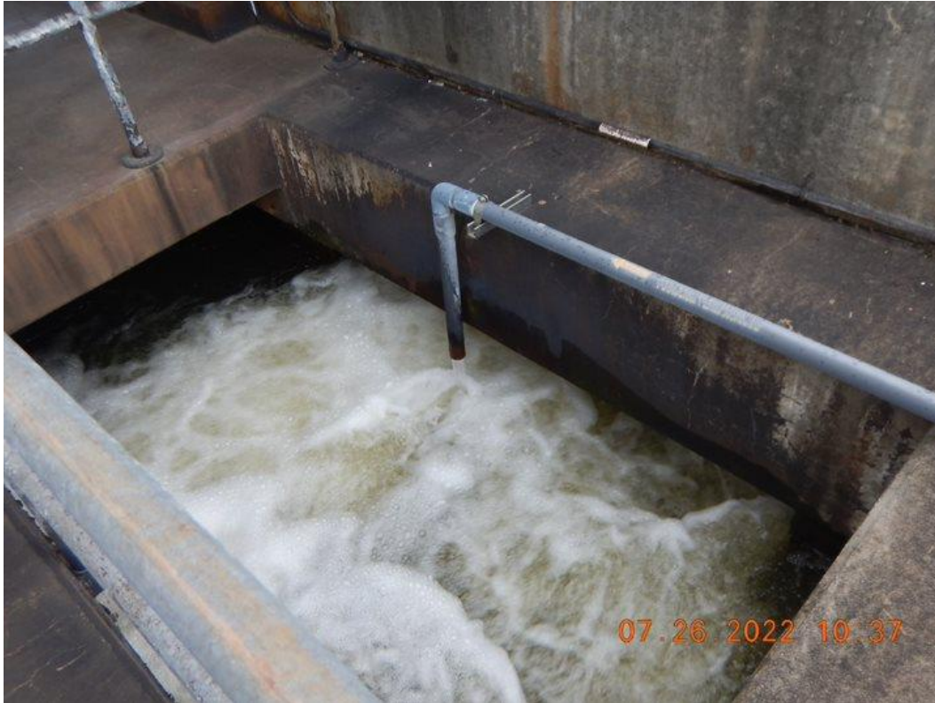
Photograph 14. Potassium permanganate chemical application area, not operating properly since water is clear instead of purple.
