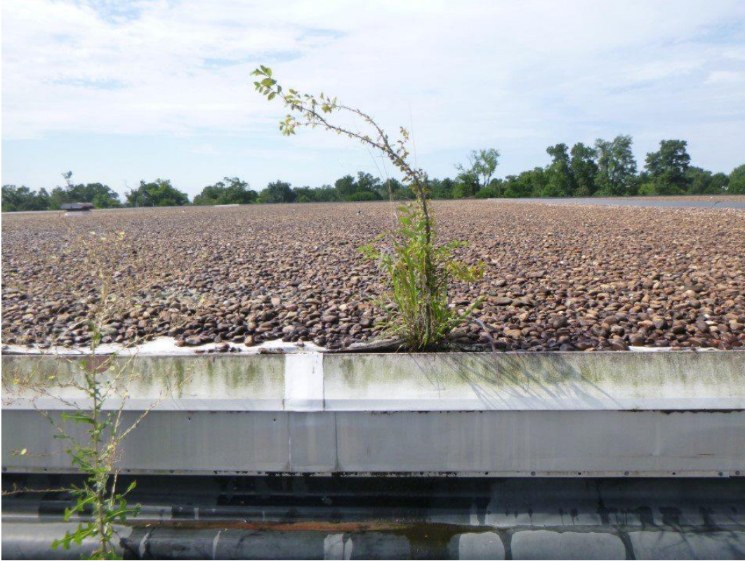
Photograph 55. Vegetation growth on the roof of Byrd Park Reservoir.
