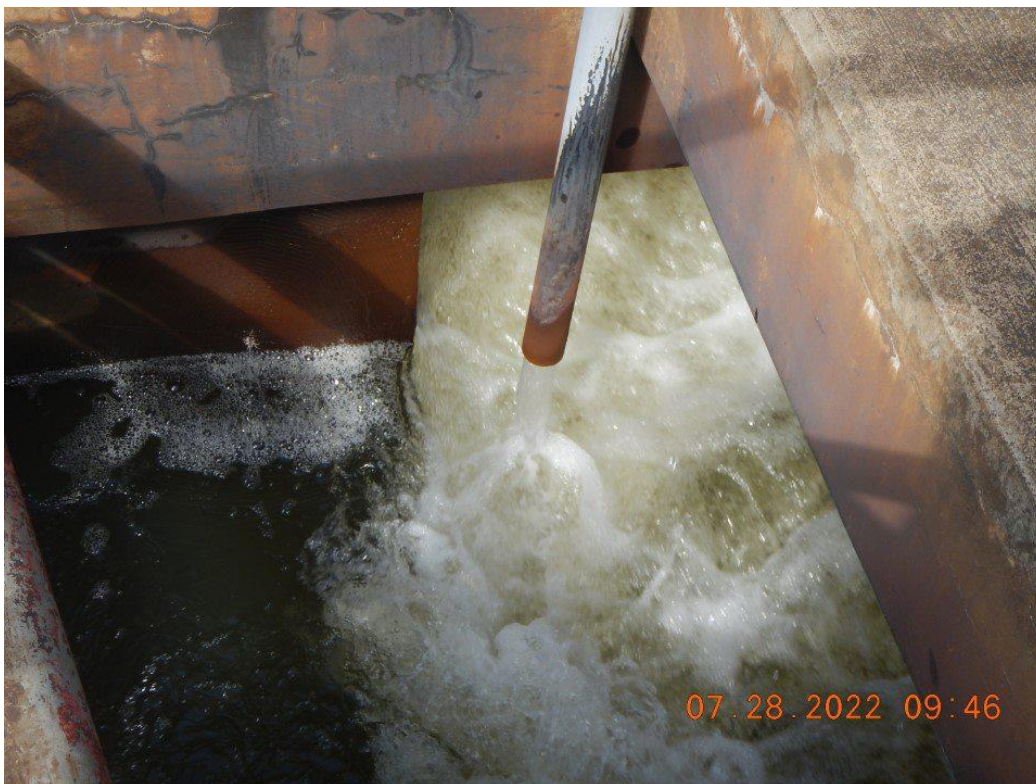
Photograph 125. Potassium permanganate in raw water coagulation channel during Day 2 of inspection out of service with clear water at chemical application point.
