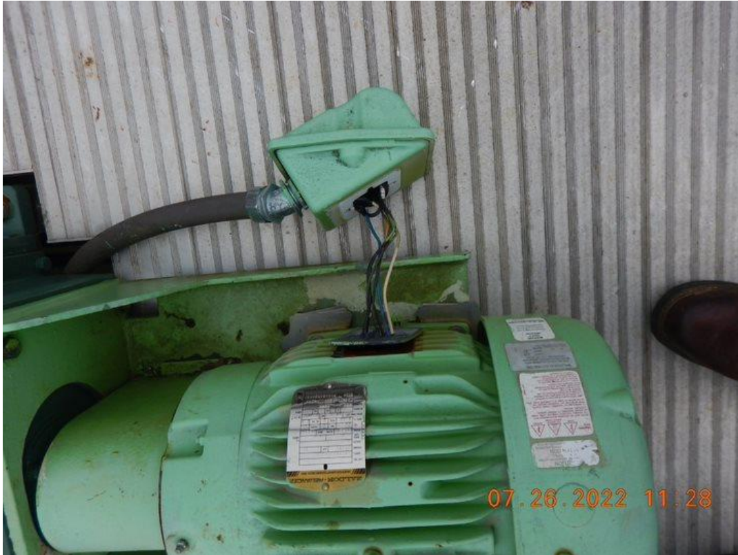
Photograph 24. Exposed wiring at flocculator 4-2A.
