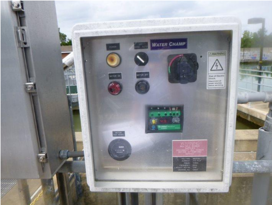
Photograph 17. Water Champ flash mixer controls at Plant 2.
