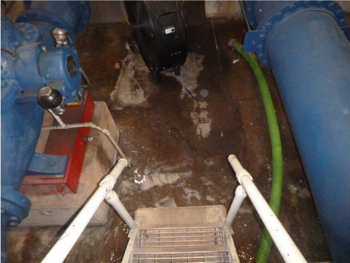
Photograph 45. Water and algal growth on floor of Korah 2 and 3 Pump Station.
