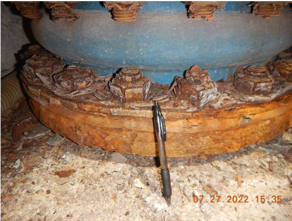
Photograph 116. Corrosion on pump 3 that takes water from the clearwell to the finished water basin in Plant 1 pipe gallery.
