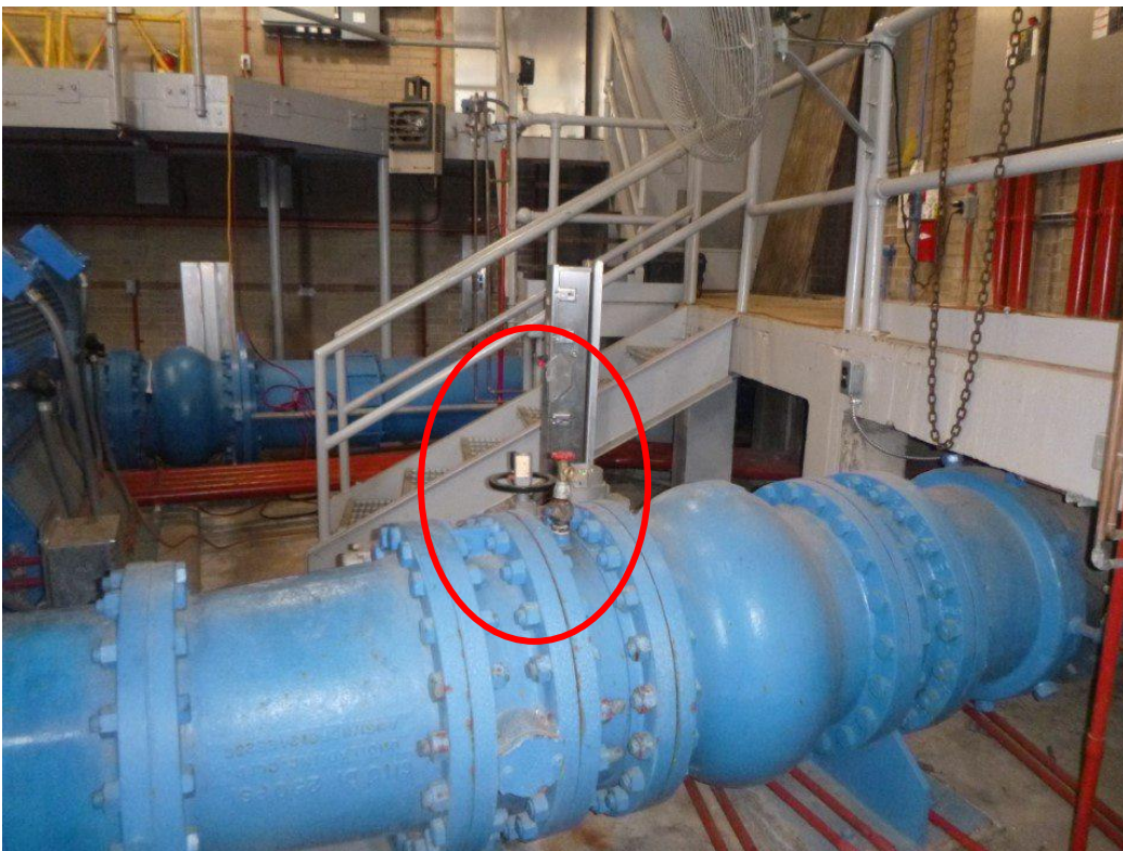
Photograph 92. Threaded tap on finished water line without backflow prevention at the Columbus Pump Station.
