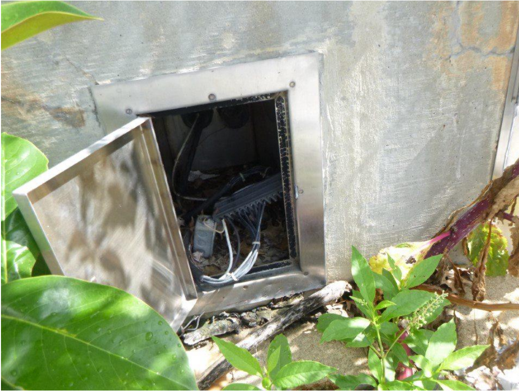
Photograph 69. Opened electric box at end of southern access walkway at Byrd Park Reservoir.
