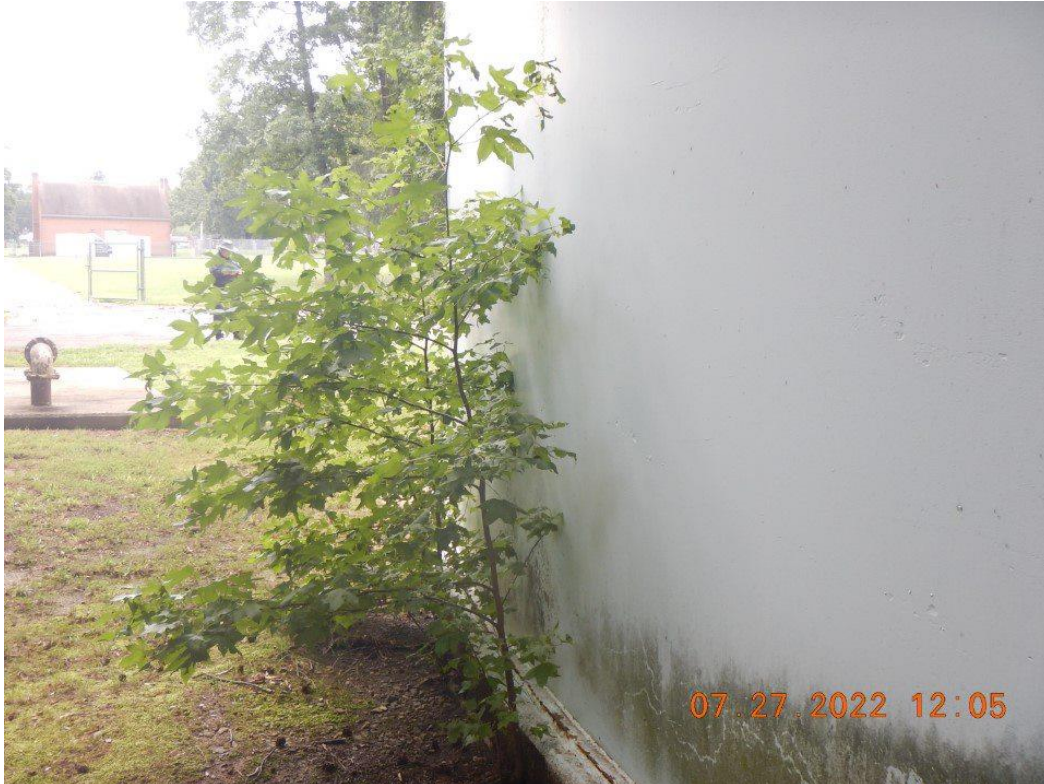
Photograph 74. Vegetation and algal growth at base of Jahnke Road Tank.
