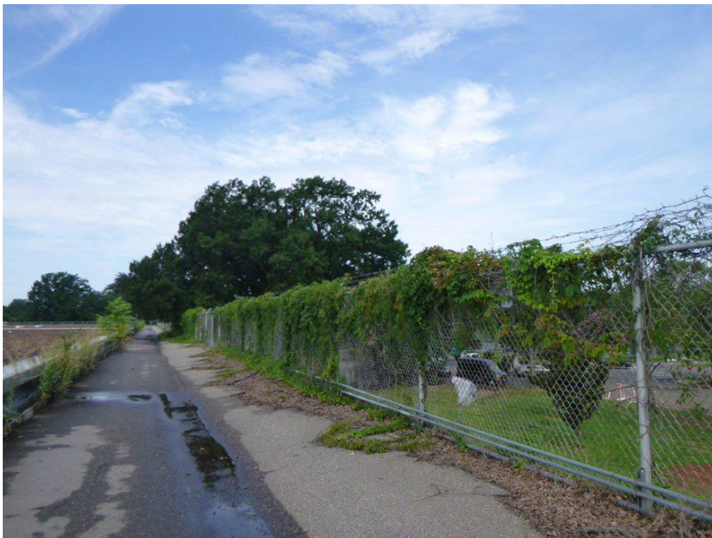
Photograph 52. Fencing and vegetation growth at the Byrd Park Reservoir.
