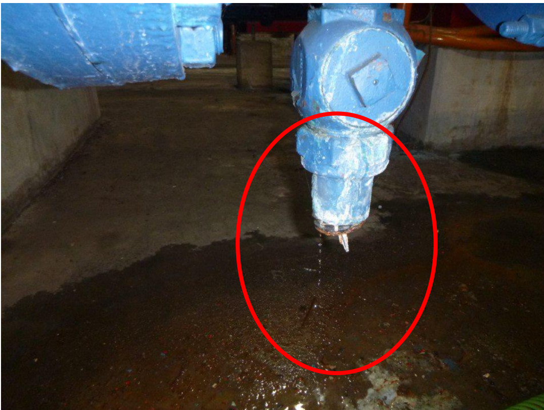
Photograph 48. Leaking fitting from corroded pipe in Korah 2 and 3 Pump Station.
