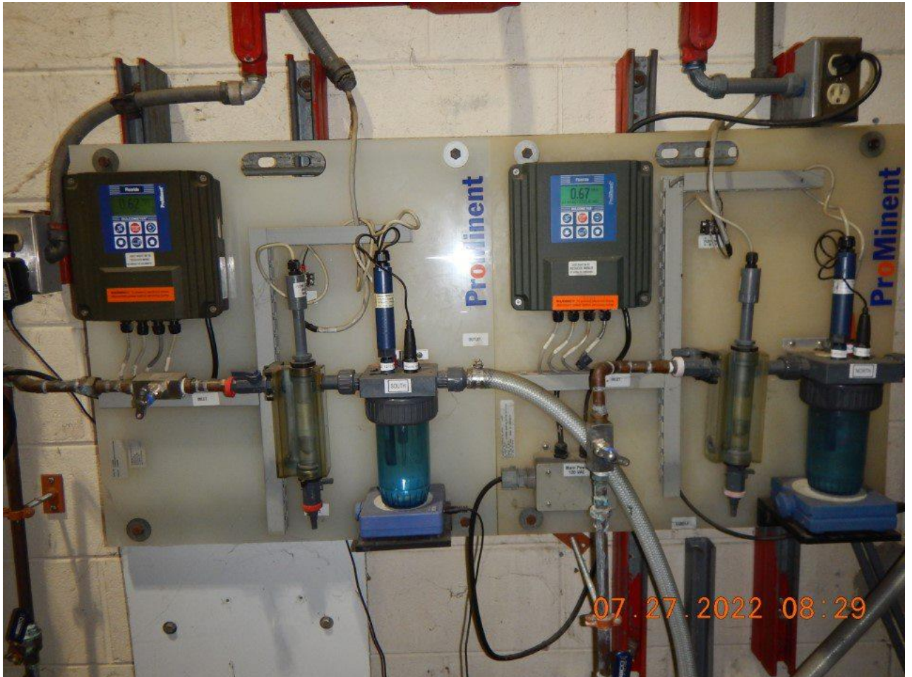
Photograph 40. Korah 2 and 3 Pump Station – ‘north’ and ‘south’ fluoride analyzers.
