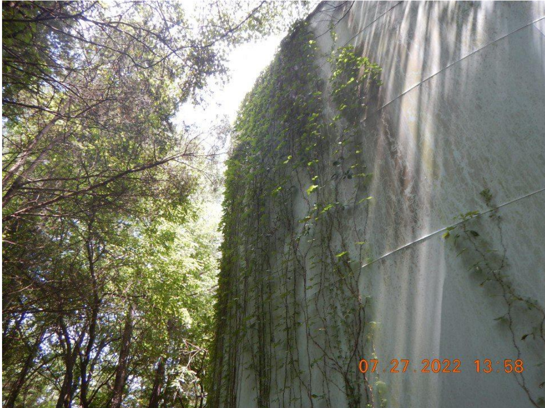
Photograph 87. Vegetation growing up and overhanging the Huguenot Road Tank.
