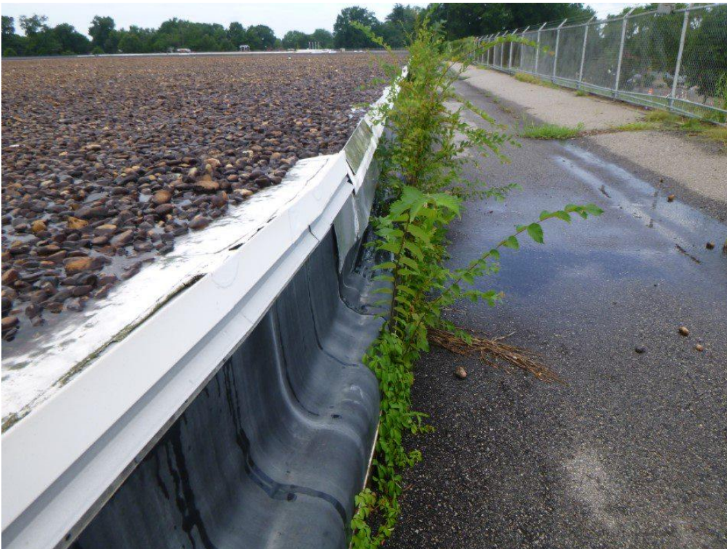
Photograph 62. Plant growth at base of Byrd Park Reservoir.
