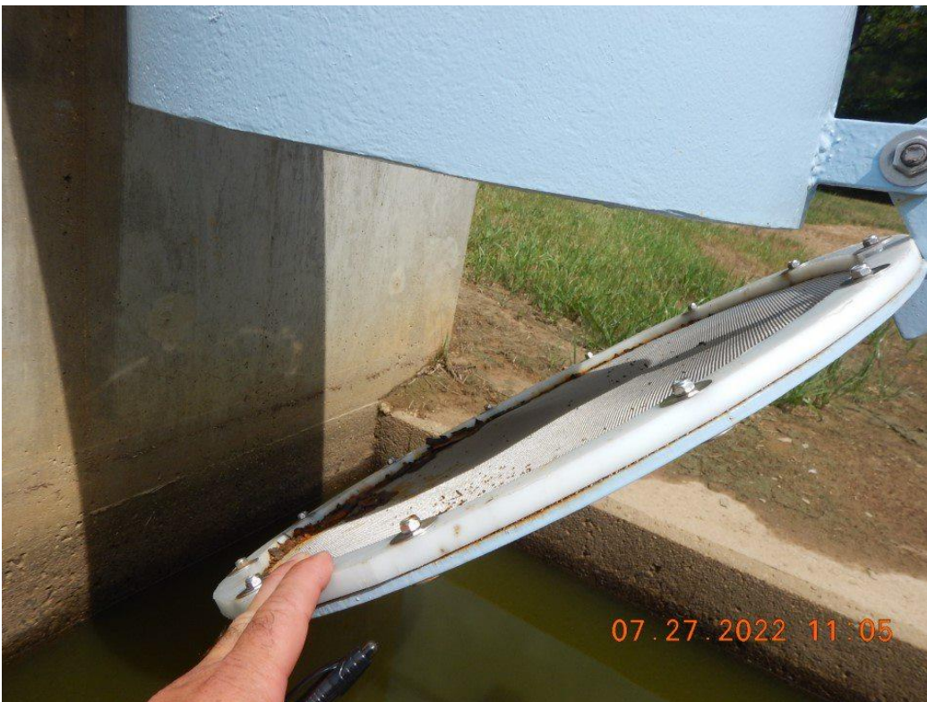
Photograph 70. Cofer Road Tank B overflow and debris inside screen.
