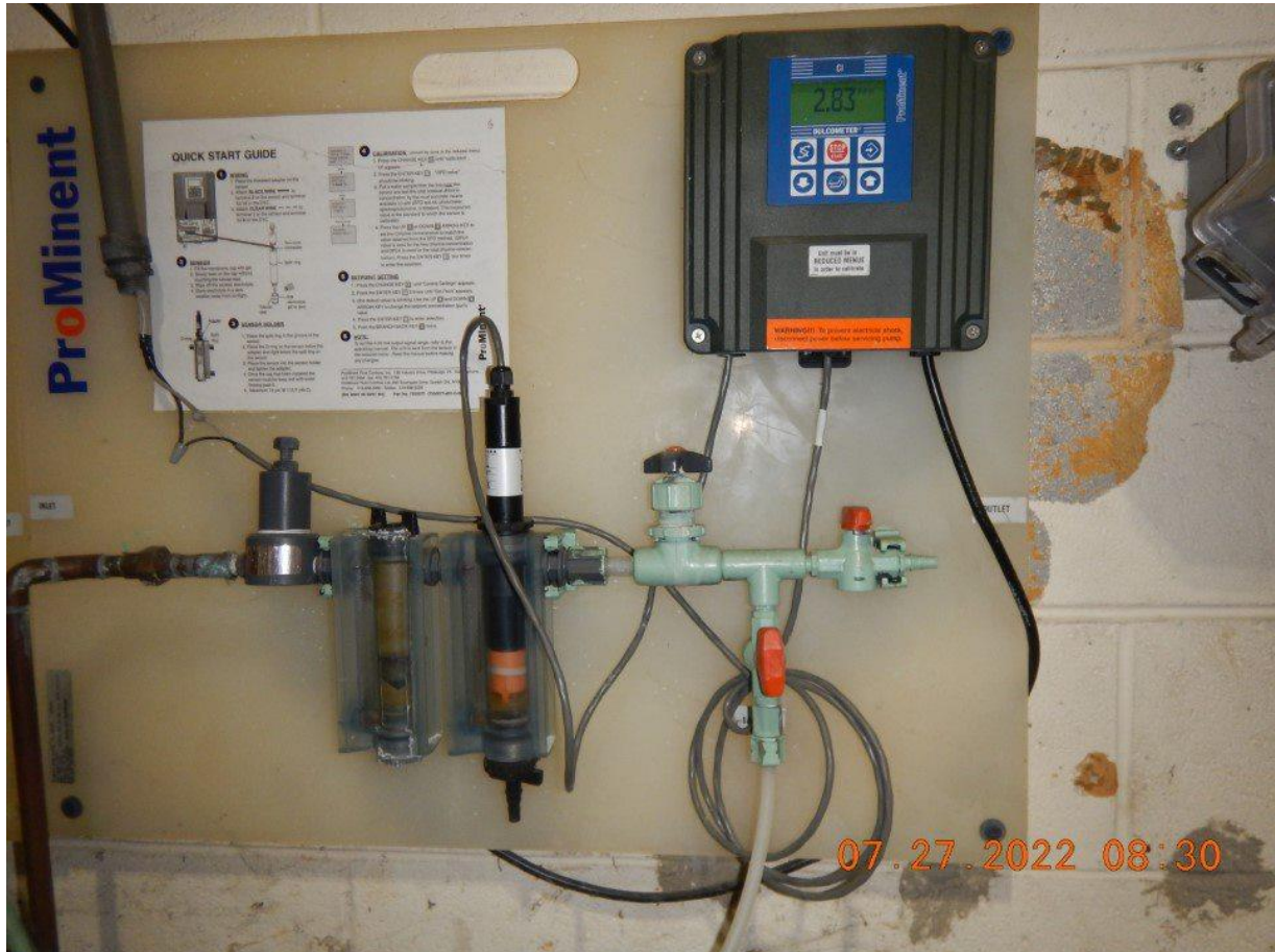
Photograph 42. Korah 2 and 3 Pump Station – ‘south’ chlorine analyzer.
