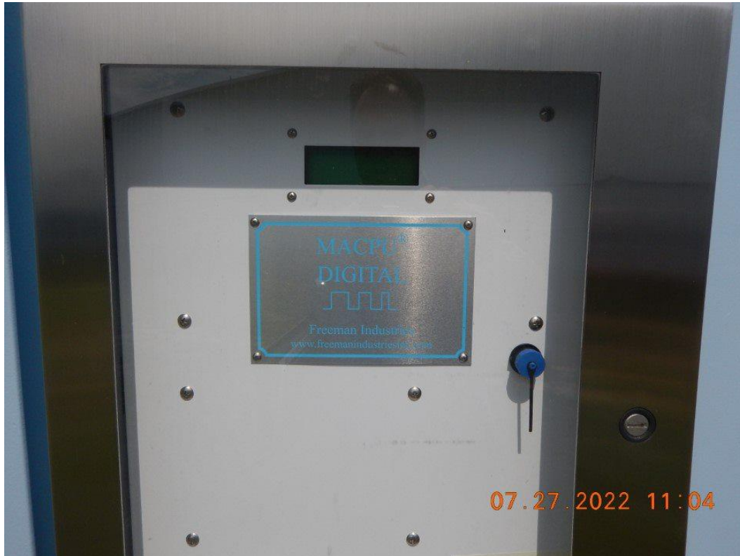
Photograph 71. MACPU unit, not in service at Cofer Road Tank A.
