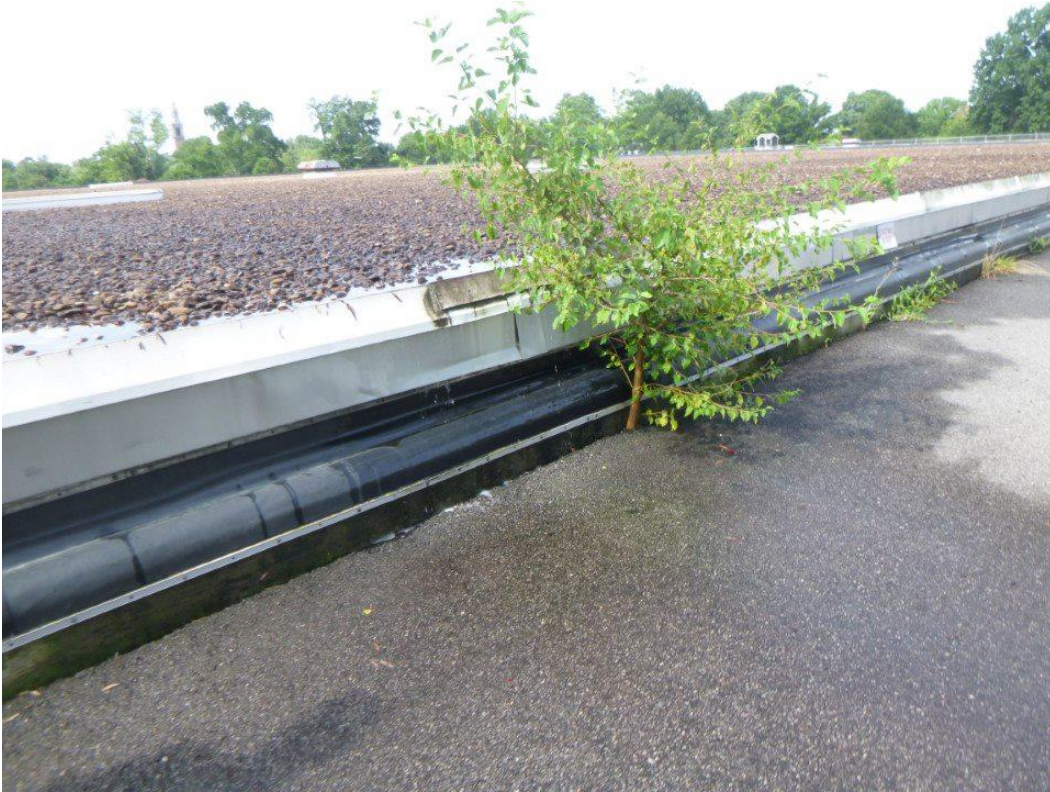
Photograph 61. Plant growth at base of Byrd Park Reservoir.
