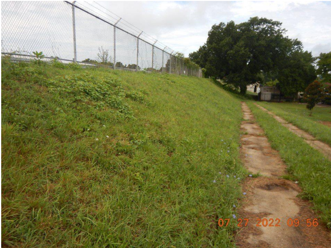
Photograph 51. Fencing and vegetation growth at the Byrd Park Reservoir.
