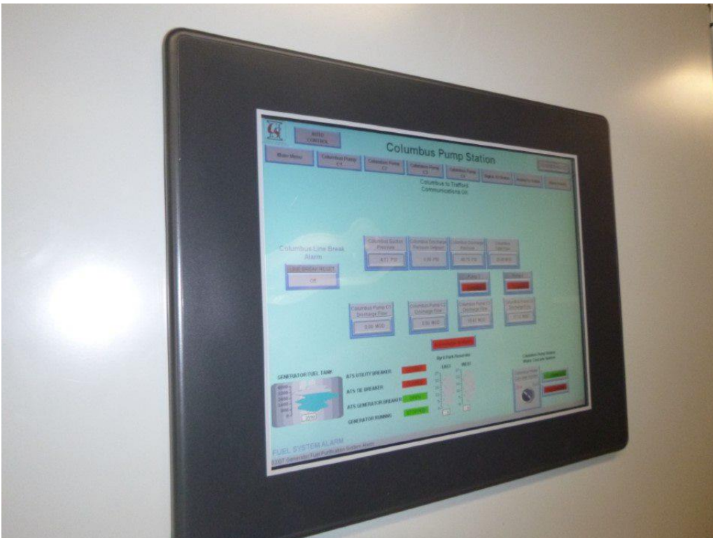
Photograph 94. PLC in electrical room at Columbus Pump Station.
