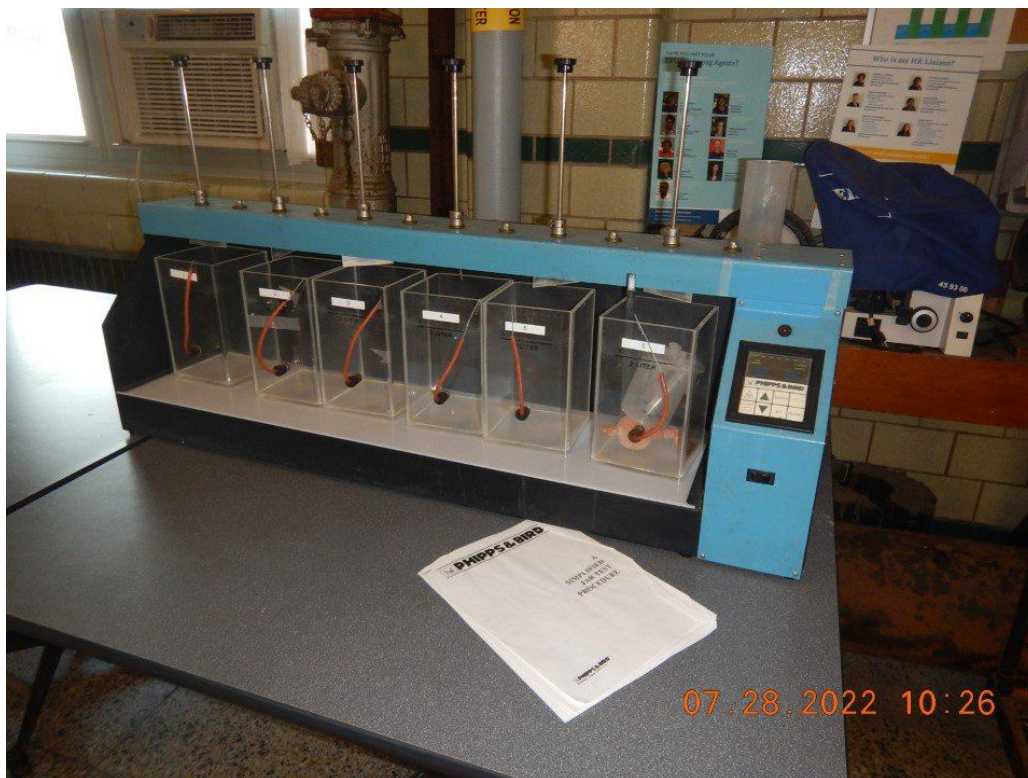
Photograph 128. Jar test apparatus outside of SCADA control room and process laboratory of Plant 2.
