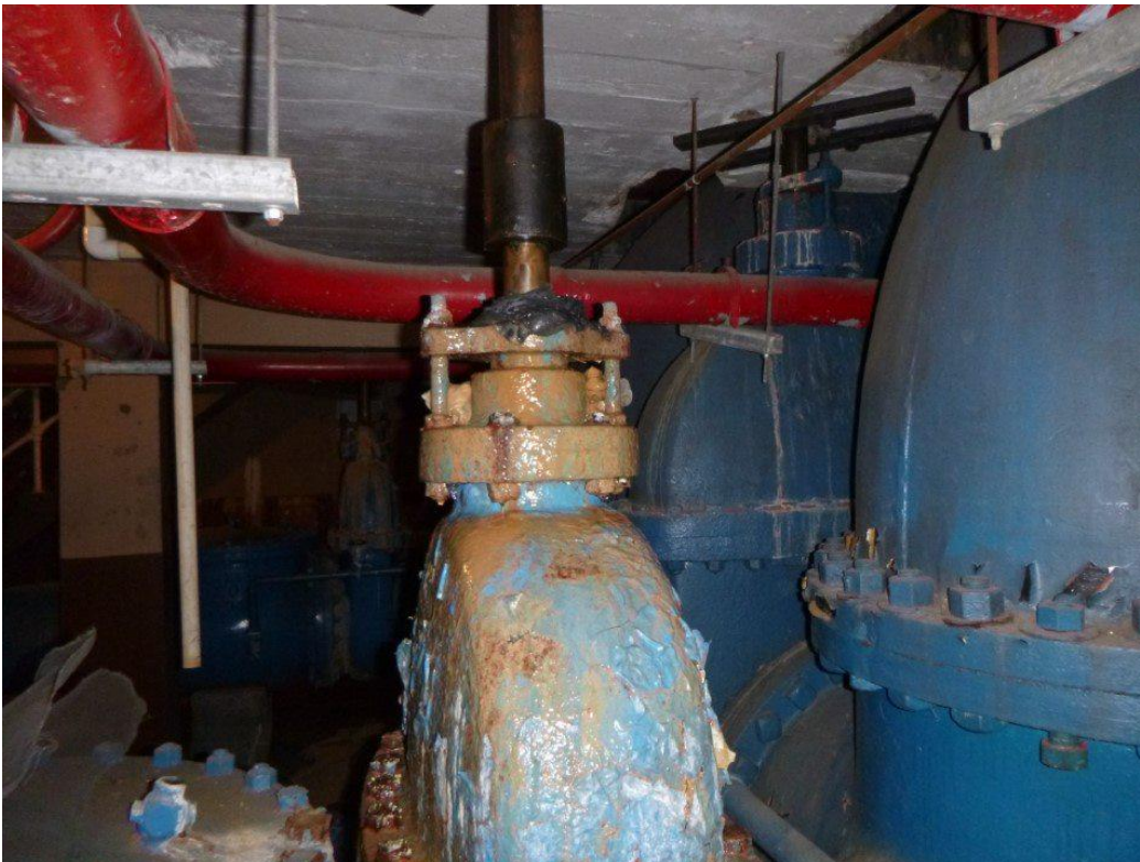
Photograph 100. Leaking seals on gate valves at Byrd Park Main Pump Station.
