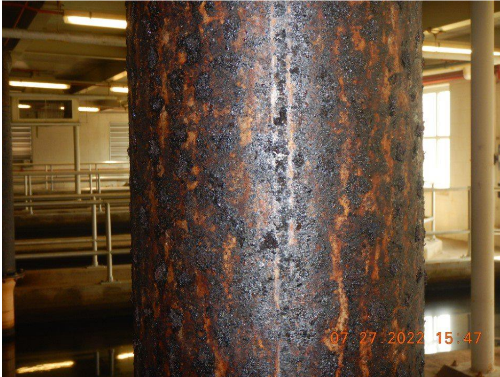
Photograph 113. Corrosion on air scour pipes located inside the enclosed Plant 1 filter room.
