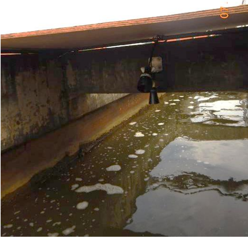
Photograph 16. Plant 2 flow meter above raw water coagulation channel, below piece of wood.
