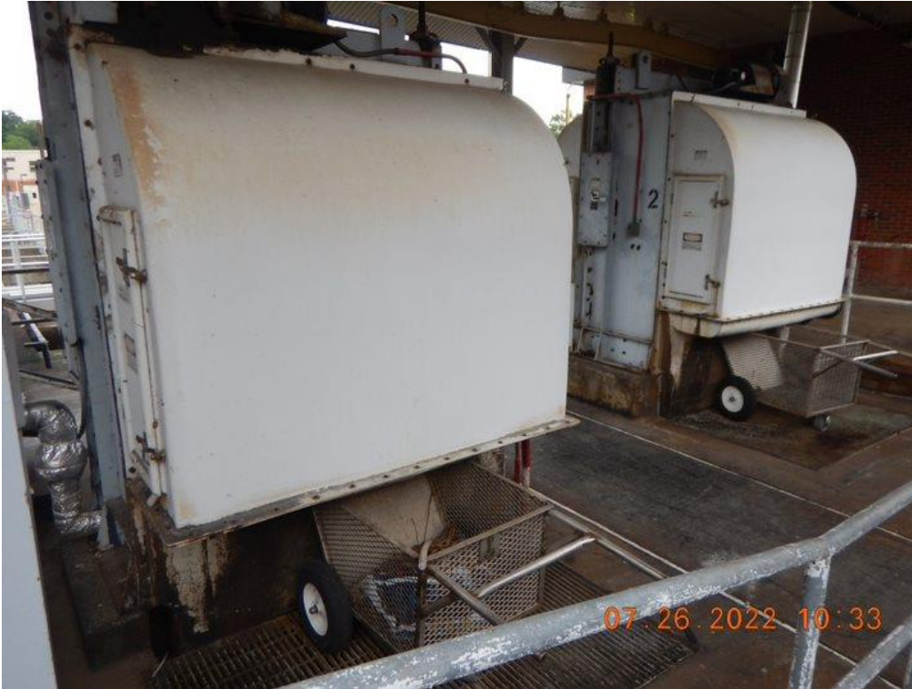
Photograph 12. Traveling screens at raw water intake.
