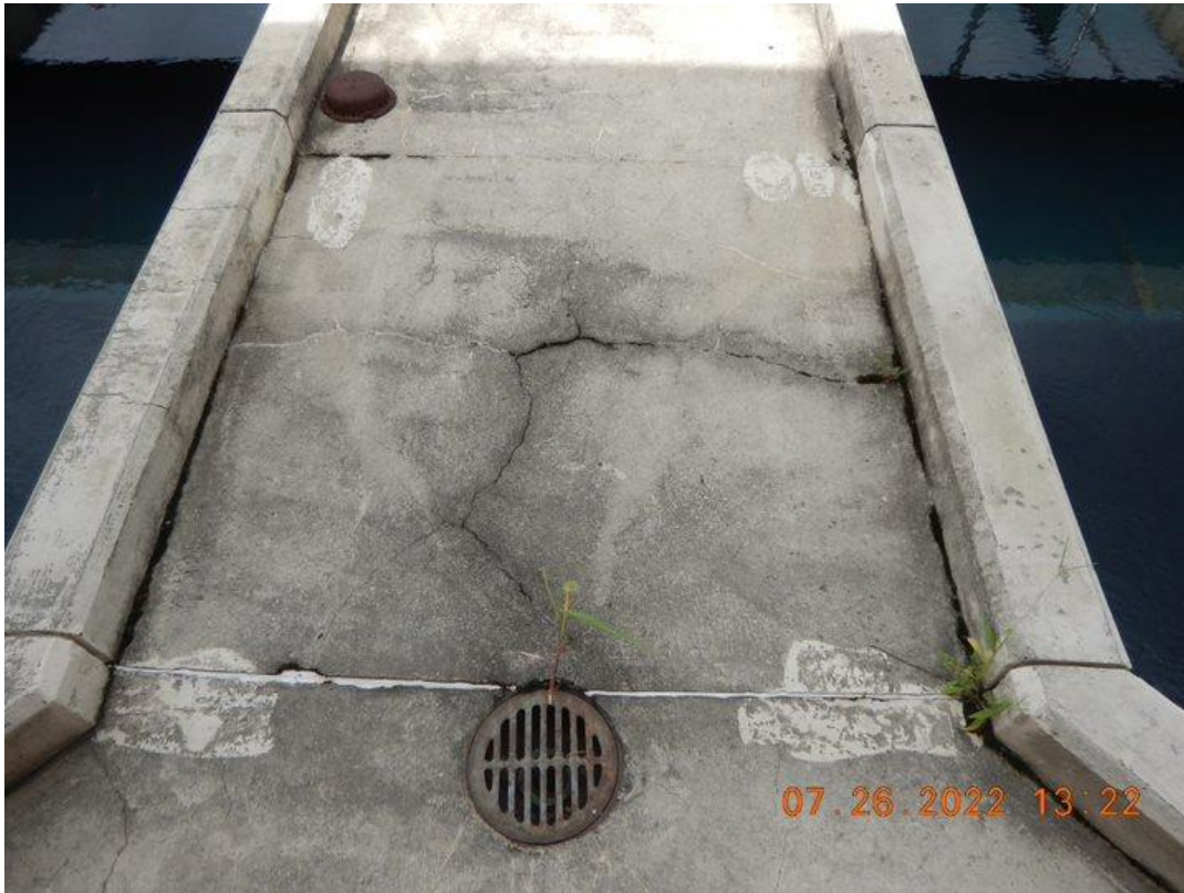
Photograph 26. Cracks in concrete above Plant 2 filter beds.
