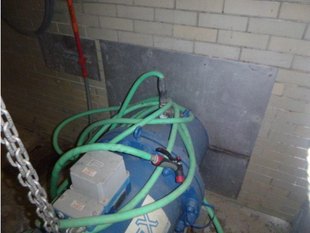
Photograph 109. Hose connected to threaded tap without vacuum breaker at Westhampton Pump Station.
