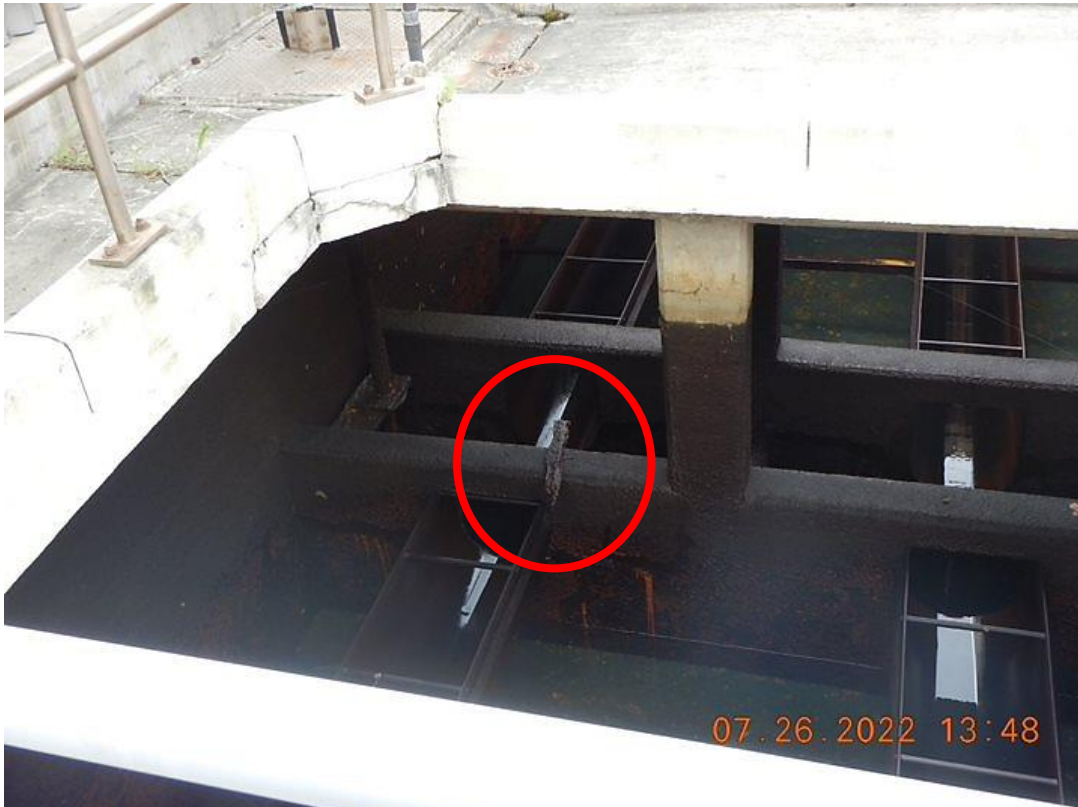
Photograph 30. Debris near influent/effluent channel of Filter 16.
