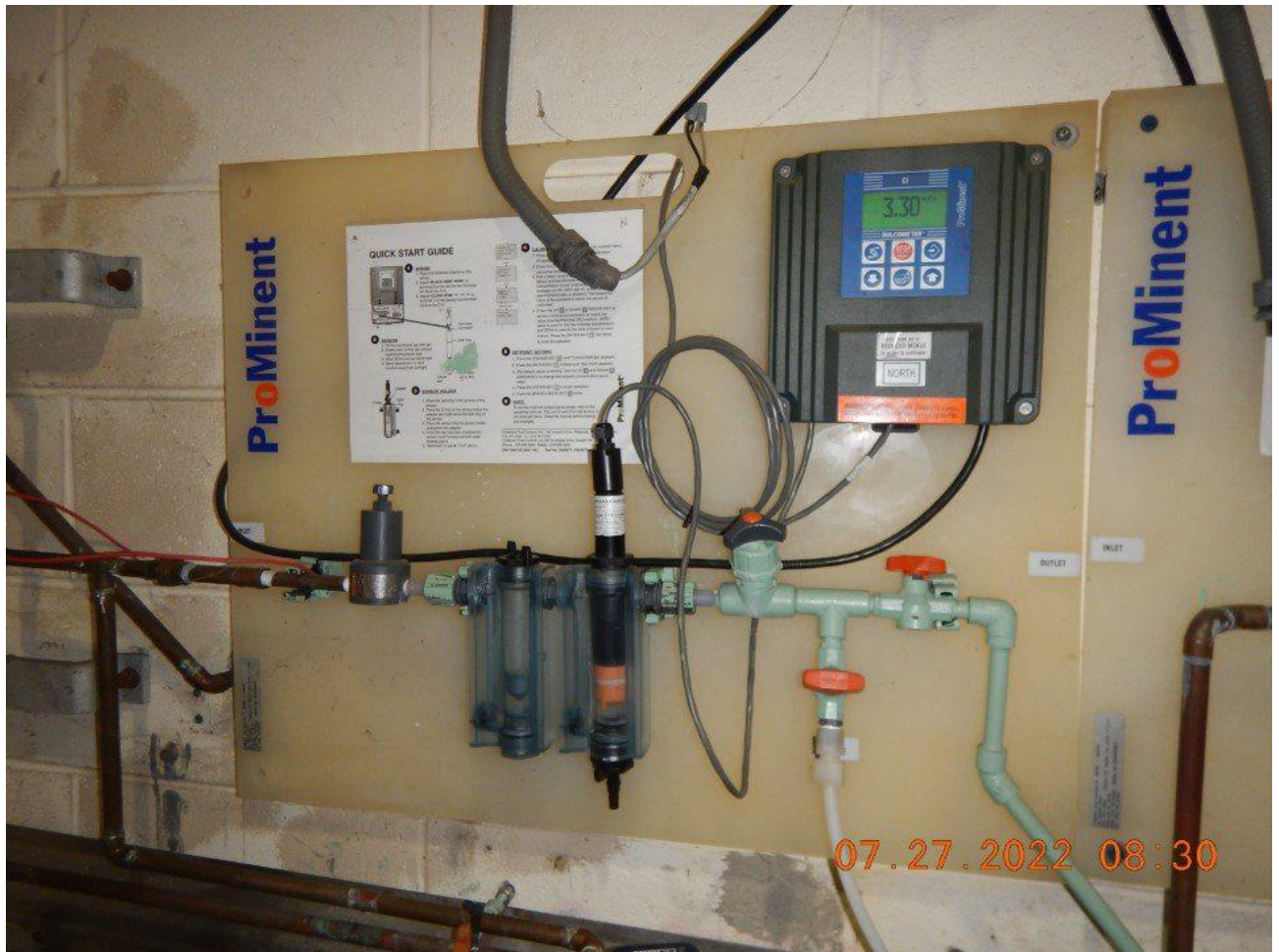
Photograph 41. Korah 2 and 3 Pump Station – ‘north’ chlorine analyzer.
