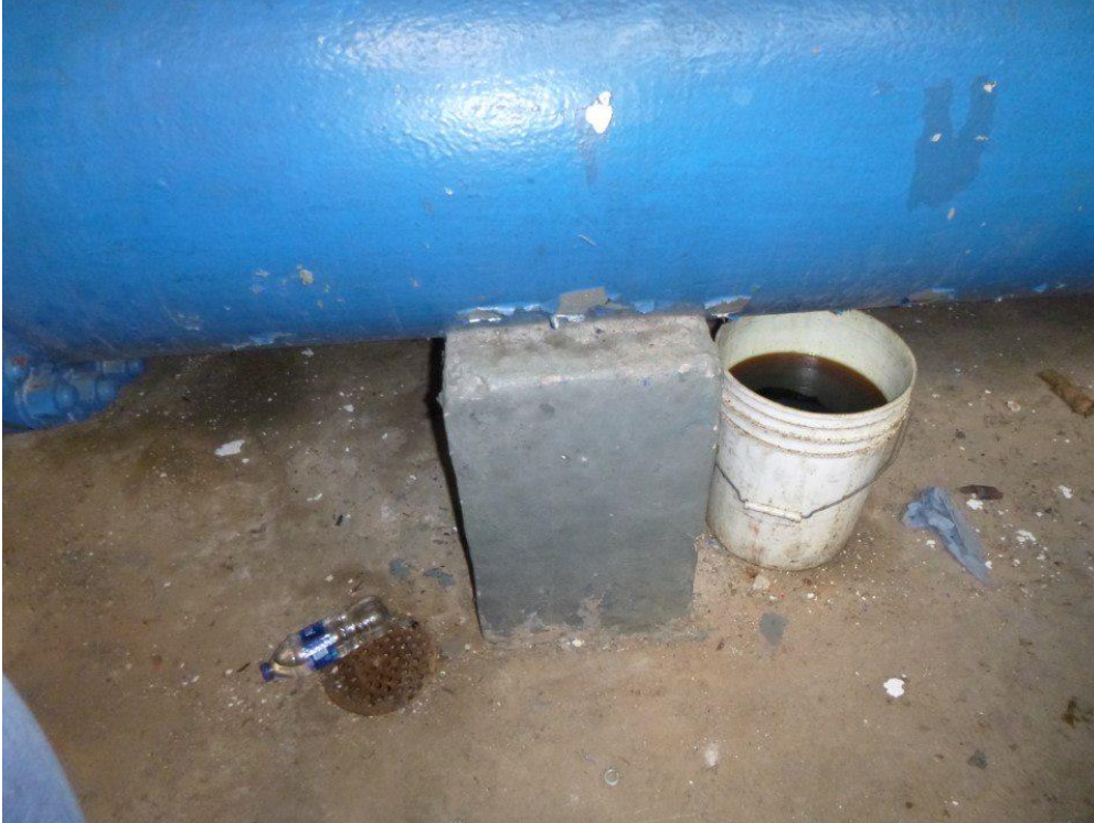
Photograph 103. Five-gallon bucket of oil/water mixture at Byrd Park Main Pump Station.
