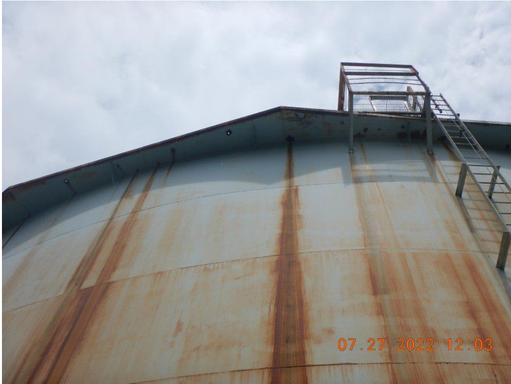
Photograph 77. Rust on exterior of Jahnke Road Tank.
