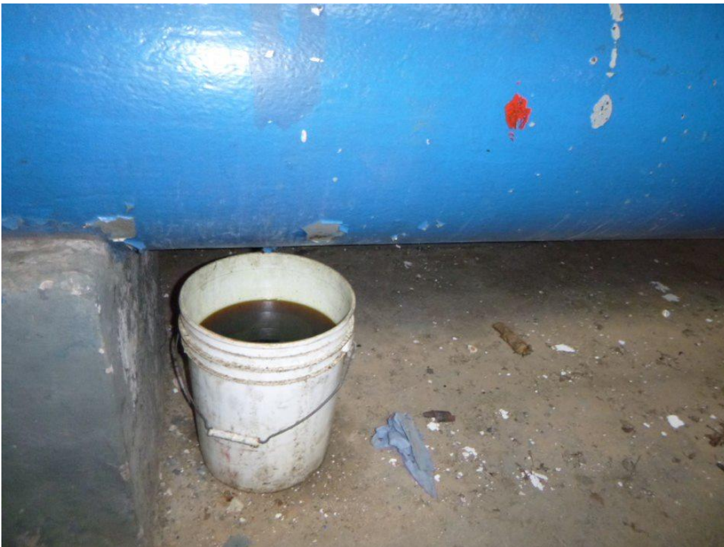
Photograph 98. Byrd Park Main Pump Station floor with debris and bucket of water/oil.
