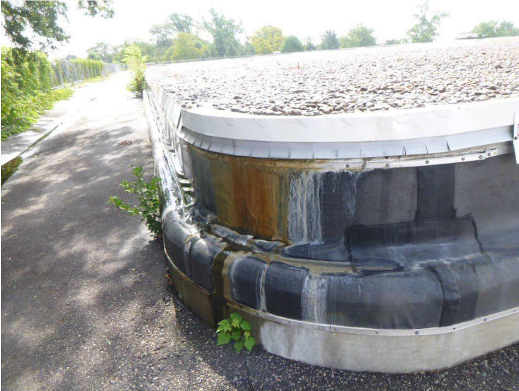
Photograph 59. Water leaking from siding on Byrd Park Reservoir roof.
