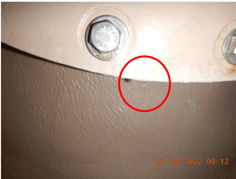
Photograph 119. Leak around gasket of sodium hypochlorite tank T-SH-1-3 at the West Chemical Building.
