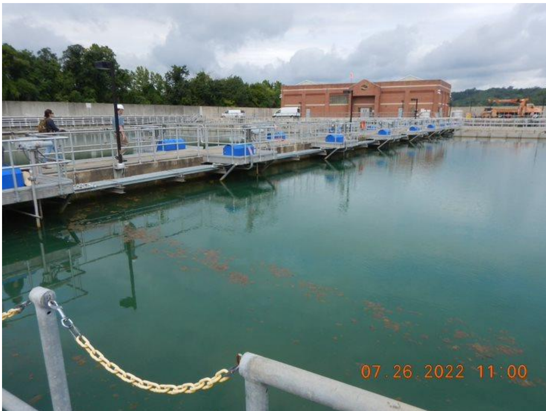
Photograph 19. Sedimentation basin of Plant 1 and solids residual collection system along middle walkway.
