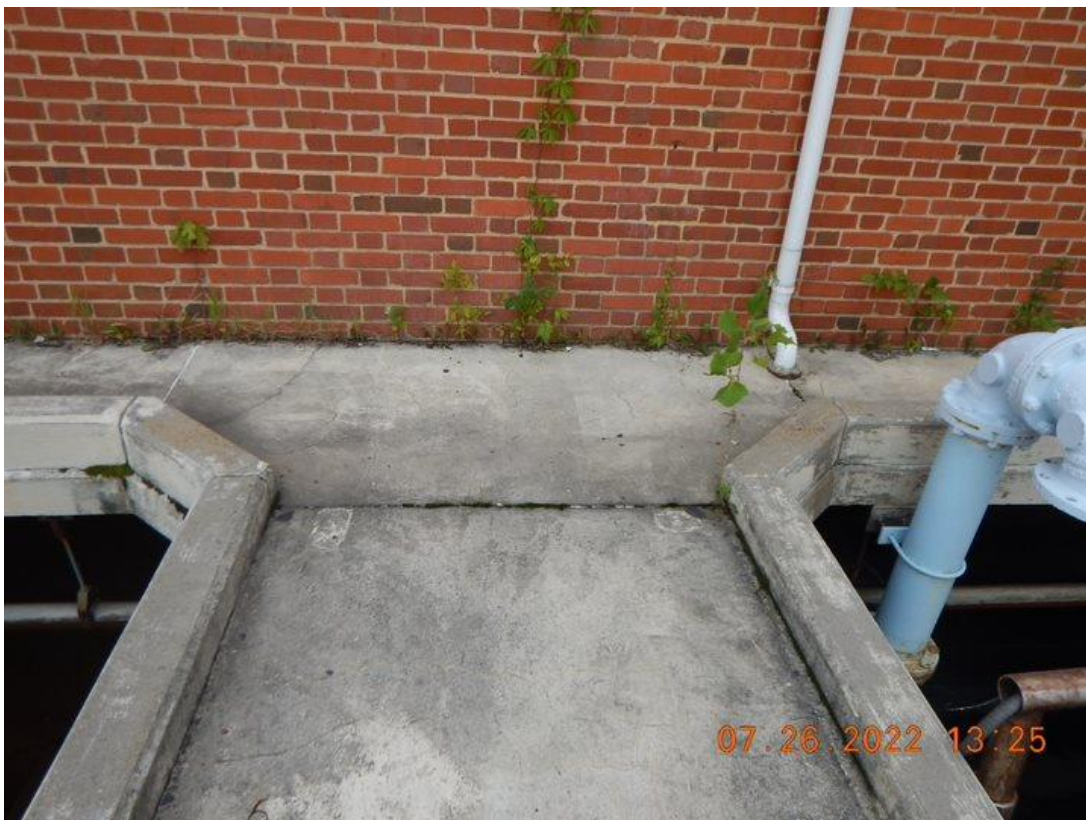
Photograph 27. Cracks in concrete above and vegetation growing around Plant 2 filters.
