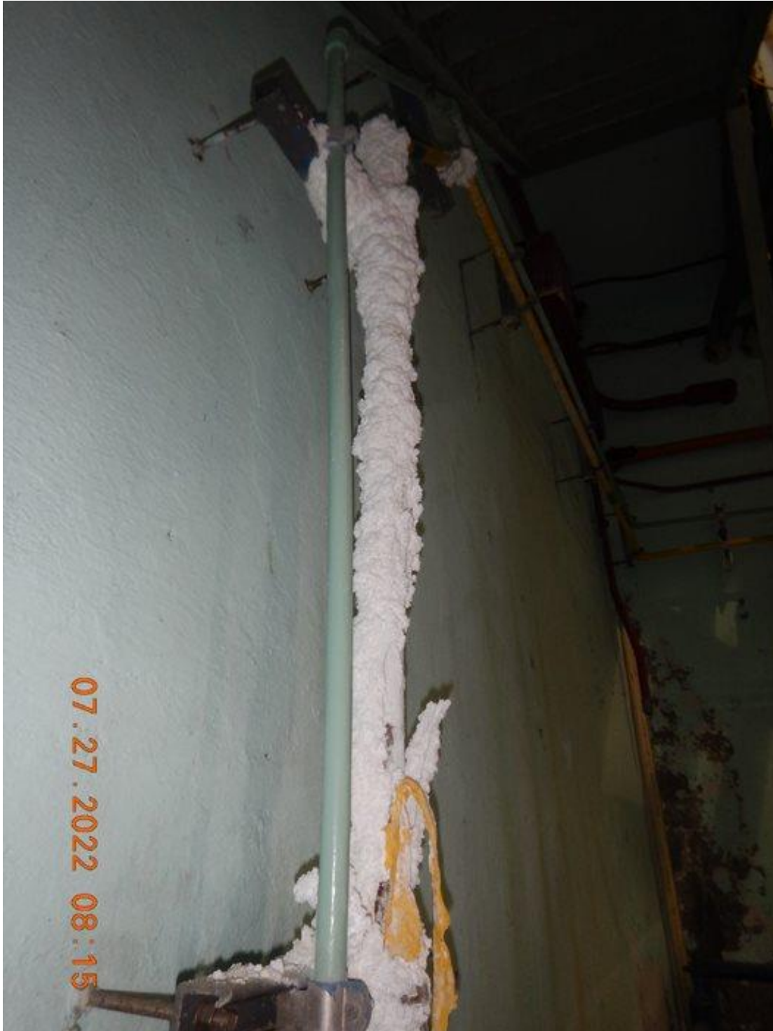
Photograph 35. Caustic soda line leak in Korah 1 Pump Station.
