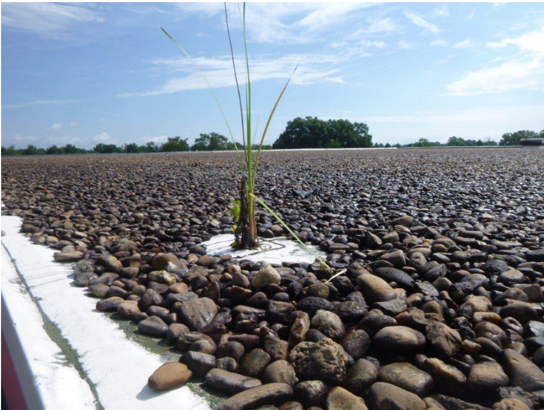
Photograph 56. Vegetation growth on the roof of Byrd Park Reservoir.
