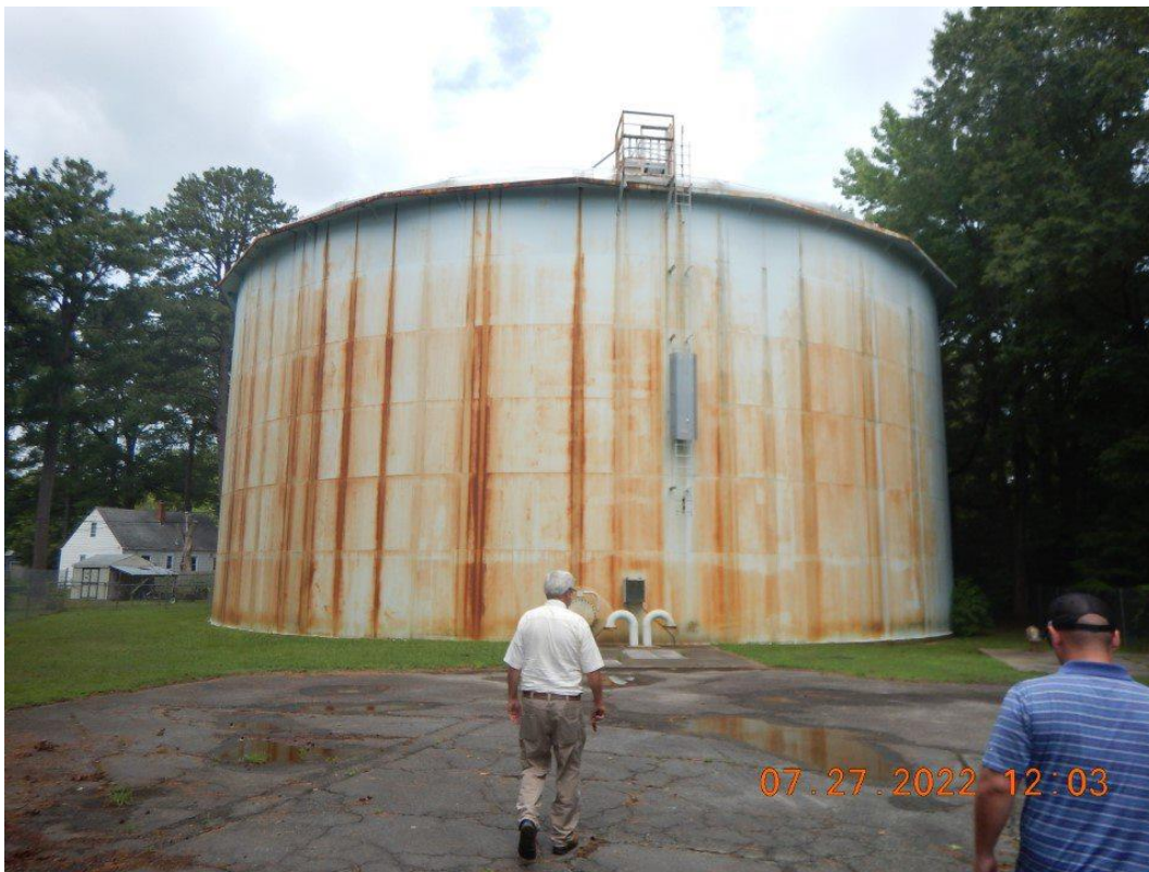
Photograph 76. Rust on exterior of Jahnke Road Tank.
