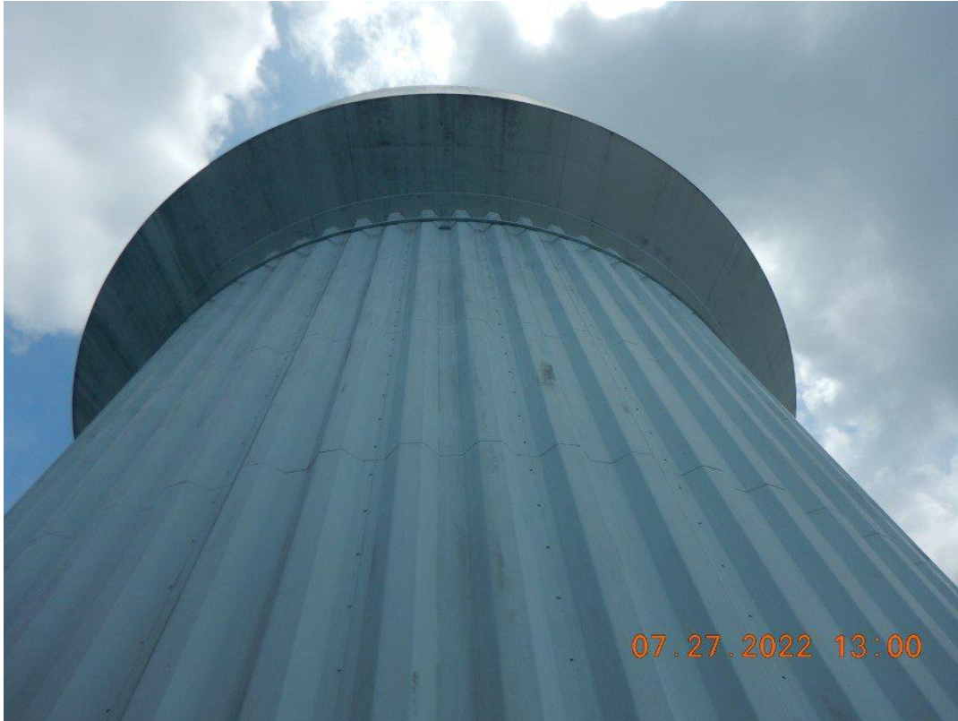
Photograph 81. Base of Warwick Road Tank with algal growth on bottom.
