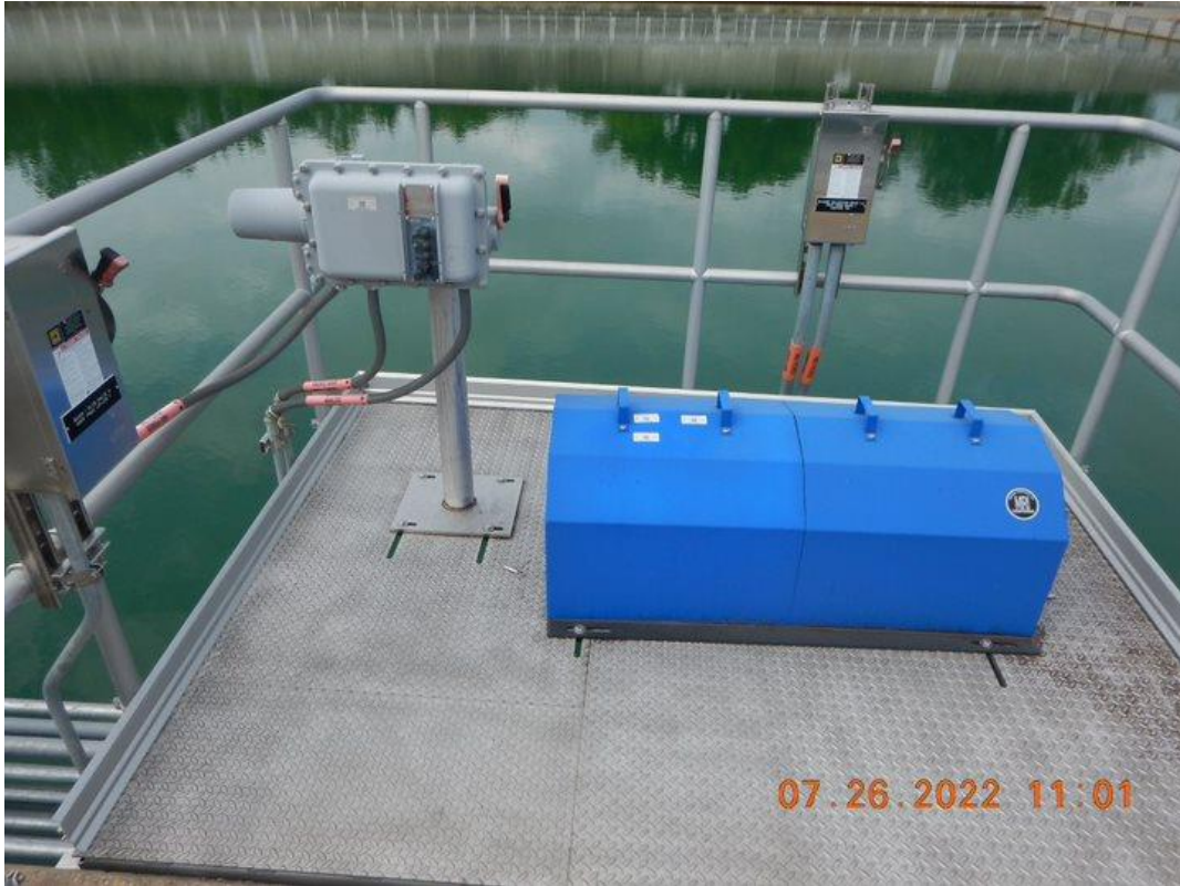
Photograph 20. Solids residual collection system cables and controls.
