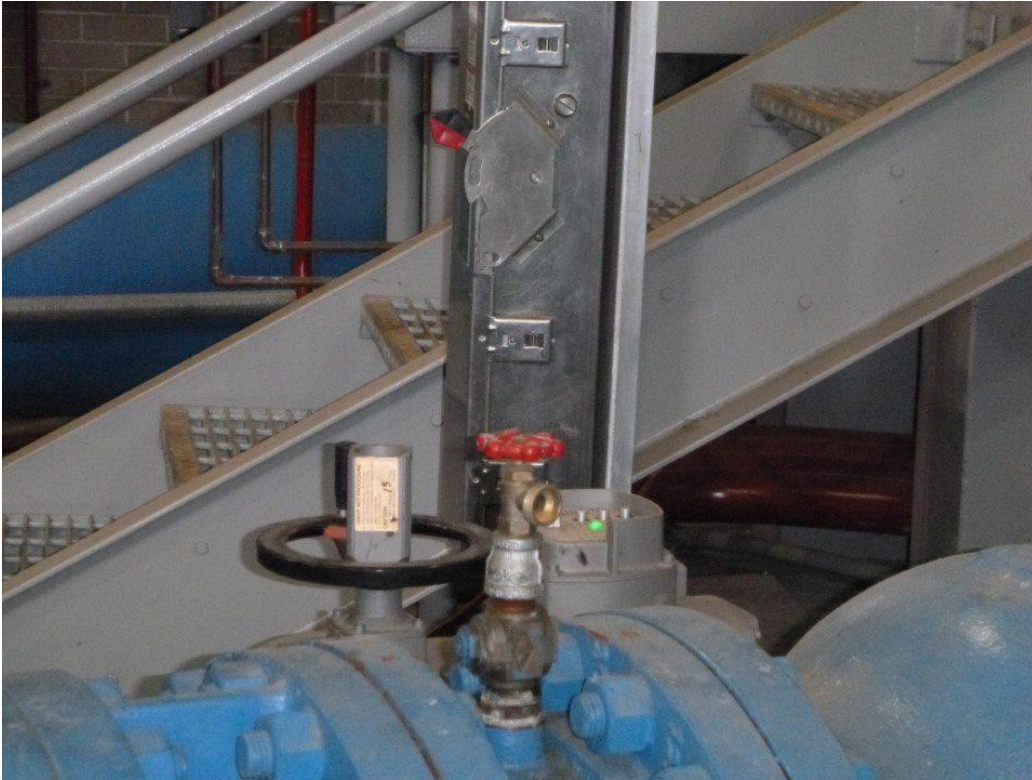
Photograph 93. Threaded tap on finished water line without backflow prevention at the Columbus Pump Station.
