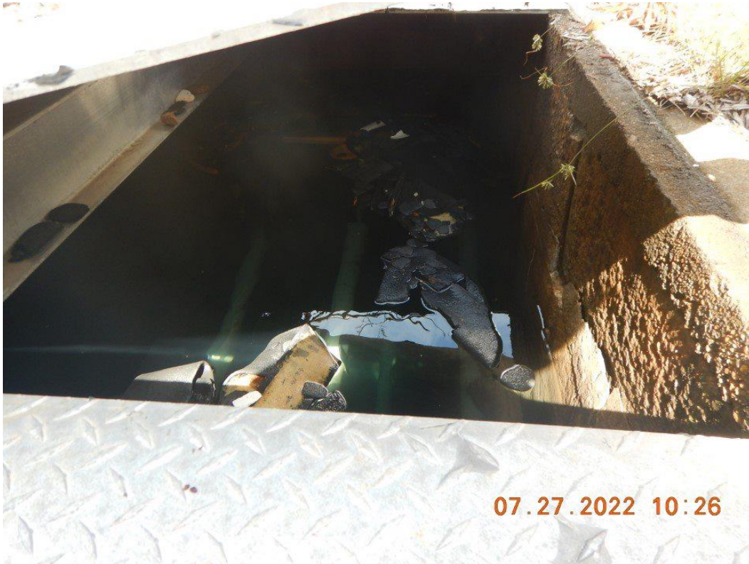
Photograph 67. Access vault filled with water in northern walkway of Byrd Park Reservoir.
