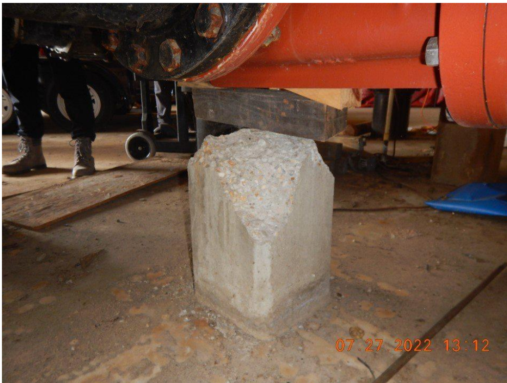
Photograph 82. Pieces of wood stacked to attempt to provide support to the transmission pipe at Warwick Road Tank.
