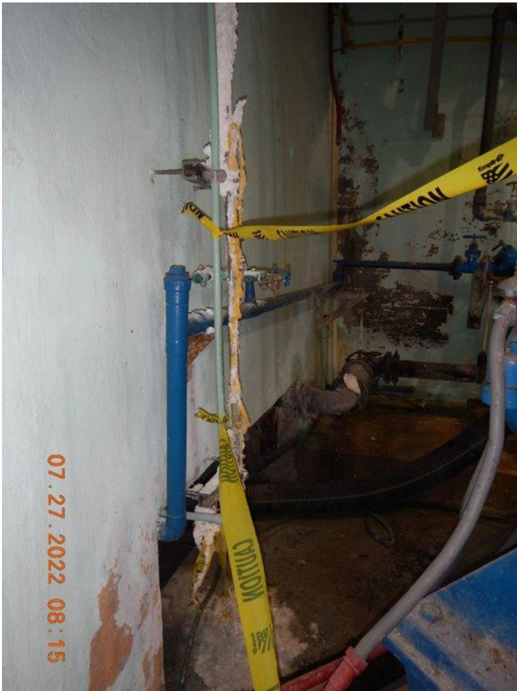
Photograph 34. Caustic soda line leak and caution tape in Korah 1 Pump Station.
