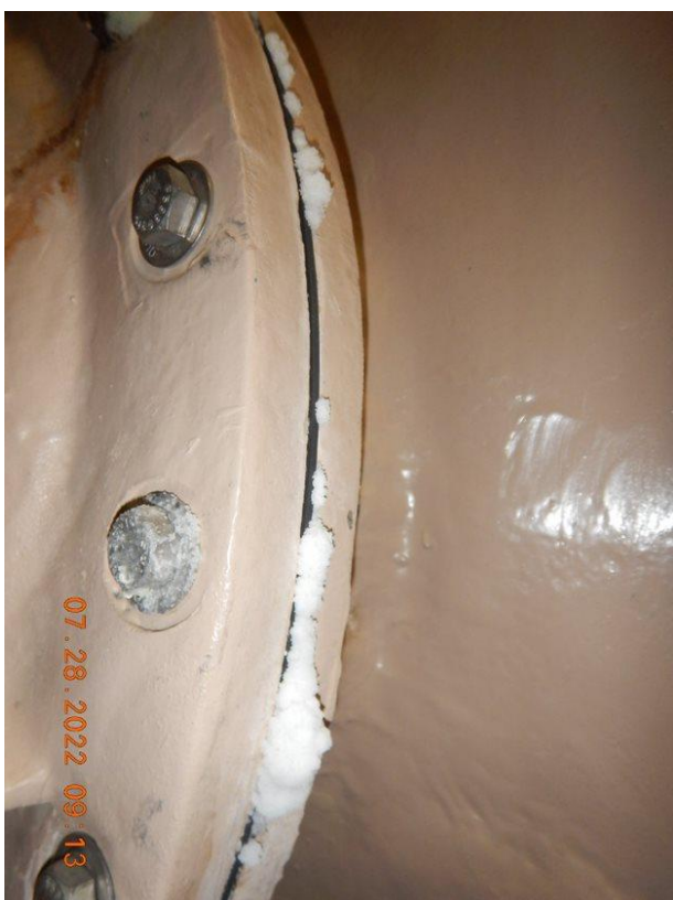
Photograph 120. Crystallized sodium hypochlorite around gasket at tank T-SH-1-3 at the West Chemical Building.
