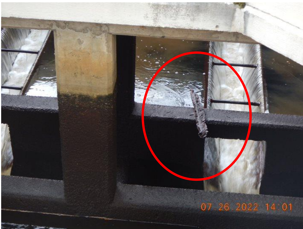
Photograph 31. Debris near influent/effluent channel of Filter 16.
