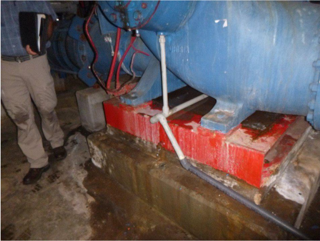
Photograph 47. K2-2 pump motor discharging water onto Korah 2 and 3 Pump Station floor.
