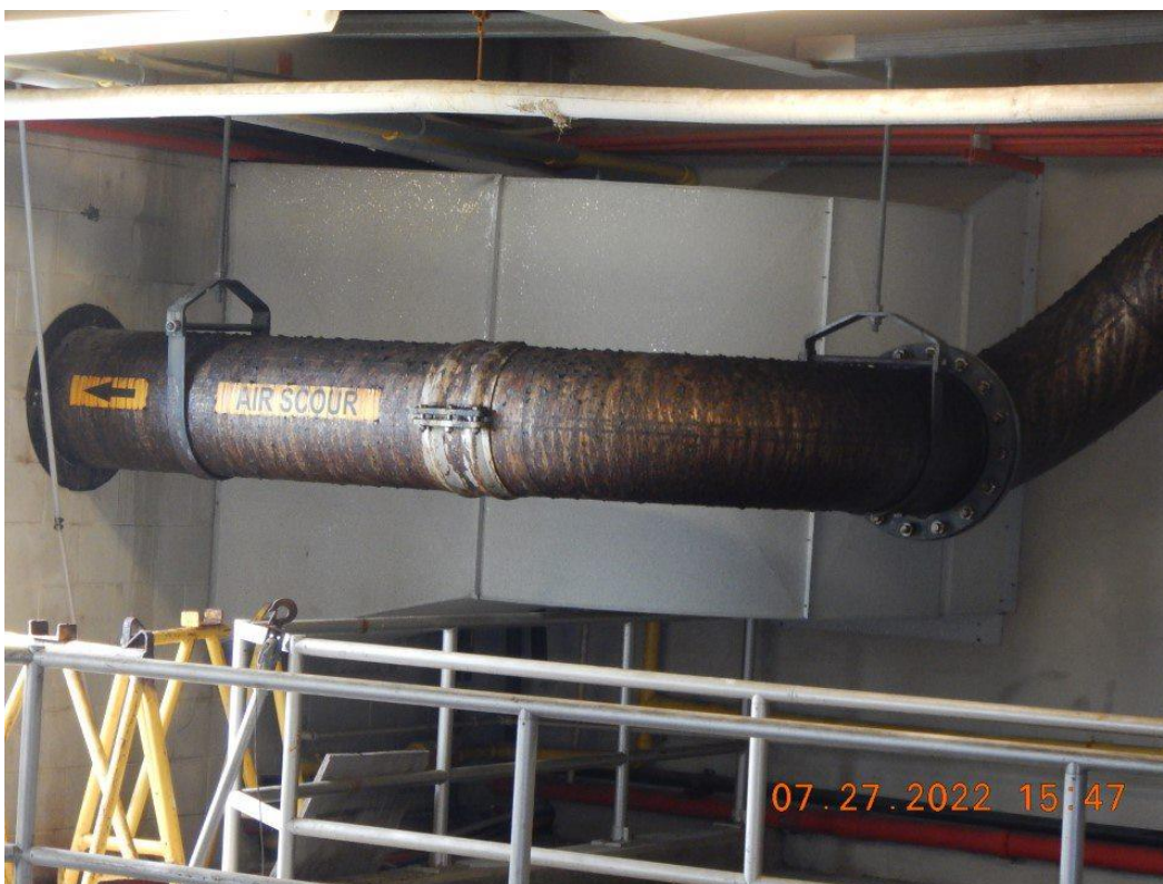
Photograph 112. Corrosion on air scour pipes located inside the enclosed Plant 1 filter room.
