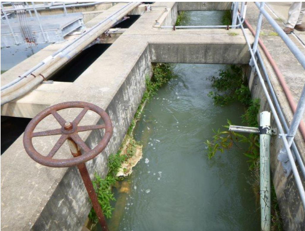
Photograph 13. Vegetation growing in concrete raw water channel at water line.
