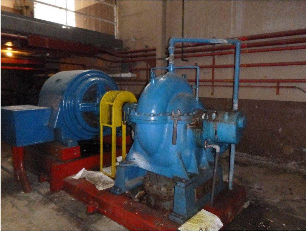
Photograph 101. Leaking lubrication at pump at Byrd Park Main Pump Station.
