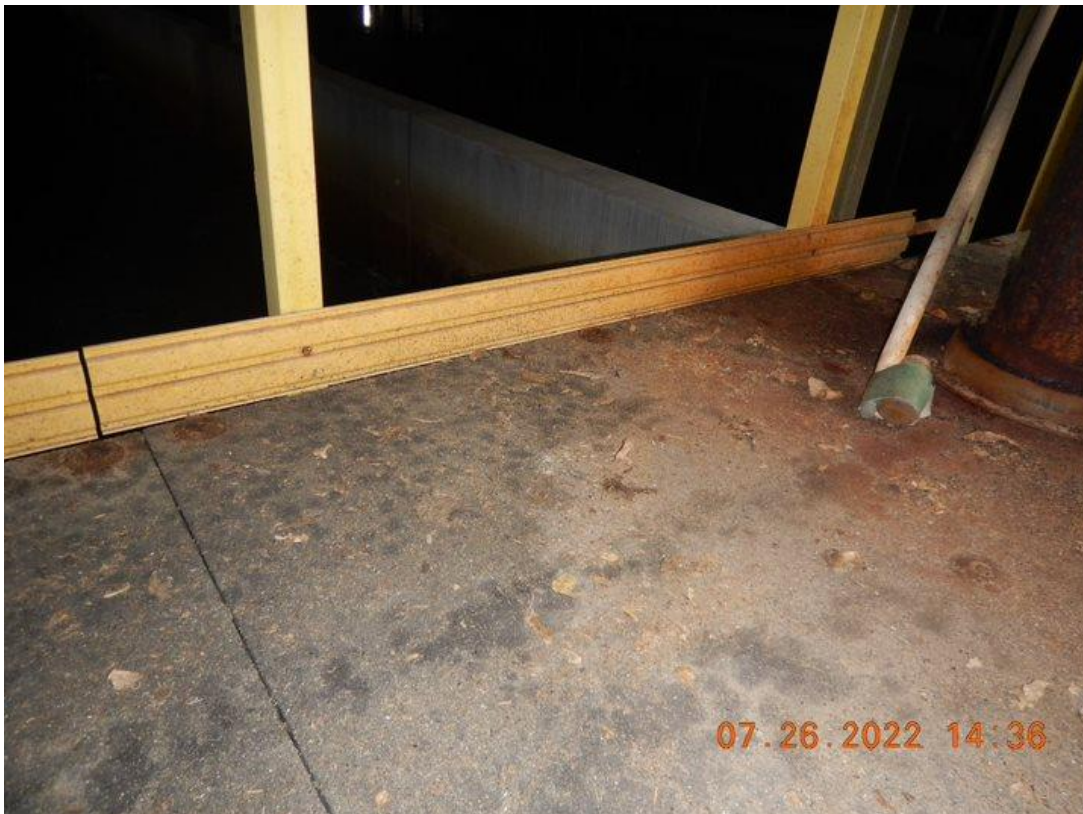
Photograph 33. Dirt and debris on landing area above Plant 2 finished water basin.
