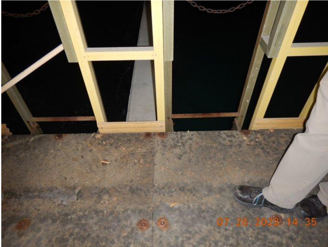
Photograph 32. Landing area at entry of Plant 2 finished water basin; no baseboards to prevent debris from falling into water.
