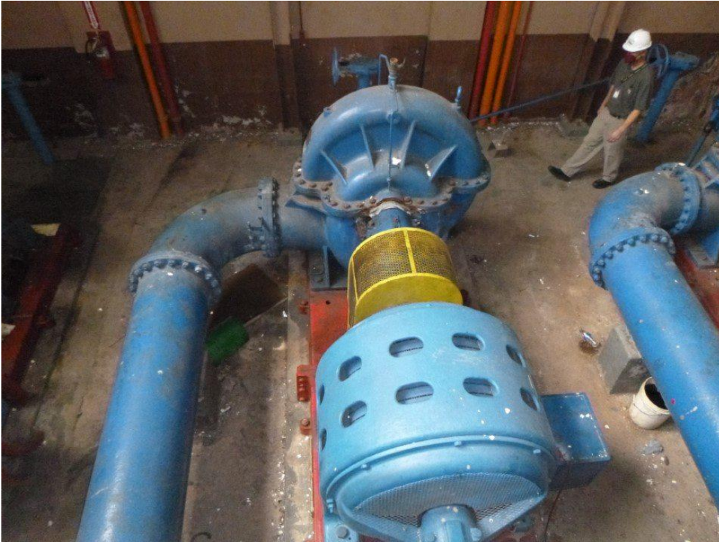
Photograph 97. Byrd Park Main Pump Station floor with debris.
