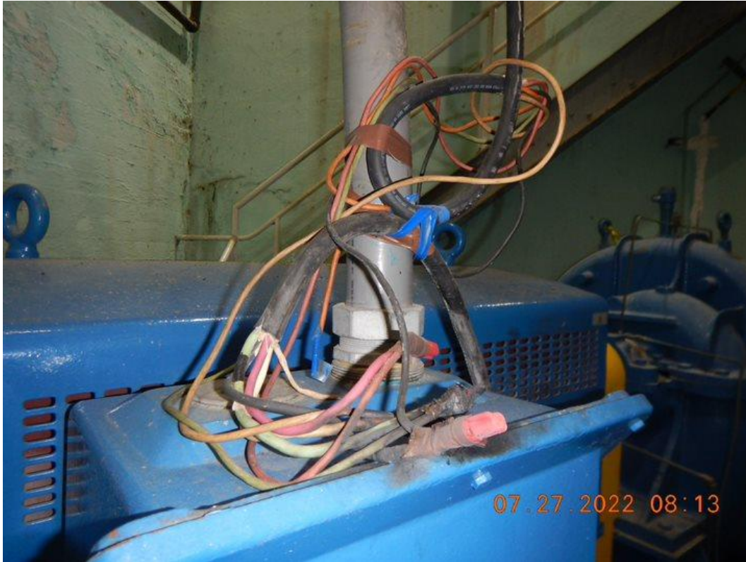
Photograph 38. Exposed wiring on K1-2 pump at Korah 1 Pump Station.
