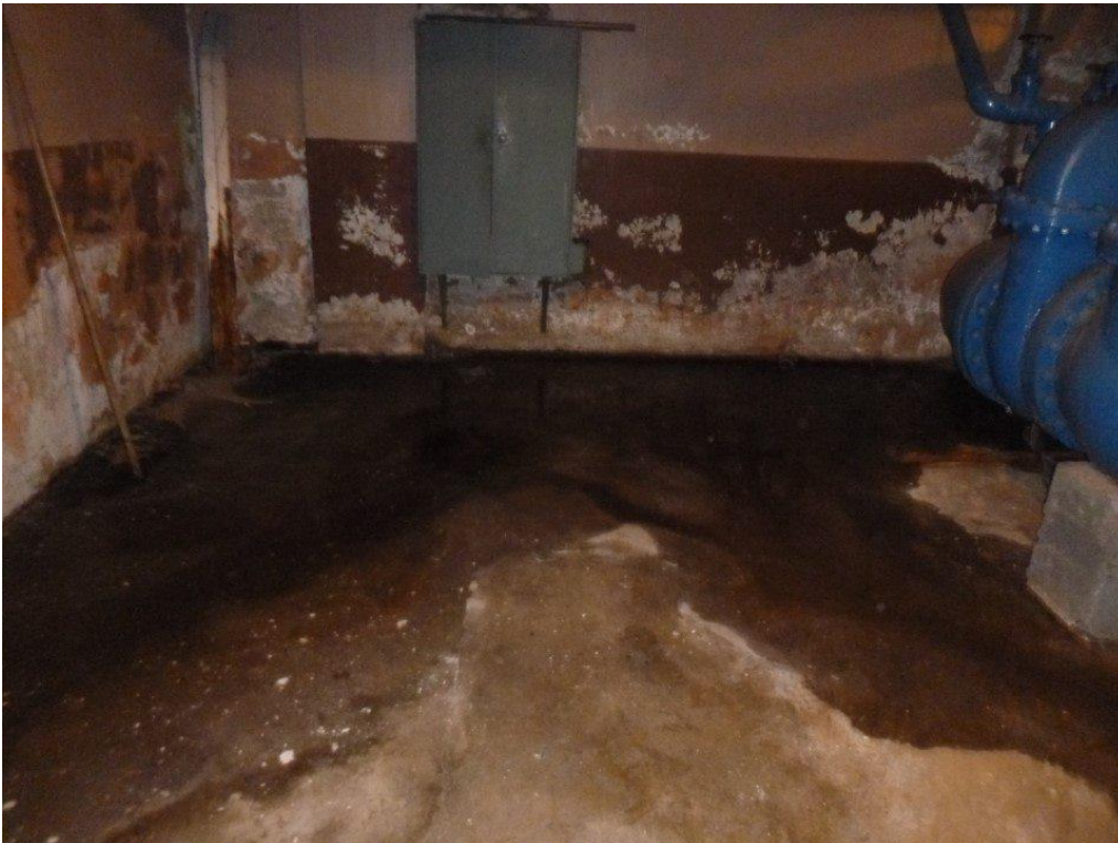
Photograph 102. Standing water on floor at Byrd Park Main Pump Station.
