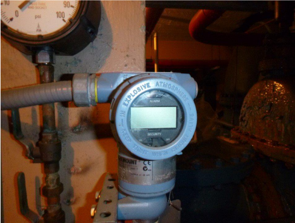
Photograph 107. Non-operational meter at Byrd Park Main Pump Station.
