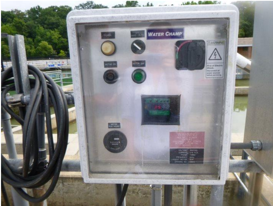
Photograph 18. Water Champ flash mixer controls at Plant 1.
