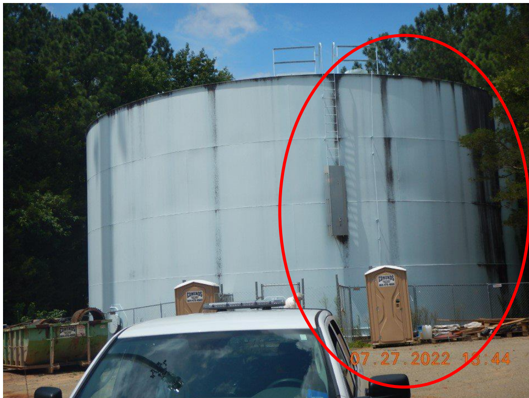
Photograph 86. Huguenot Road Tank with temporary fencing and staining.
