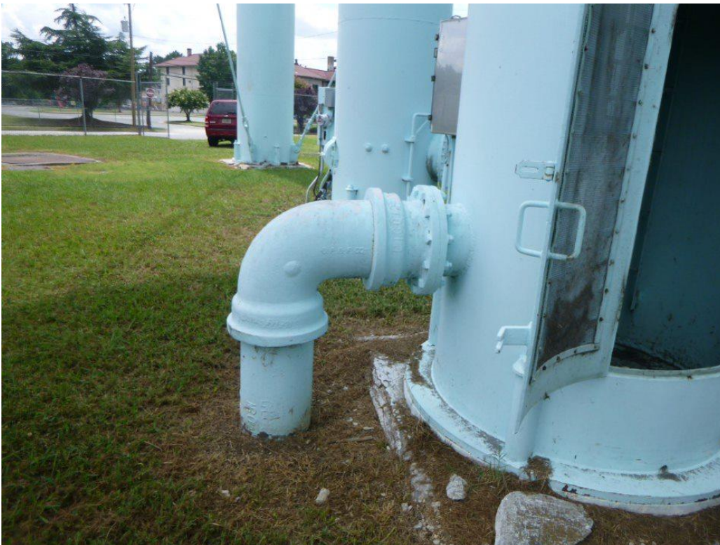
Photograph 110. Potential overflow pipe for Ginter Park Tank.
