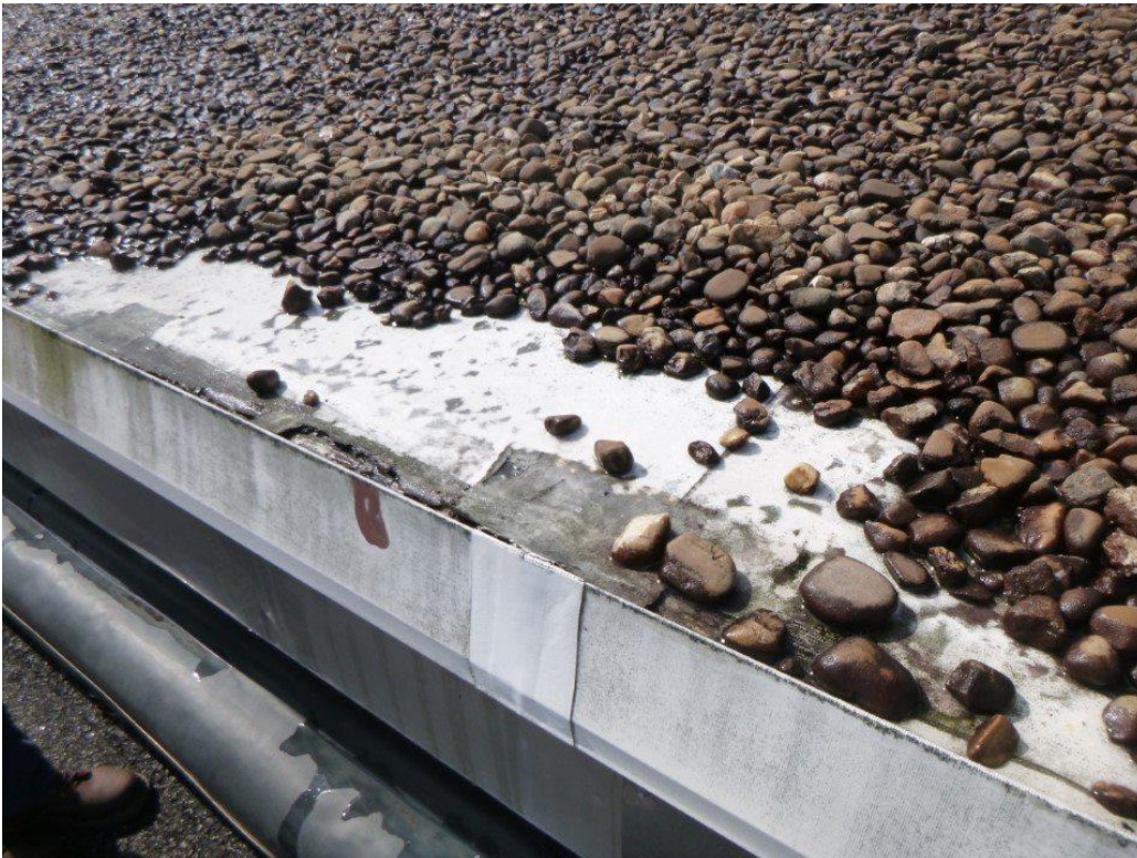
Photograph 60. Damage and water leaking from roof and siding on Byrd Park Reservoir.
