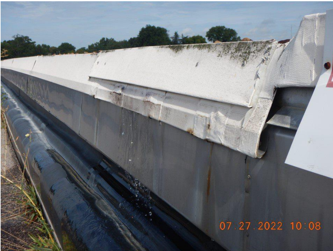
Photograph 58. Water leaking from siding on Byrd Park Reservoir roof.
