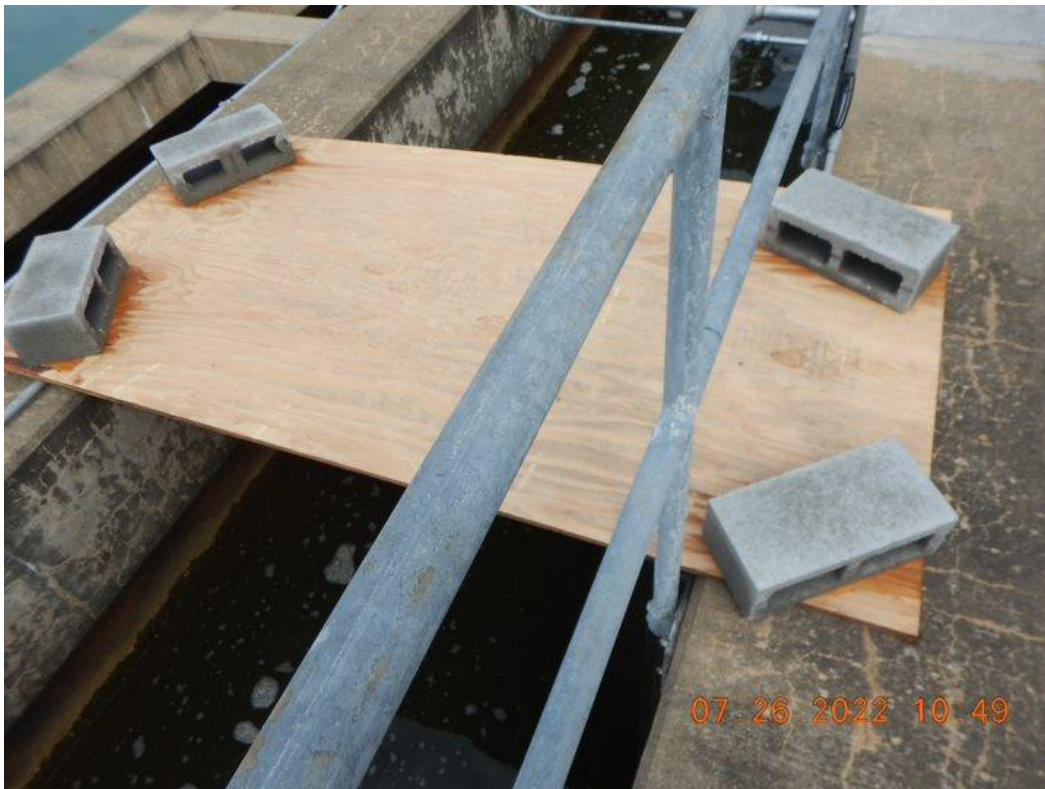
Photograph 15. Plant 2 flow meter above raw water coagulation channel, wood to block potential sun interference.
