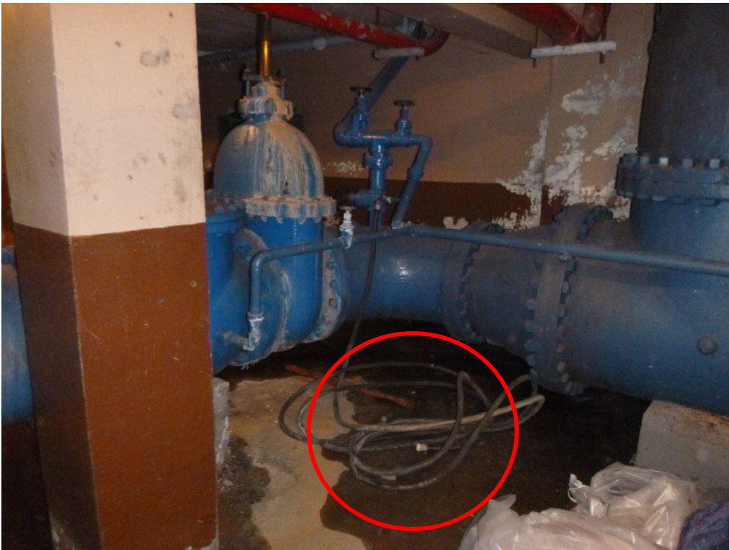
Photograph 104. Hose on ground in standing water attached to finished water line without vacuum breaker at Byrd Park Main Pump Station.
