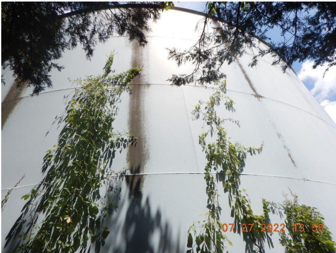
Photograph 88. Vegetation growing up and overhanging the Huguenot Road Tank.
