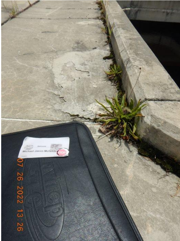
Photograph 28. Vegetation growing around concrete structures above Plant 2 filters.
