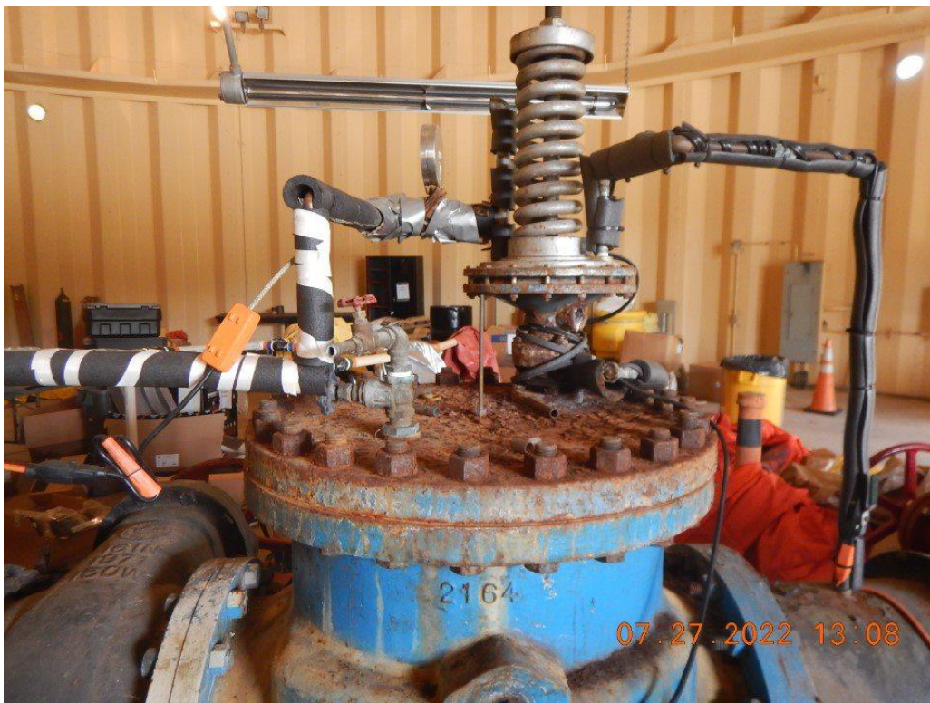
Photograph 84. Corrosion on the control valve on the transmission pipe of the Warwick Road Tank.
