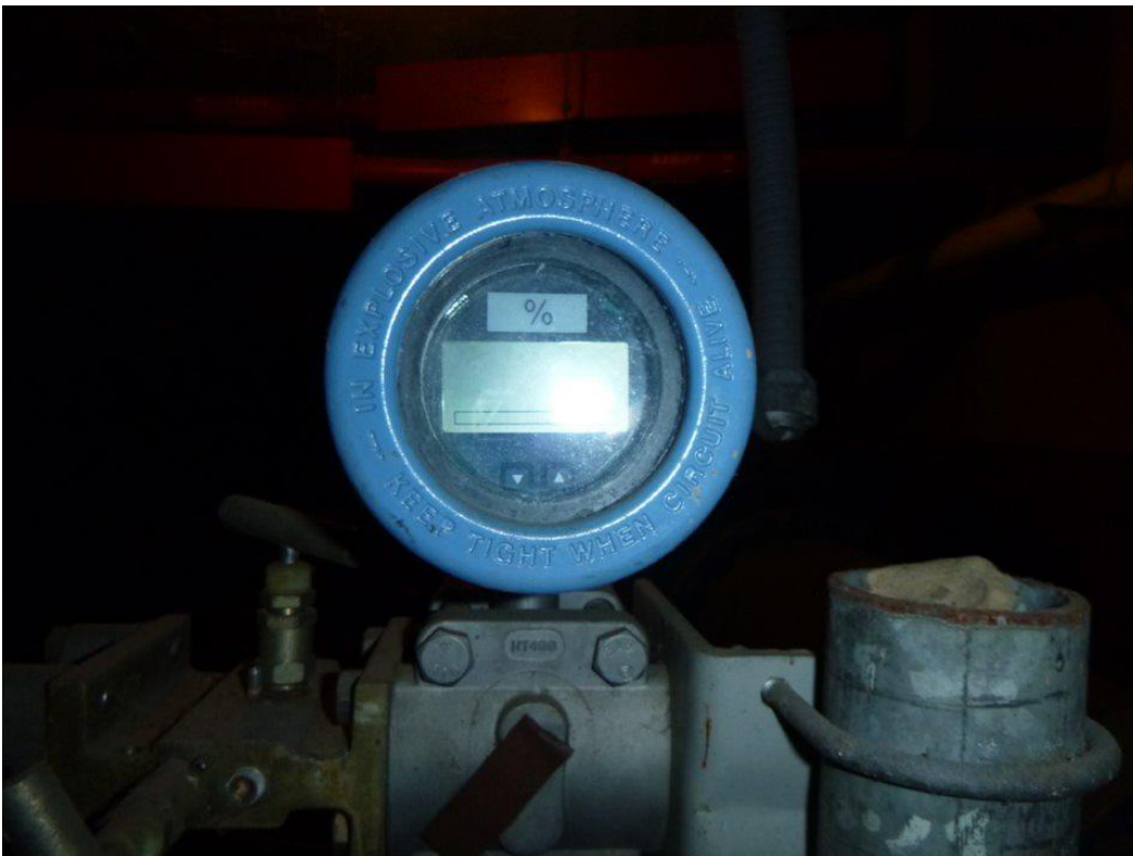
Photograph 106. Non-operational meter at Byrd Park Main Pump Station.
