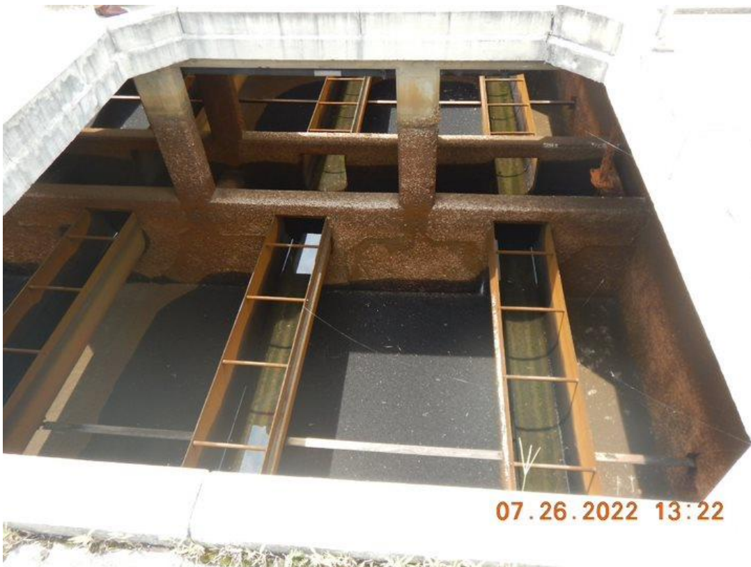
Photograph 25. Filter 19, not in service.
