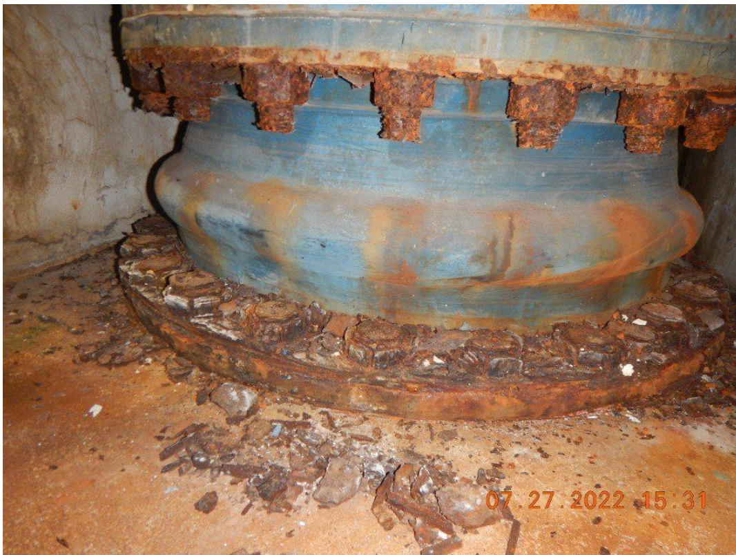
Photograph 114. Corrosion on pump 1 that takes water from the Plant 1 clearwell to the finished water basin.
