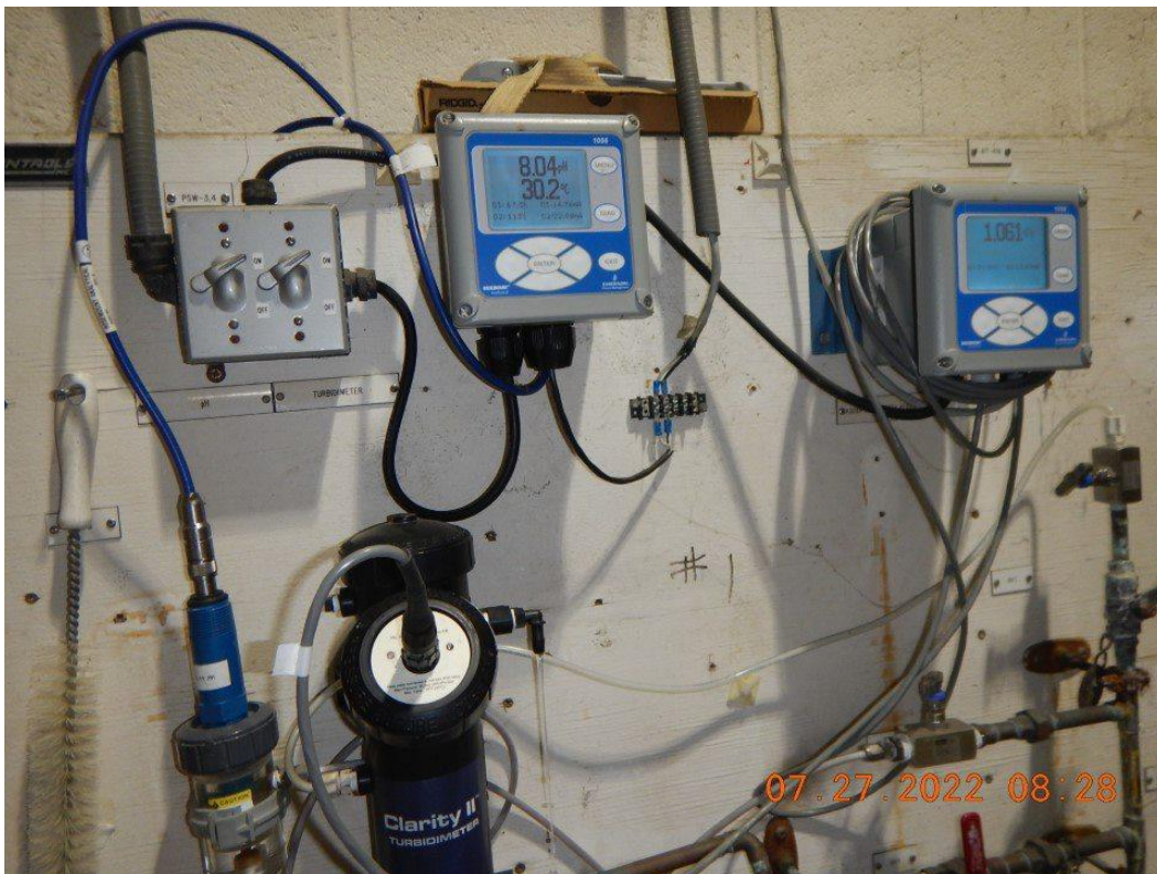
Photograph 39. Korah 2 and 3 Pump Station – ‘south’ analyzers for pH, temperature, and turbidity.
