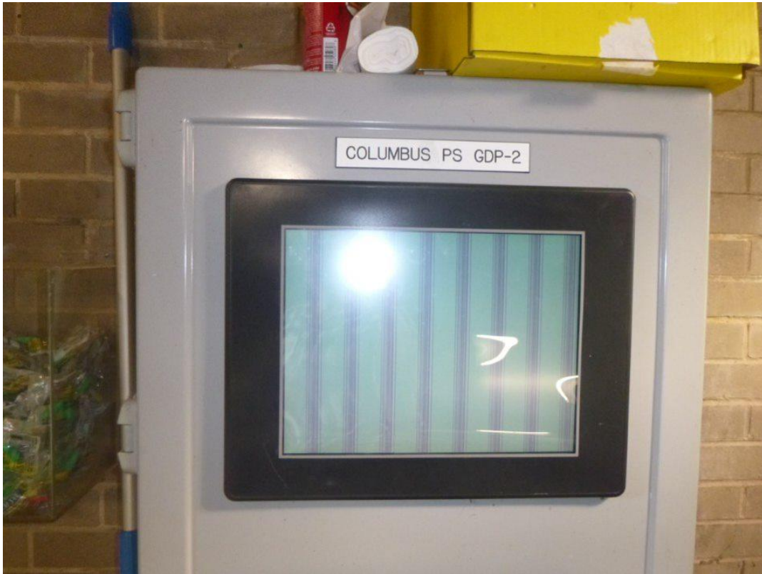
Photograph 91. Programmable logic controller (PLC) out of service at the Columbus Pump Station main building.
