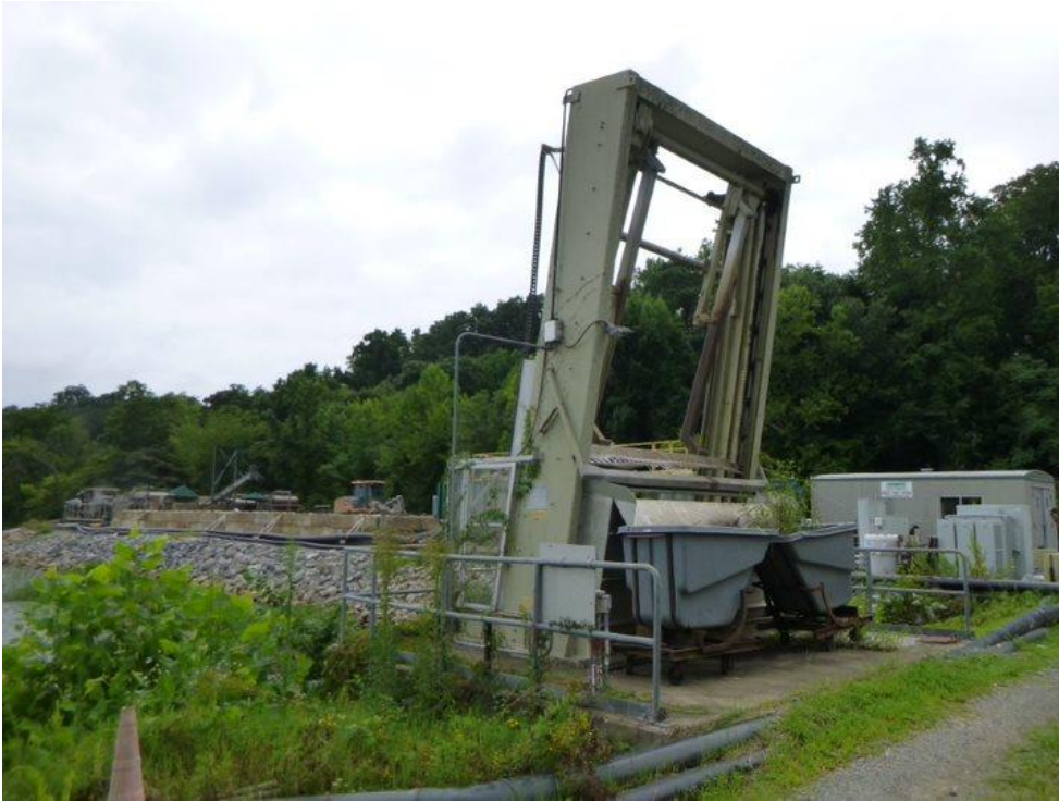
Photograph 5. Bar screen and waste containers with vegetation and other debris.
