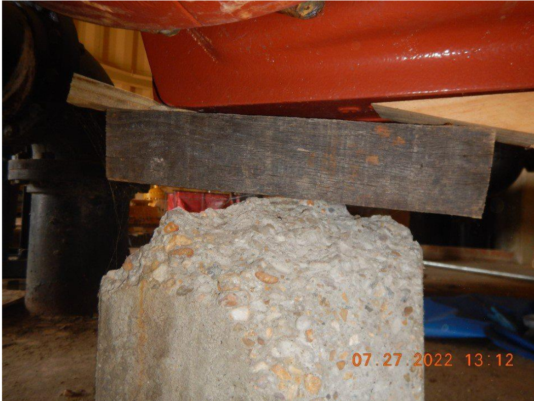
Photograph 83. Pieces of wood stacked to attempt to provide support to the transmission pipe at Warwick Road Tank.
