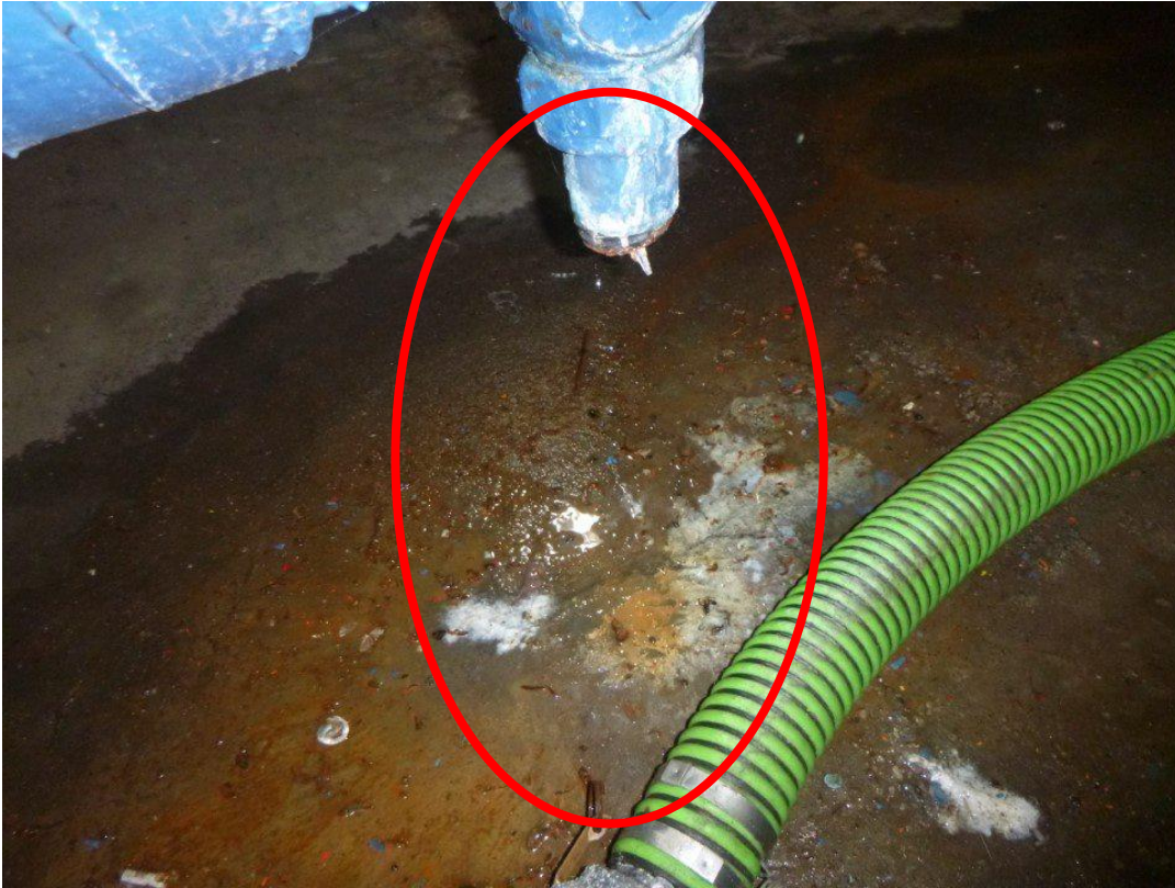
Photograph 49. Fitting leaking from corroded pipe onto floor in Korah 2 and 3 Pump Station.
