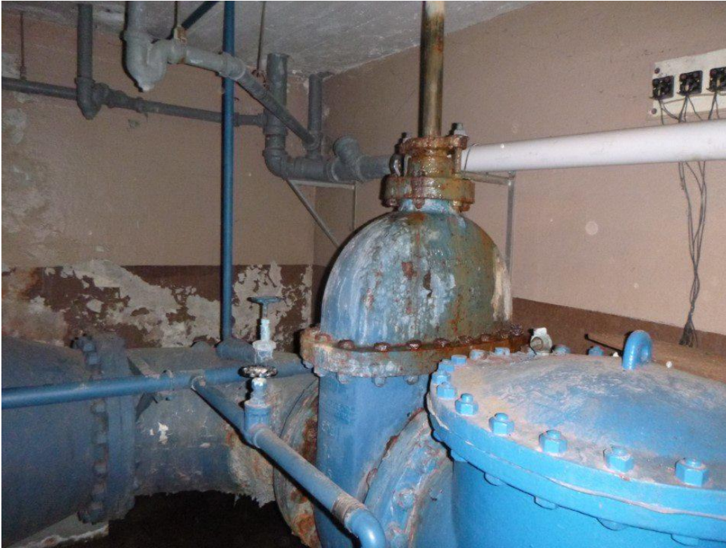
Photograph 99. Leaking seals on gate valves at Byrd Park Main Pump Station.
