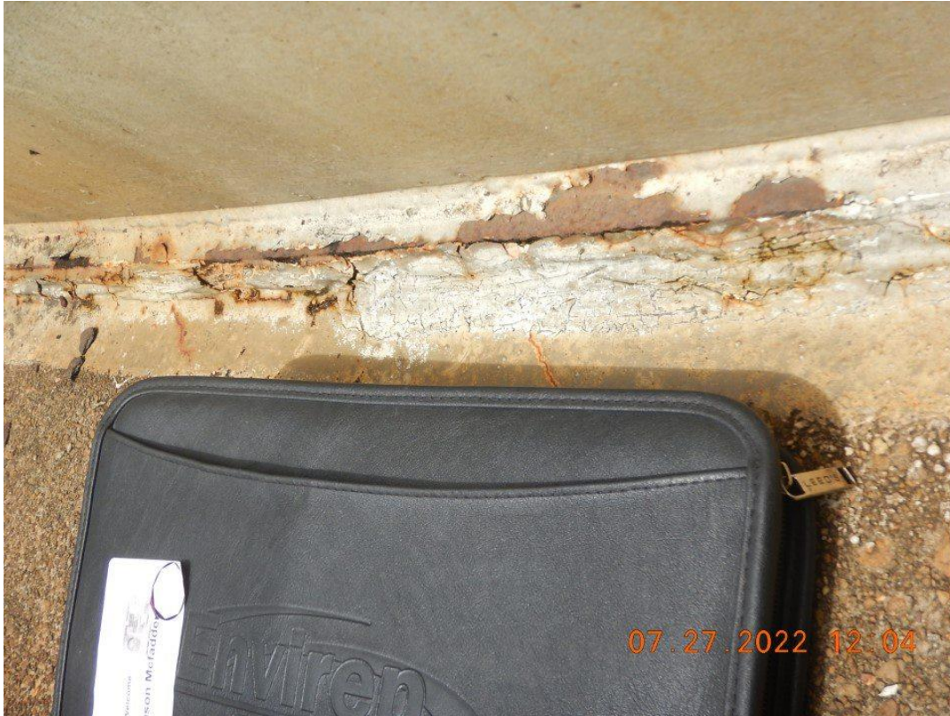
Photograph 79. Corrosion and degraded seal at base of Jahnke Road Tank.
