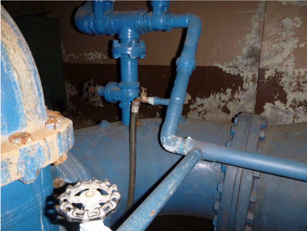
Photograph 105. Hose on ground attached to finished water line without vacuum breaker.
