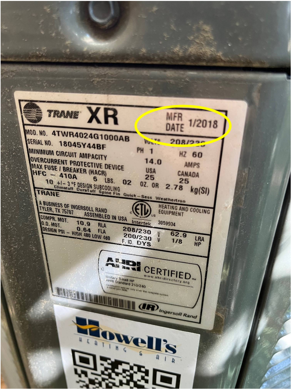
Exhibit C – Upstairs HVAC Units Installed in 2018
