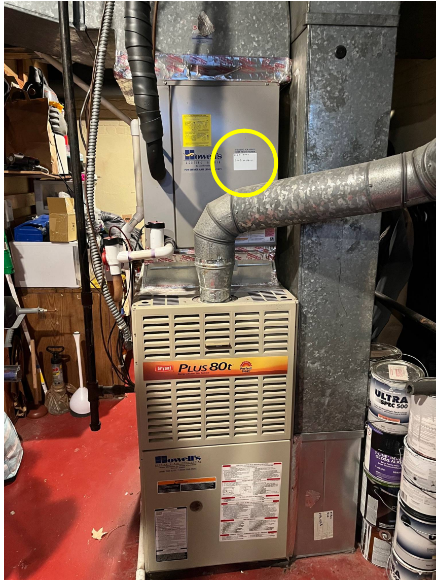
Exhibit B - Downstairs HVAC Unit Installed in 2015
