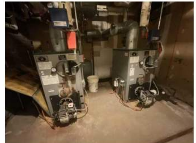
18 - MAIN BOILER HEATING COMPONENT
