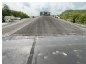
Roofing in Poor condition.
