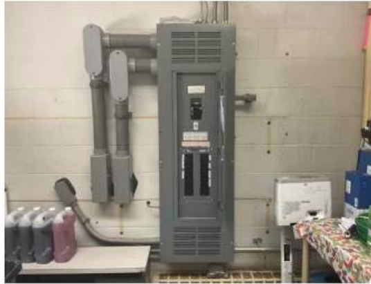
46 - DISTRIBUTION PANEL, 120/208 V, 400 AMP,
