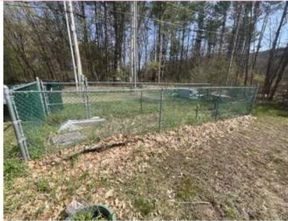
20 - PROPANE STORAGE ENCLOSURE
