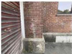
Exterior Walls in Poor condition.
