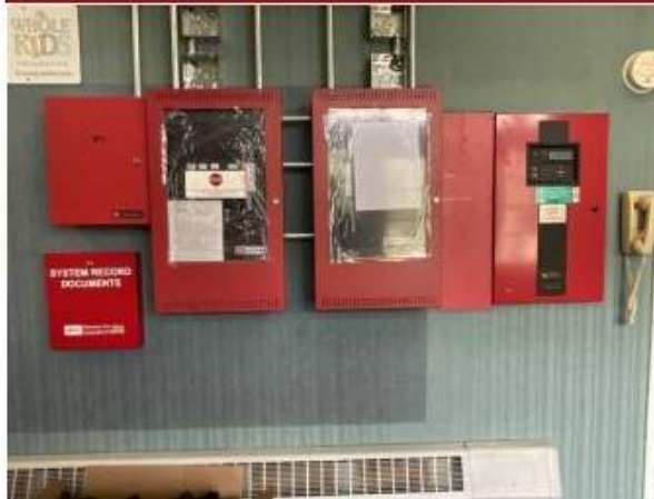
25 - FIRE ALARM PANEL IN LOBBY
