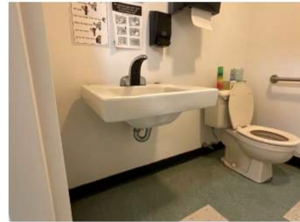
10 - SINK, FAUCET HANDLES
