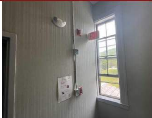
26 - FIRE ALARM DEVICES
