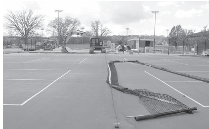
ANNA CIRACI | STAFF PHOTOGRAPHER Construction begins at Purdue's CoRec. The new complex is expected to be open in Fall 2026, including 18 pickleball courts and two tennis courts.
