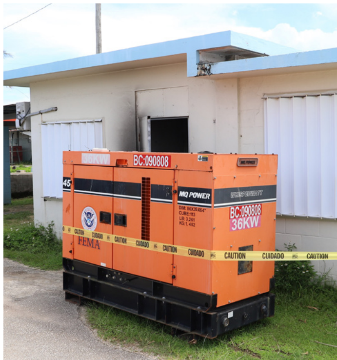
The Generator Provides Power To A Food Distribution Site After Typhoon Mawar, Installed by U.S. Army Corps of Engineer Contractors
