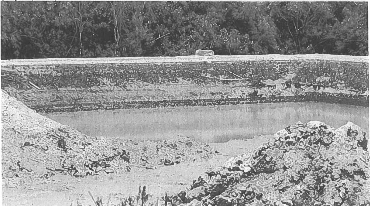
Close up of Pond 1 rim, showing high water mark indicating near-overtopping from prior storm. (July 23, 2021)
