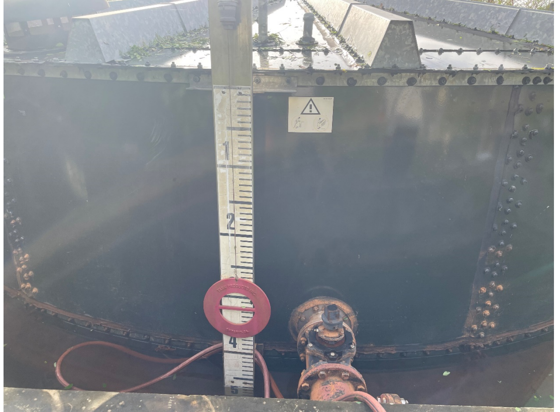
Figure 4. Level of drawdown in the leachate tanks by the morning of the 26 th of May.
