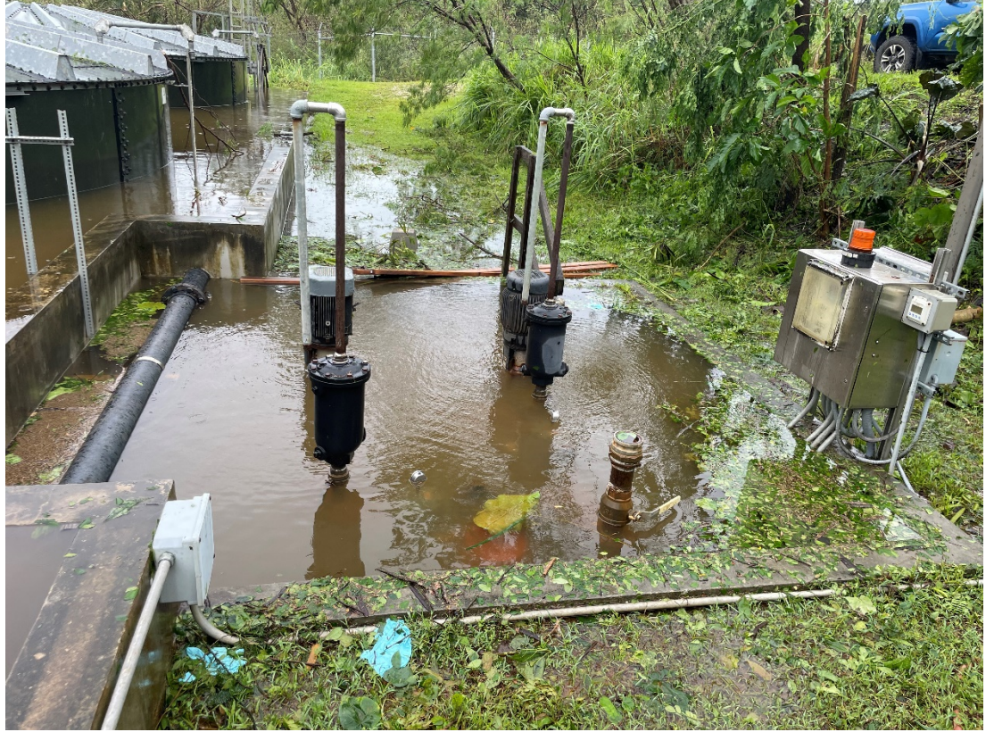
Figure 2. Condition of the Leachate pump station when staff made it back to the site after the storm on the 25 th of May.
