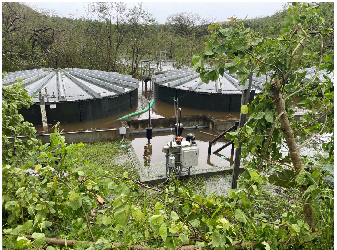
Figure 1. Condition of Leachate tanks and pump station when staff made it back to the site after the storm on the 25 th of May.
