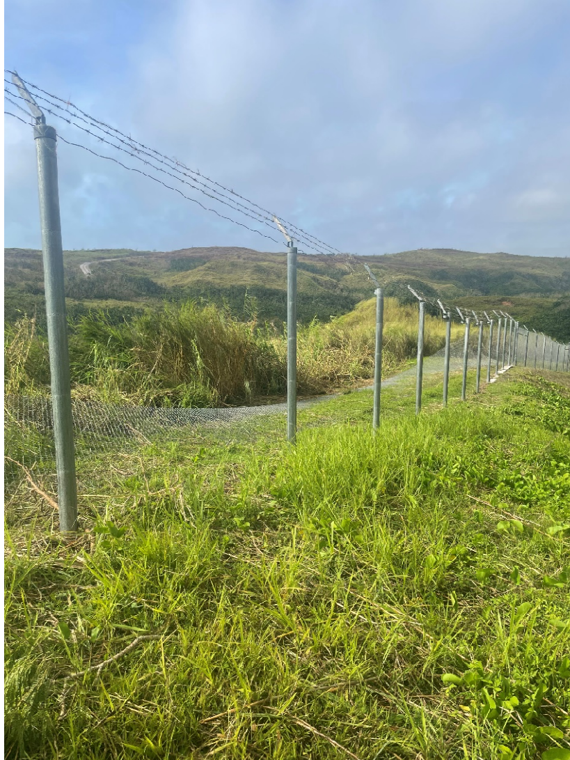
Figure 7. Part of the perimeter fence on the eastern side of the site—damaged during the storm.
