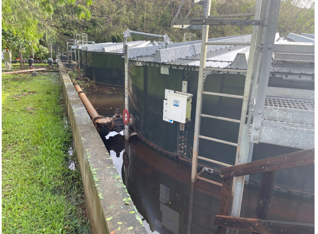
Figure 3. Level of drawdown in the secondary containment due to the use of the portable pump to return the liquid into tank 2 by the morning of the 26 th of May.
