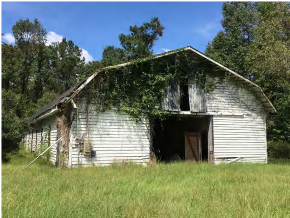
View of a large old barn in poor condition.
