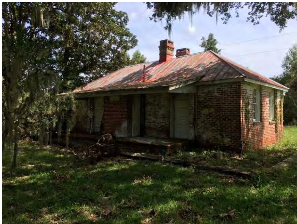
View of bunk house 2 in poor condition.
