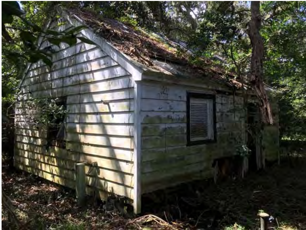
View of an old pump house in poor condition.
