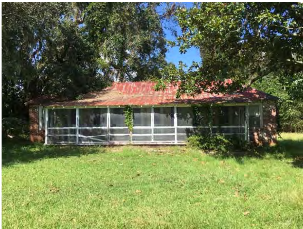
View of bunk house 1 in poor condition.
