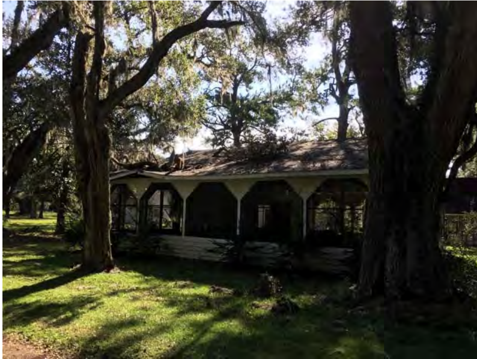
View of the screened shed. The reader will note the roof damage caused by the tree limb.
