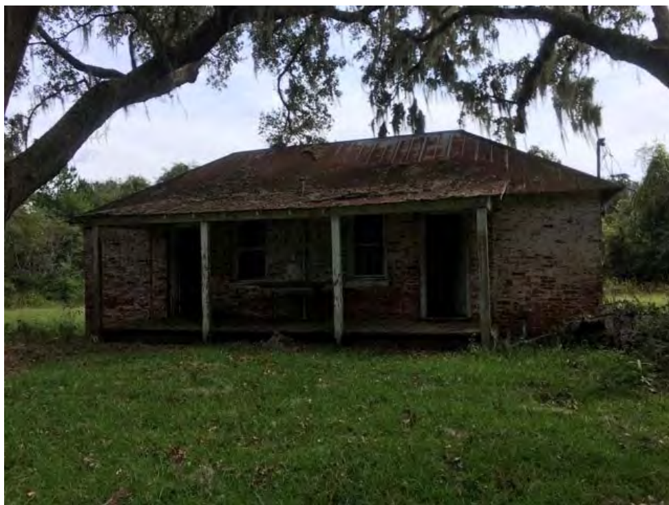
View of bunk house 3 in poor condition.
