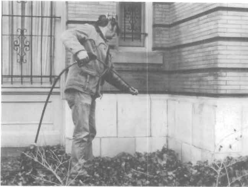
Figure 7. A contractor prepares equipment before testing a low-pressure water wash on a Roman brick and terra cotta building. Photograph: Sharon C. Park, AIA
