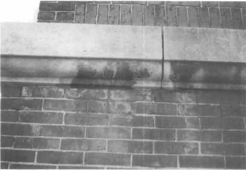
Figure 25. Excess moisture leaching out through the walls has resulted in the formation of white efflorescent salts on the brick and blackish sulfate salts on the limestone water table.
