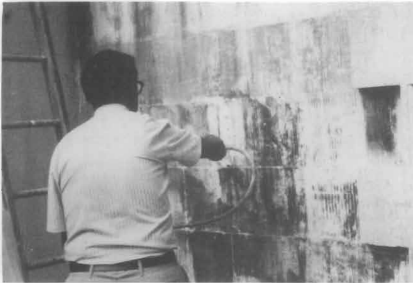
Figures 15a-15b. If a highly articulated facade is being cleaned it may be necessary to scaffold the building, one elevation at a time. When the monumental task of chemically removing all the paint from the White House was begun, each side was scaffolded in preparation for repainting. Removal of the many layers of paint that had obscured the stone tooling marks for almost a century, without damaging the historic sandstone, required much painstaking hand work.
