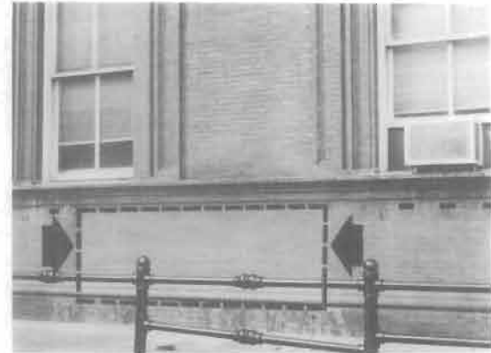
Figure 9. A test patch on brick to remove a century of dirt reveals only a slight difference in appearance between the cleaned and the uncleaned brick. The hard-baked outer skin of the brick provides a surface that is not only impervious to dirt penetration, but resists dirt accumulation. Photograph: Christina Henry
