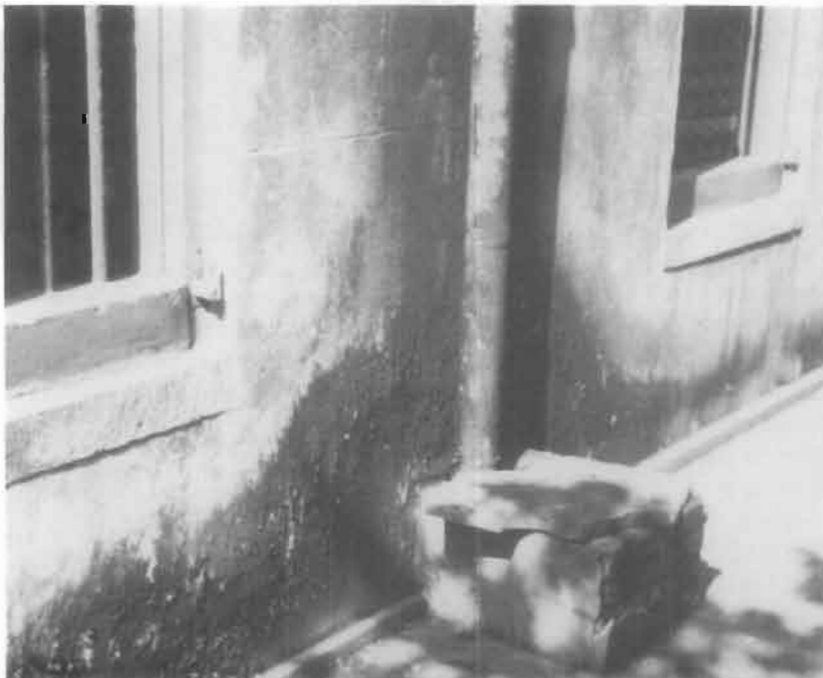
Figure 23. The moss growing around the downspout and along the base of this stucco building clearly indicates the presence of excess moisture—here due to rising damp as well as a leaky downspout. Photograph: Lee H. Nelson, FAIA
