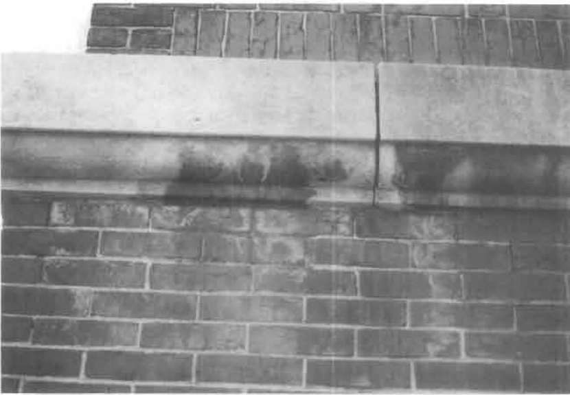
Figure 25. Excess moisture leaching out through the walls has resulted in the formation of white efflorescent salts on the brick and blackish sulfate salts on the limestone water table.
