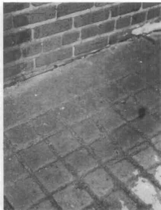
Figure 14. Although the sodium hydroxide-based test cleaning patch on the right side of this wall of common brick appears to have been successfully cleaned, closer inspection reveals that a minute portion of the brick surface has been dissolved and removed by the cleaner. As a result, considerable brick dust can be seen in the cracks of the pavement beneath the wall.
