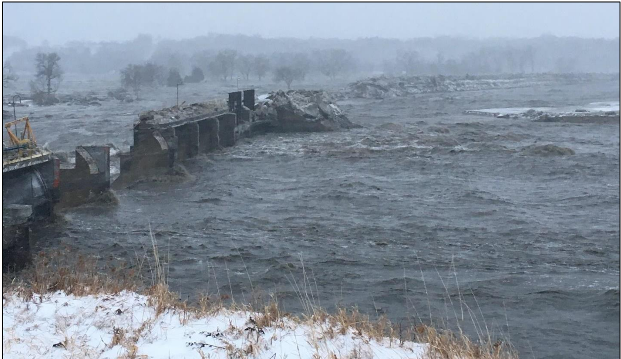
Figure 4.17 – Photo of Spencer Dam taken at 8:04 AM on March 14, 2019 (NPPD photo).
