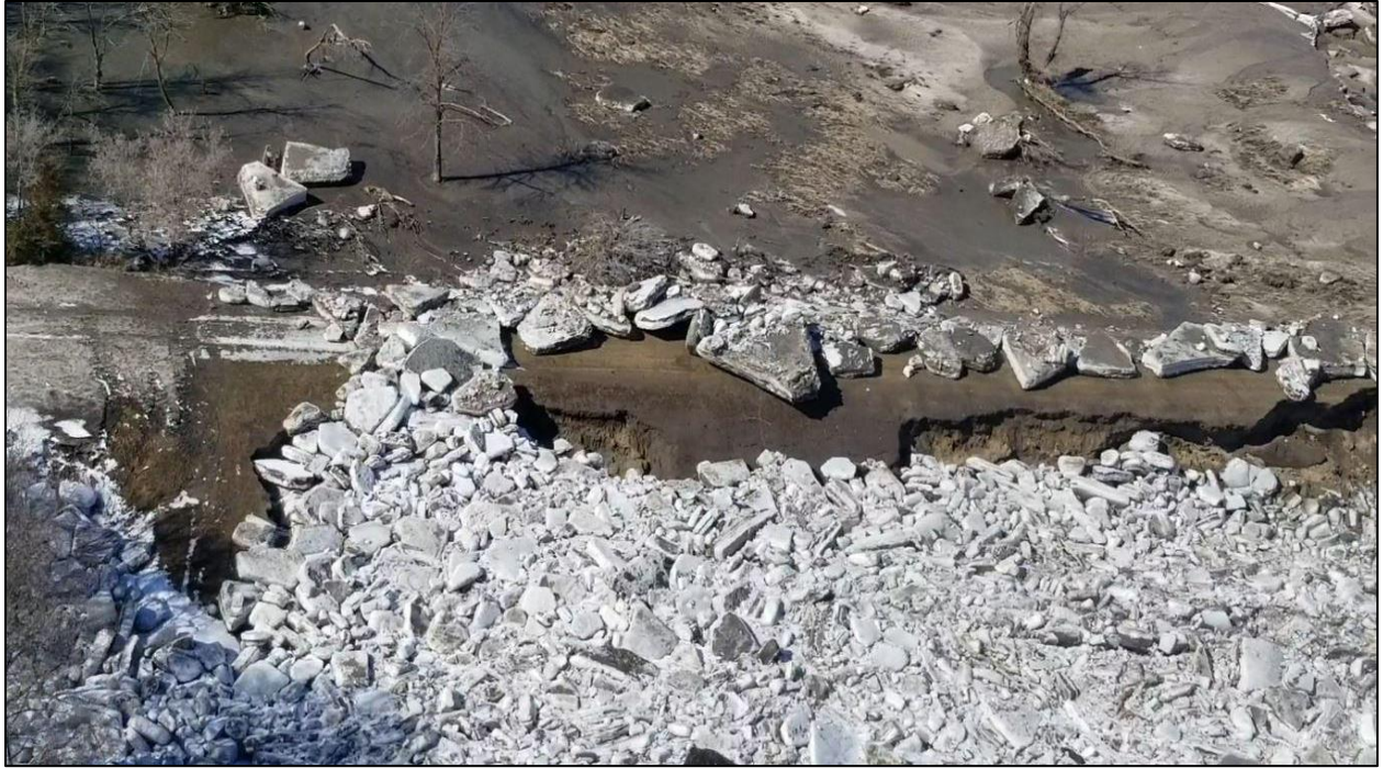
Figure 4.11 – South end of south dike looking upstream showing the headcut erosion on the downstream slope of the dike (NPPD video).
