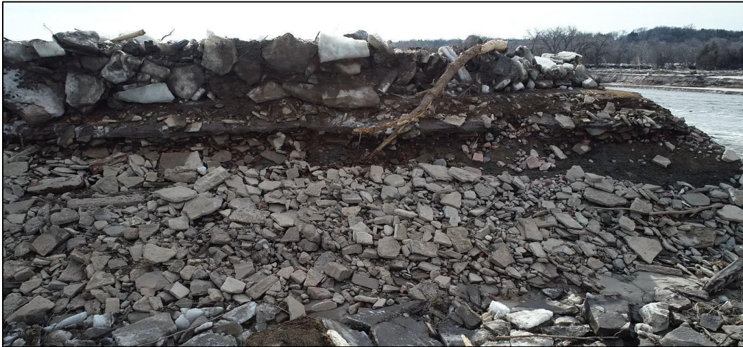
Figure 4.7 – Ice stacked on the north end of the south breach. The elevation of ice measured in the reservoir rim upstream from the powerhouse was about 4.5 feet above the design top of dam elevation (from NPPD video).
