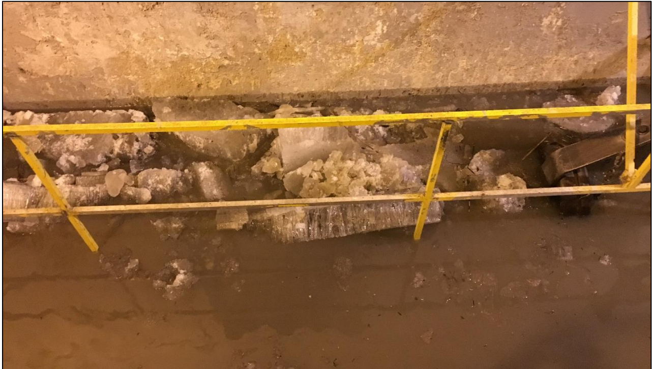
Figure 4.4 – Water and ice entering the trash-rake room at 4:38 AM on March 14. The trashrack slots are behind (upstream from) the railing (NPPD photo).
