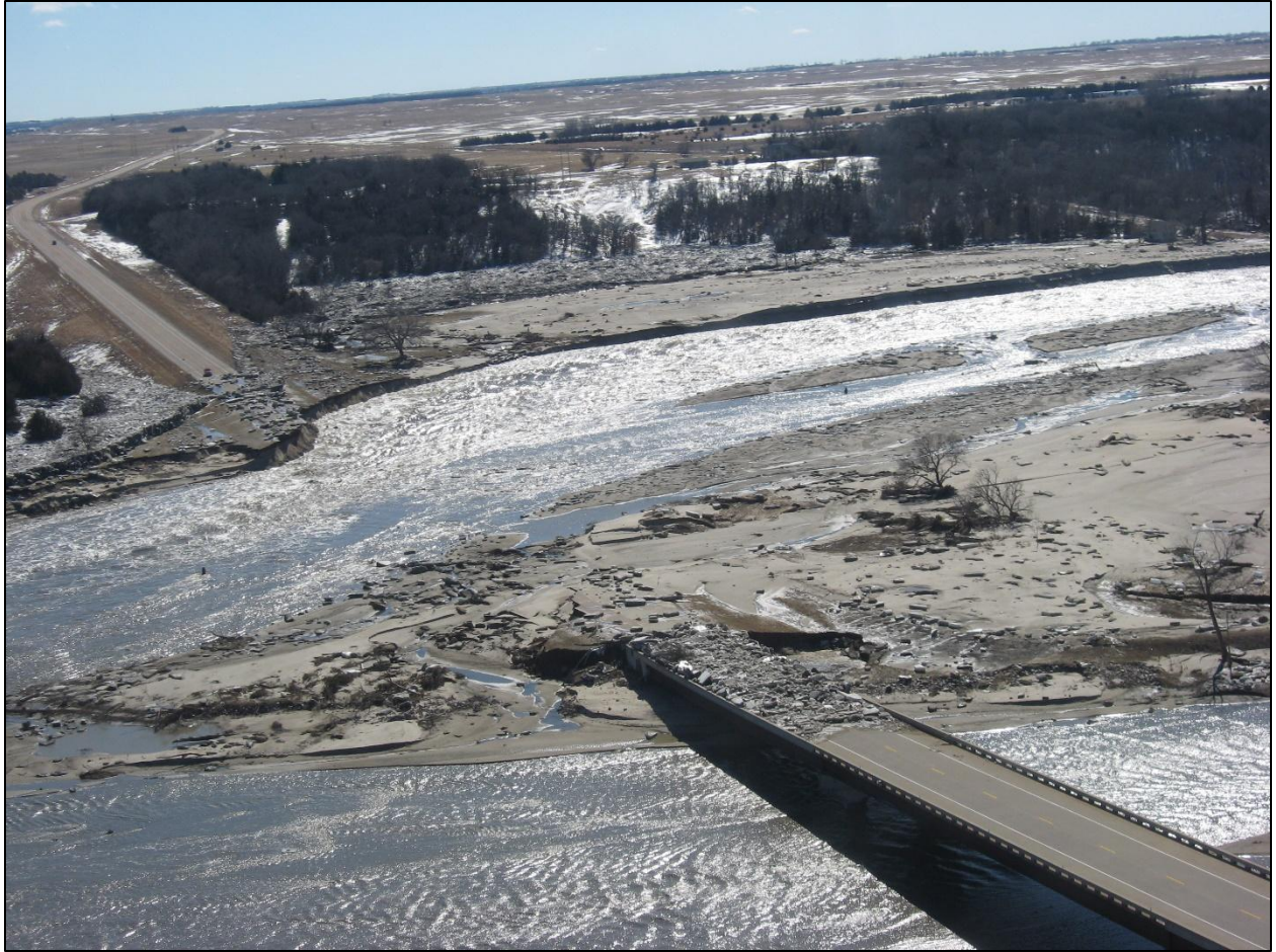
Figure 4.14 – View of washed-out Highway 281 approach ramp (looking south). Note the ice fields upstream and downstream from the road on the south bank (NPPD photo).
