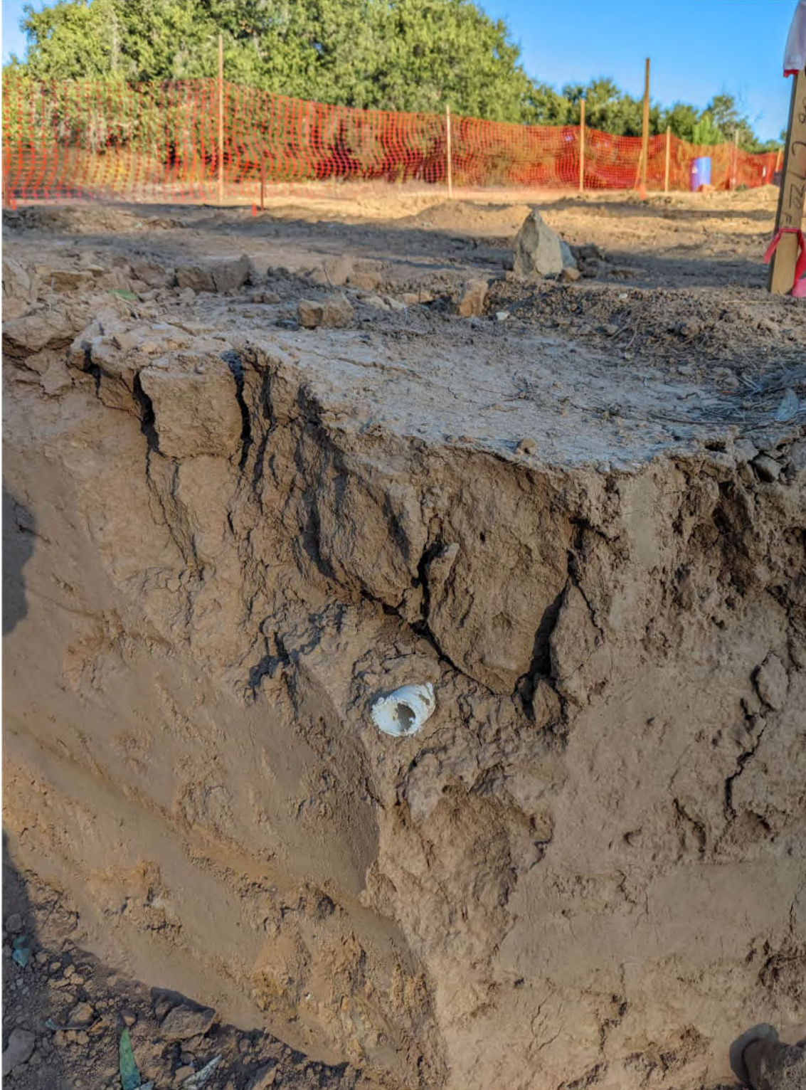
Figure 13. A buried water line is exposed in the cut bank near the northern edge of Grid 5. Water lines likely account for at least two east-west linear features in the southern grids, and may be present in other parts of the site as well. Moisture may partially account for one or both of the grave-like features in the northern portion of Grid 5.
