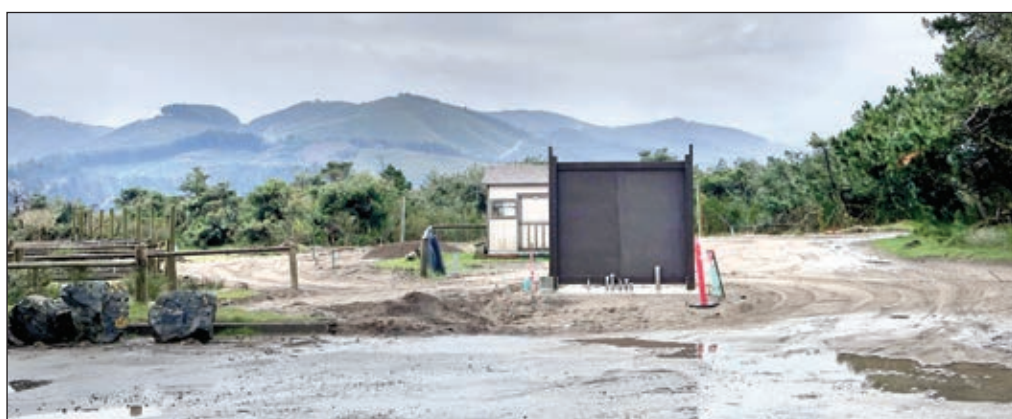
Work in progress to connect the restroom facility at the paddocks used by the park's horse concessionaire to the sewer system.
