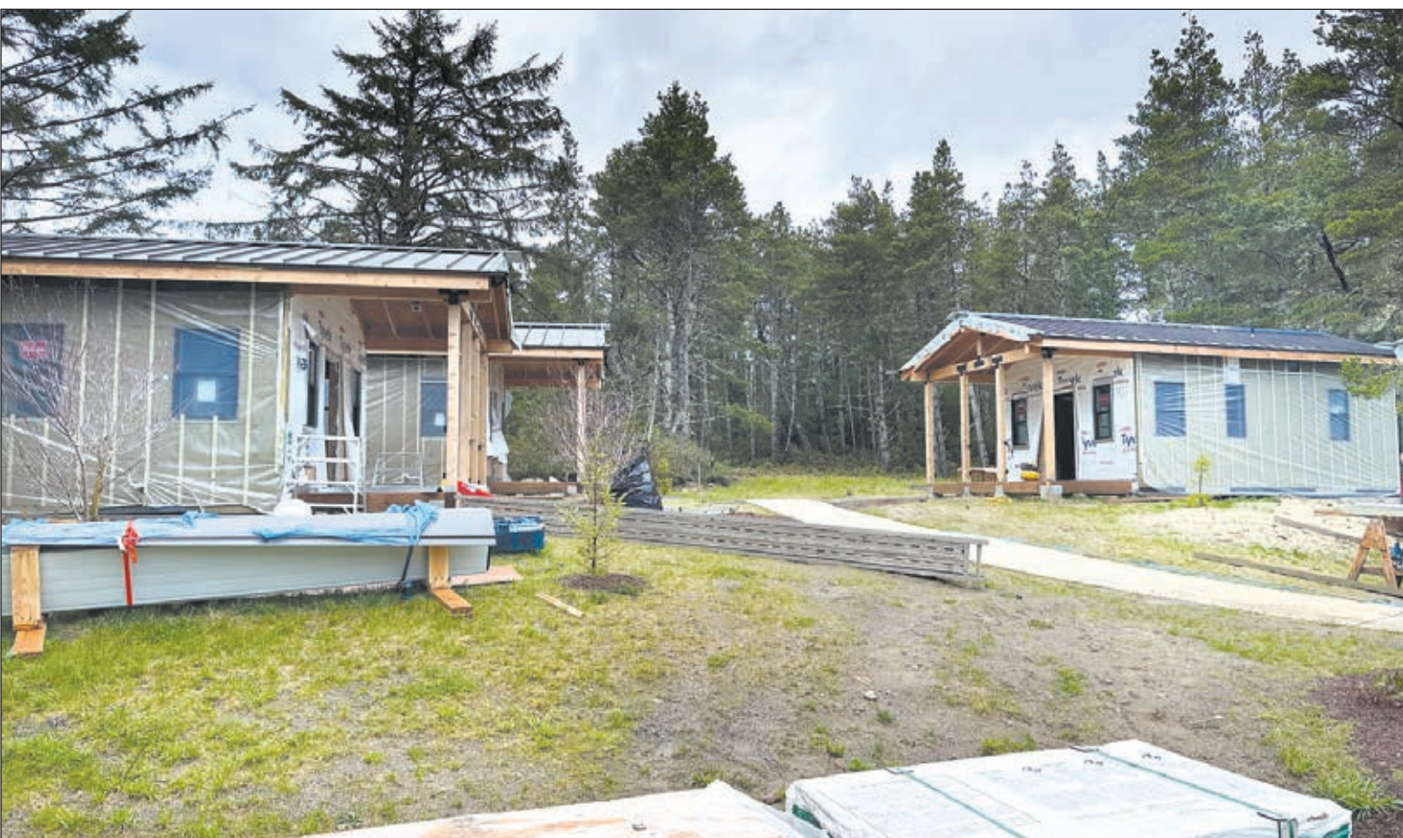
Three of the five cottages being built at the park that will house seasonal staff.
