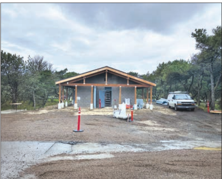
The new bathroom facility between C and D loops at the park.
