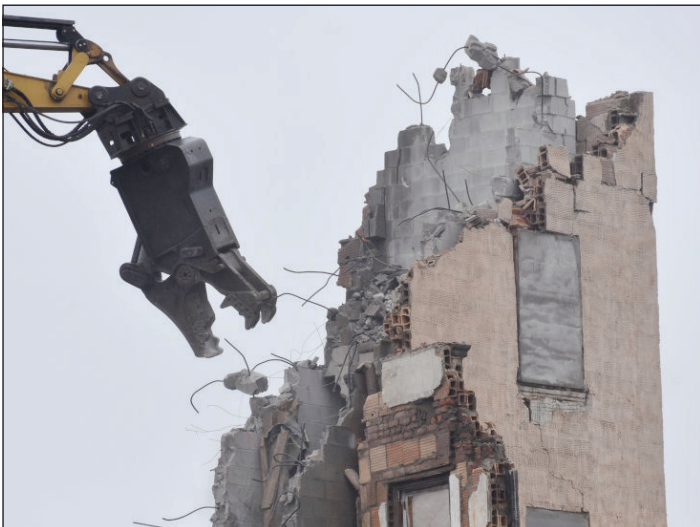
The Flanagan Hotel in Malone is reduced to rubble. Richard Rosentreter photo.
