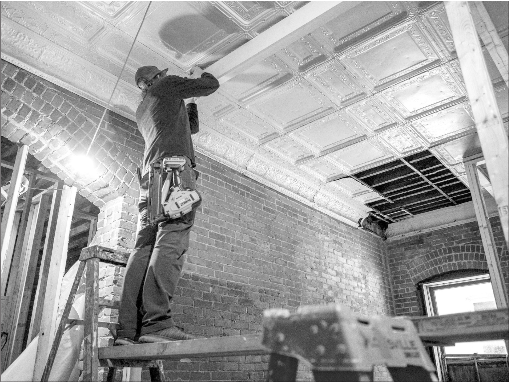
The Scott Phelps General Contracting crew does detailed trim and electrical work on the ceilings inside the former Strand Theater Wednesday. Zachary Canaperi/Watertown Daily Times
