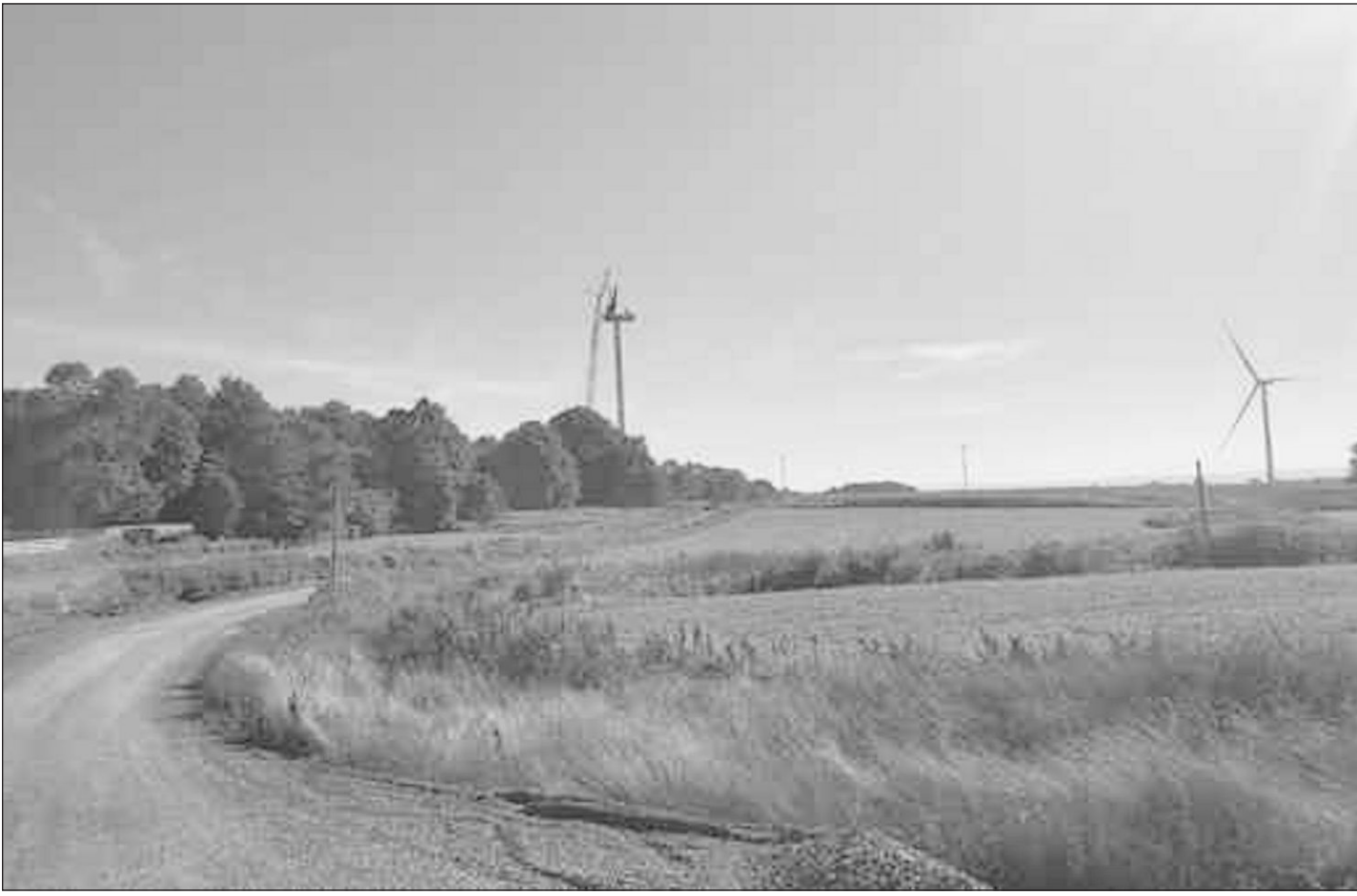
Shown in the final months of turbine construction, Number Three Wind, a renewable energy project developed by Chicago-based Invenergy, is now adding electricity to the grid. The official launch ceremony was held on Thursday morning. Julie Abbass/Watertown Daily Times
