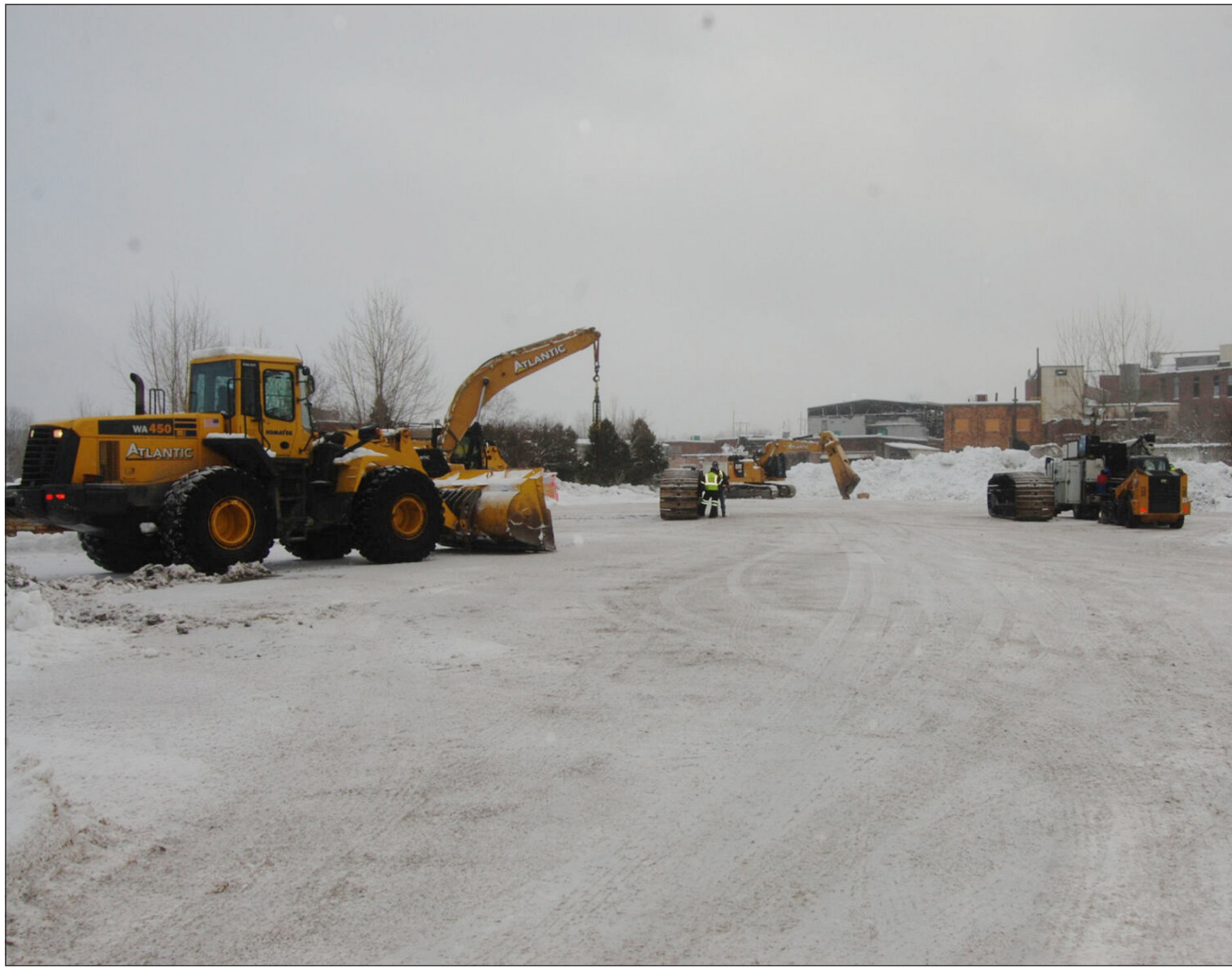
Heavy equipment is staged last winter on the property that housed the St. Regis Paper Mill to demolish unsafe buildings around the Brookfield hydroelectric power plant and along the easement to the facility. Elaine M. Avallone/Johnson Newspapers
