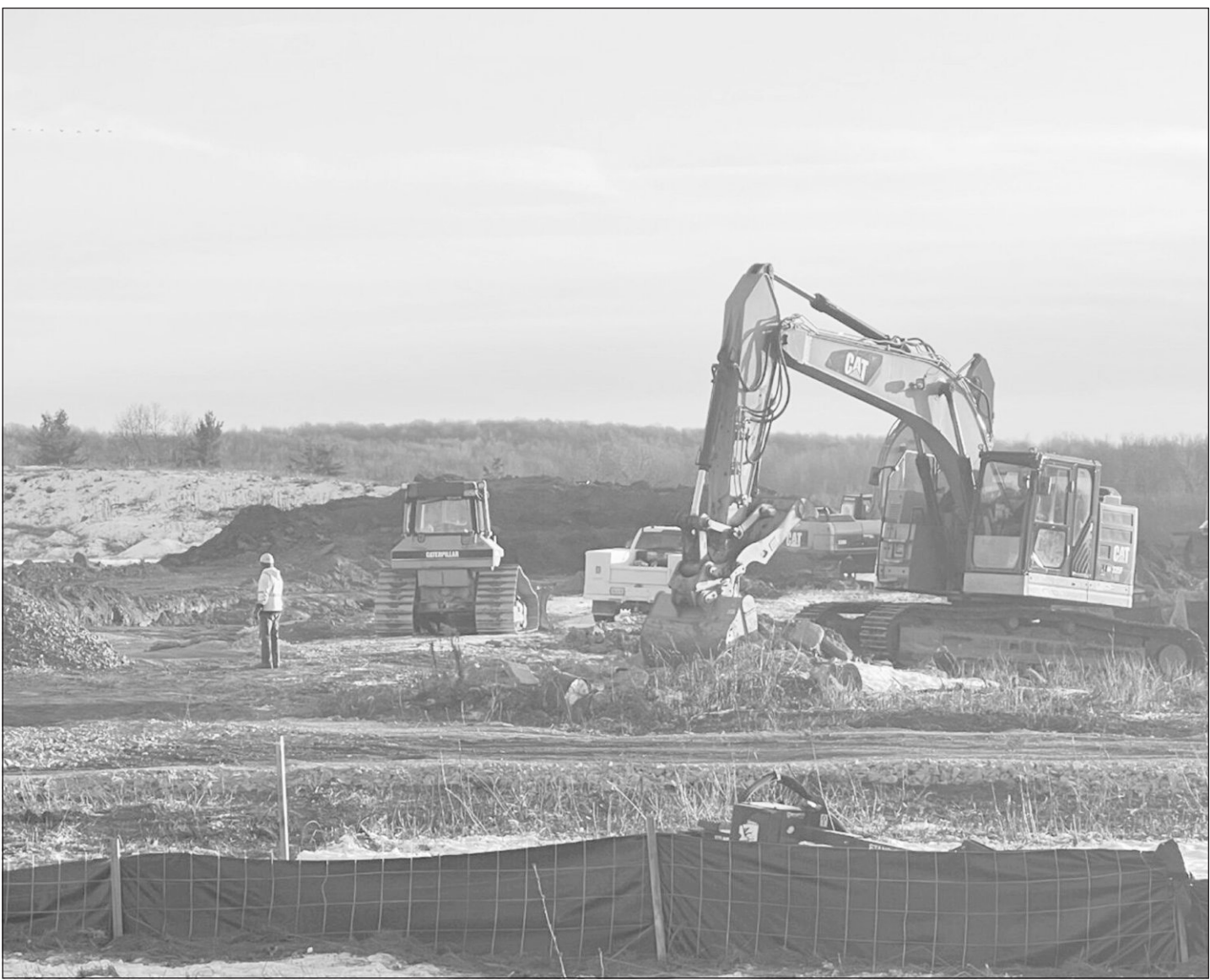
Site work began in December 2022 in preparation for Convalt Energy's 315,000-square-foot solar panel manufacturing plant near the Watertown International Airport in the town of Hounsfield. Jonathon Wheeler/Watertown Daily Times
