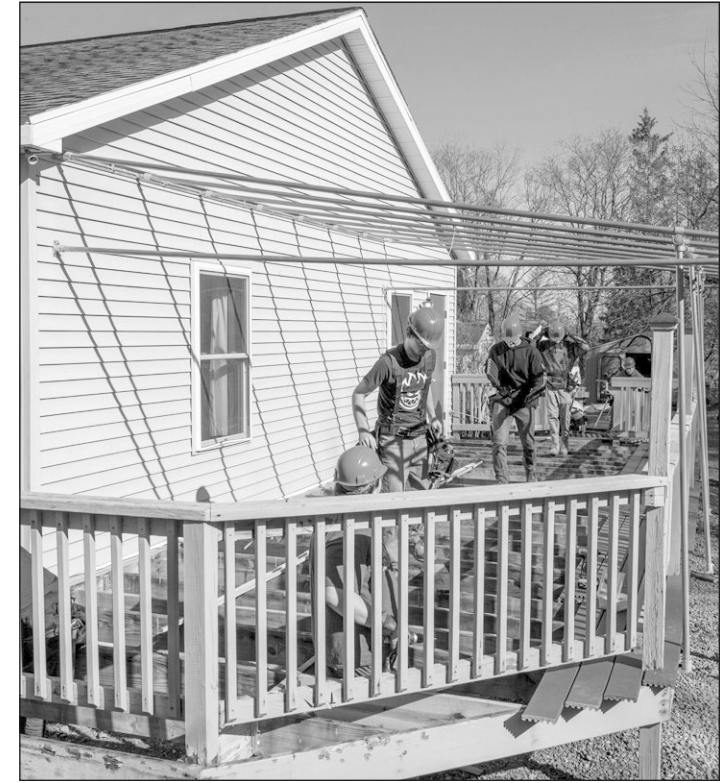
Students with Jefferson-Lewis Board of Cooperative Educational Services (BOCES), work together to construct a wrap around porch for the Arc Facility in Lowville. Zachary Canaperi/Watertown Daily Times
