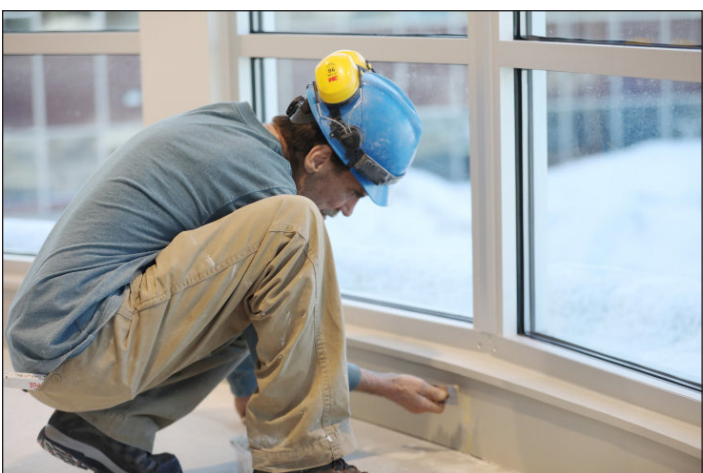
Employee for Design Build Innovations, or DBI Billy E. Decilles working inside the new Watertown Savings Bank lending center on Clinton Street. Jonathon Wheeler/Watertown Daily Times
