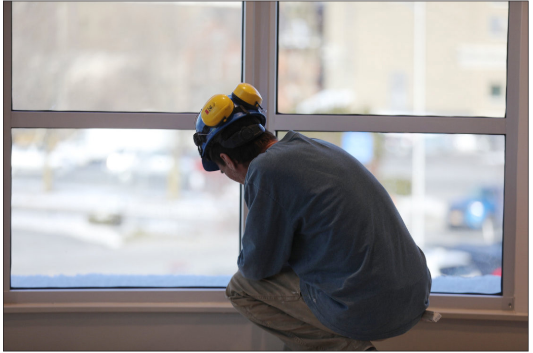
Employee for Design Build Innovations, or DBI Billy E. Decilles working inside on the new Watertown Savings Bank lending center on Clinton Street. Jonathon Wheeler/Watertown Daily Times
