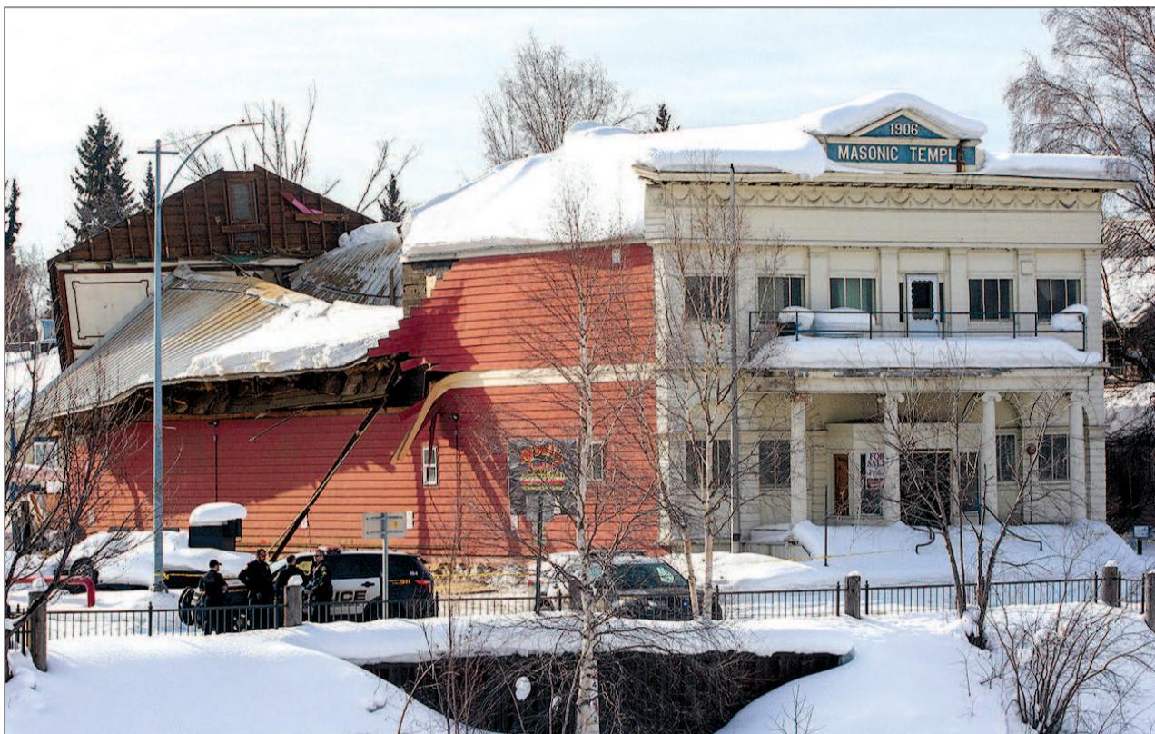
The Masonic Temple, built in 1906 and one of Fairbanks’ oldest buildings, was irreparably damaged Saturday afternoon when the roof collapsed. No one was injured, but people had been inside only minutes earlier. On Thursday, the roof of F & H Fitness Studio in south Fairbanks also collapsed. Nobody was injured. ROBIN WOOD/NEWS-MINER PHOTOS
