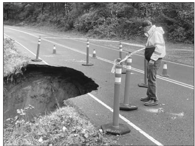
Justin Scharbrough, Newport Public Works superintendent, observes a sinkhole that opened up in October on Oceanview Drive.
