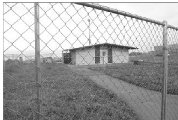
Fencing has been placed around the wayside restroom marking the start of the improvement project.
