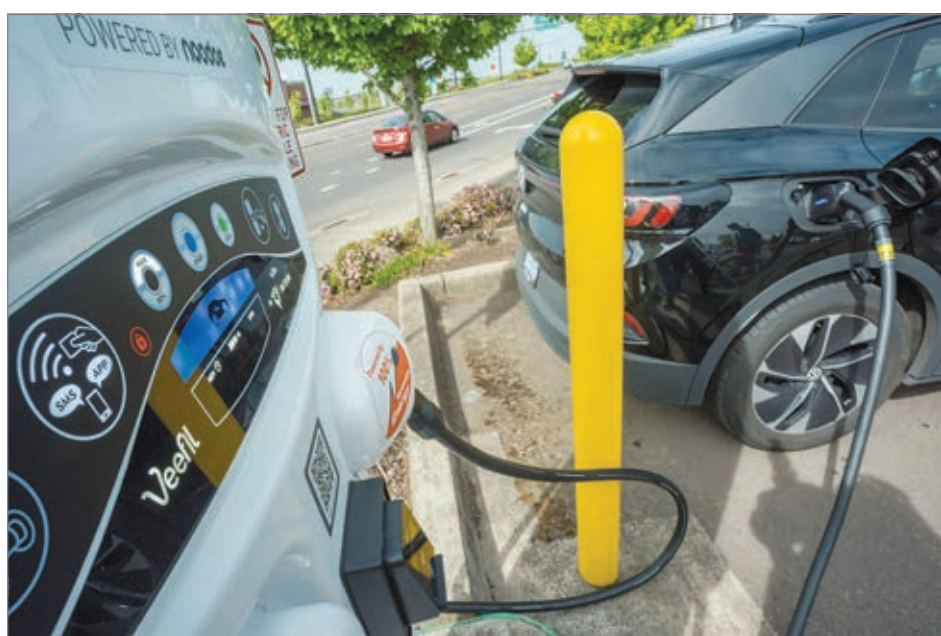
An electric vehicle is charged at the Woodburn Transit Facility in Oregon on May 24, 2022. (Courtesy from the Oregon Department of Transportation)
