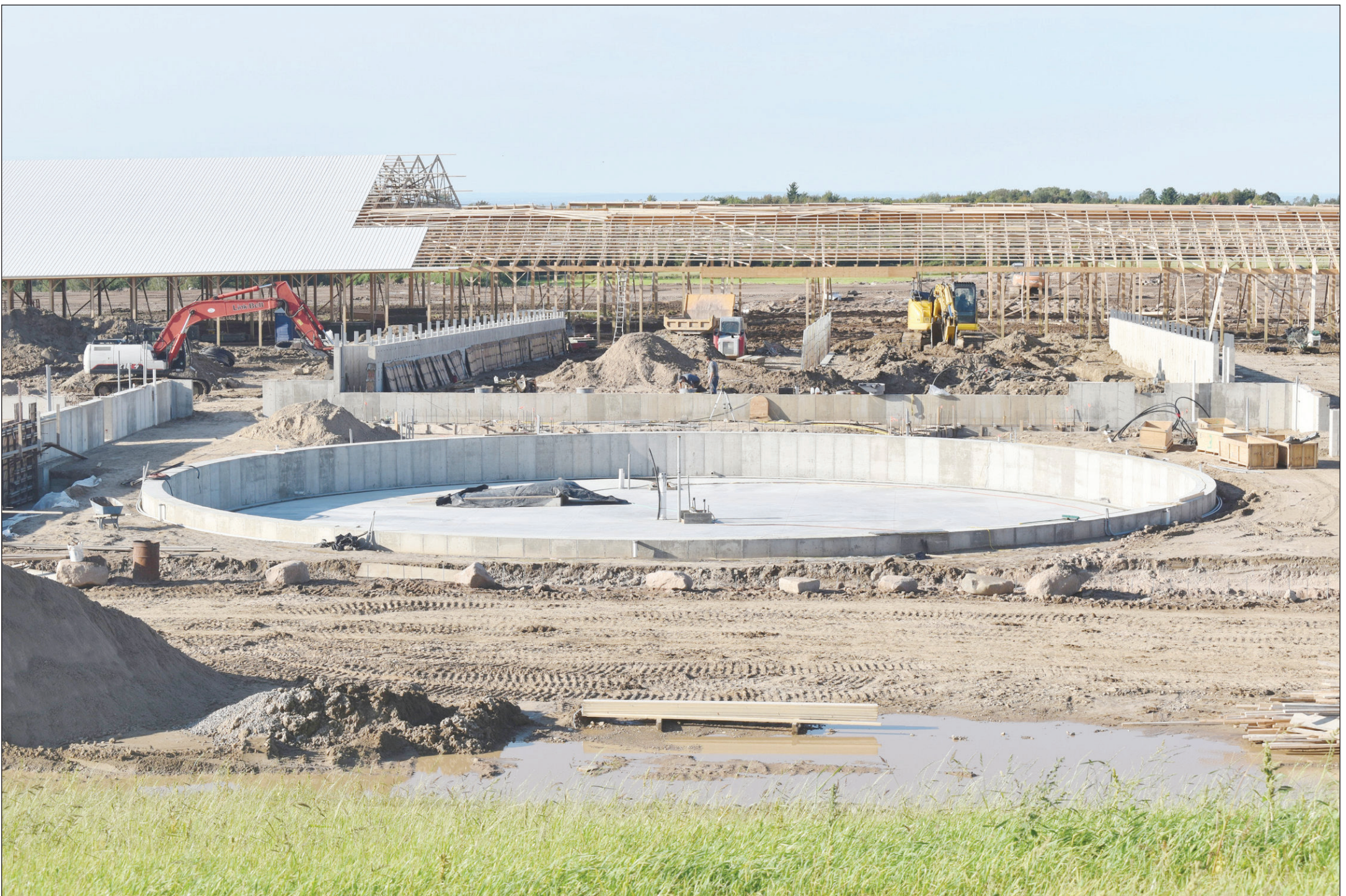
The rotary milking unit at Bilow Farms as seen under construction last year – it is slated to be completed this year. The barn in the background is also nearing completion and will house some of the dairy cows at the farm. PHOTO BY RICHARD ROSENRETER
