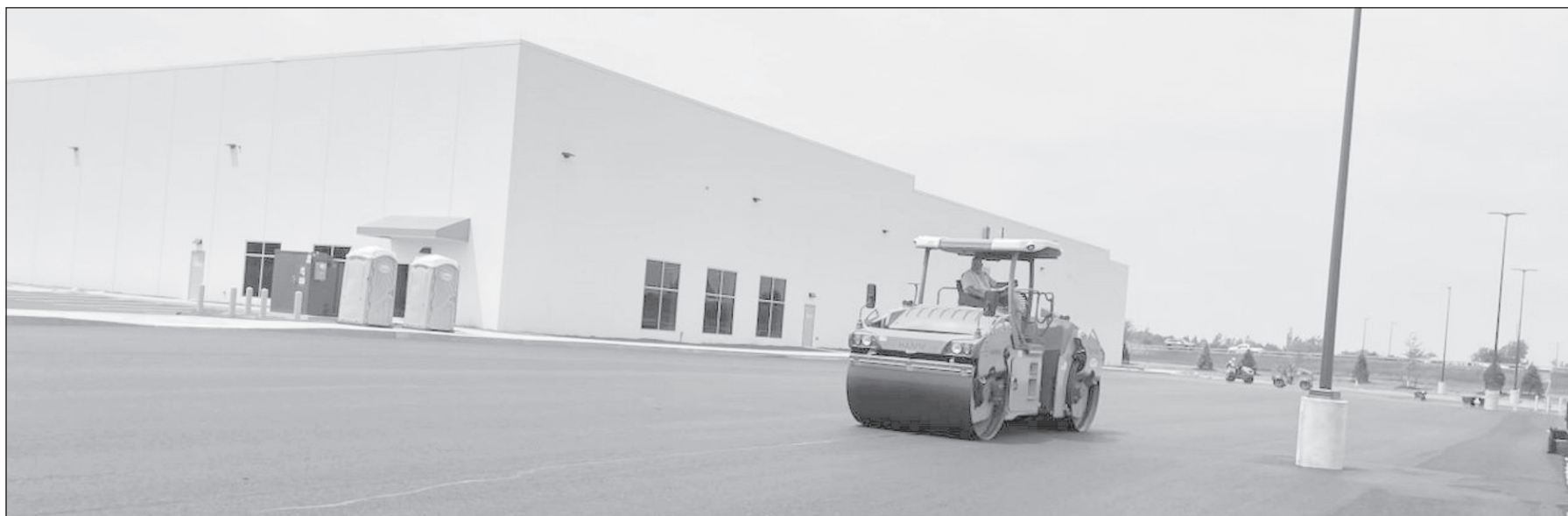
The north country's first Amazon distribution center — expected to be in operation this fall — sits between Interstate 81 and the UPS facility behind the Caprara Honda dealership in the Bradley Street Commerce Park. Construction of the 77,400-square-foot facility 'is essentially done,' according to Byron DeLuke, development director for the Montante Group. Craig Fox/Watertown Daily Times
