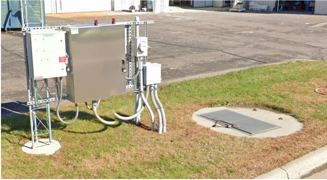
Picture of a feeder lift station within the project area with access locked.
