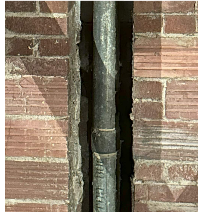
COMPROMISED STRUCTURE AT BATHROOM VENT
