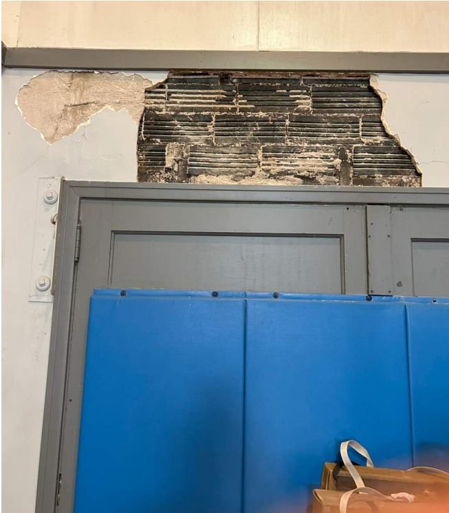
DAMAGE AT GLASS BLOCK LEAK
