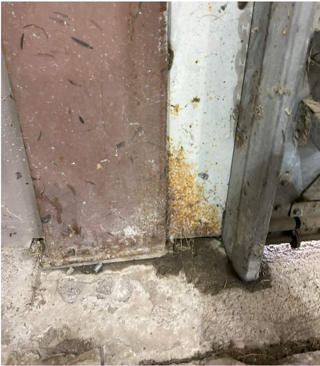
MOISTURE INTRUSION AT BASE OF WALL
