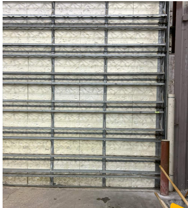
PUCK DAMAGED OVERHEAD DOOR
