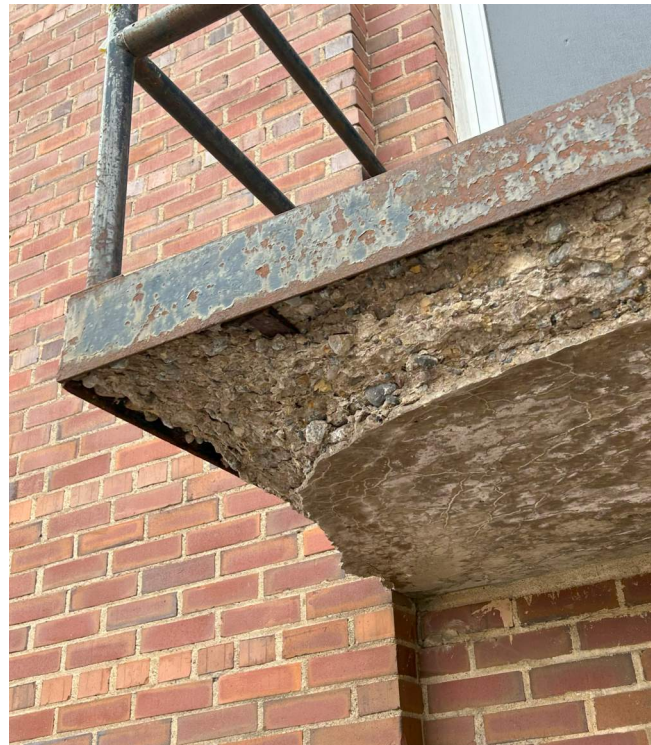
FAILING LANDING AT EGRESS STAIR
