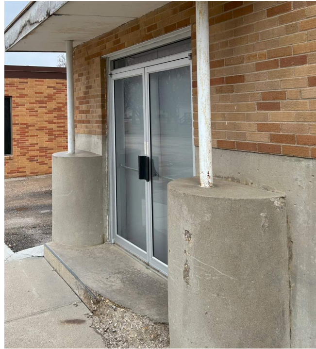
INACCESSIBLE ENTRANCES/SPALLING STOOP
