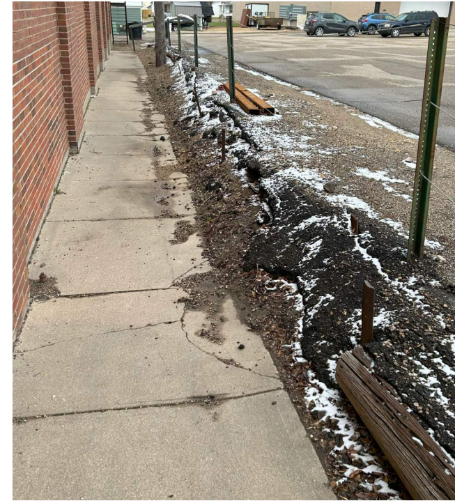
POOR DRAINAGE/BAD FENCE AT PARKING LOT
