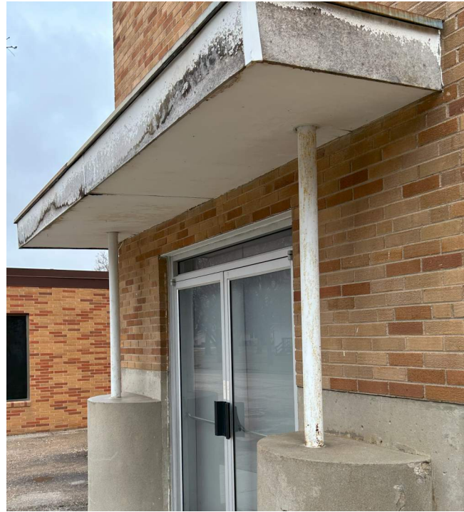
FAILING ENTRY CANOPY
