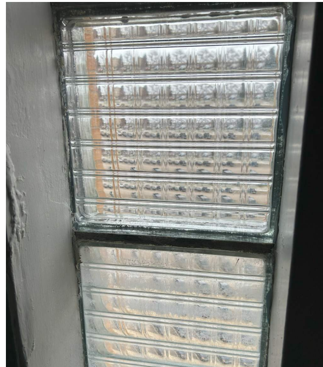
FAILED GLASS BLOCK
