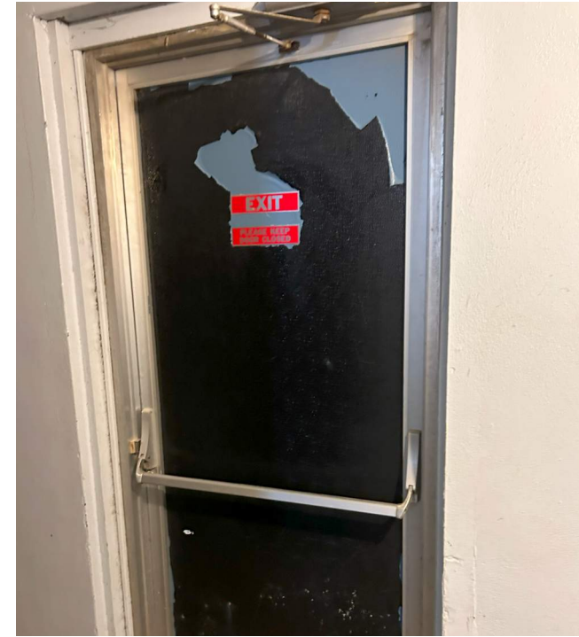
1980s ALUMINUM FRAMES AND FAILED PANEL
