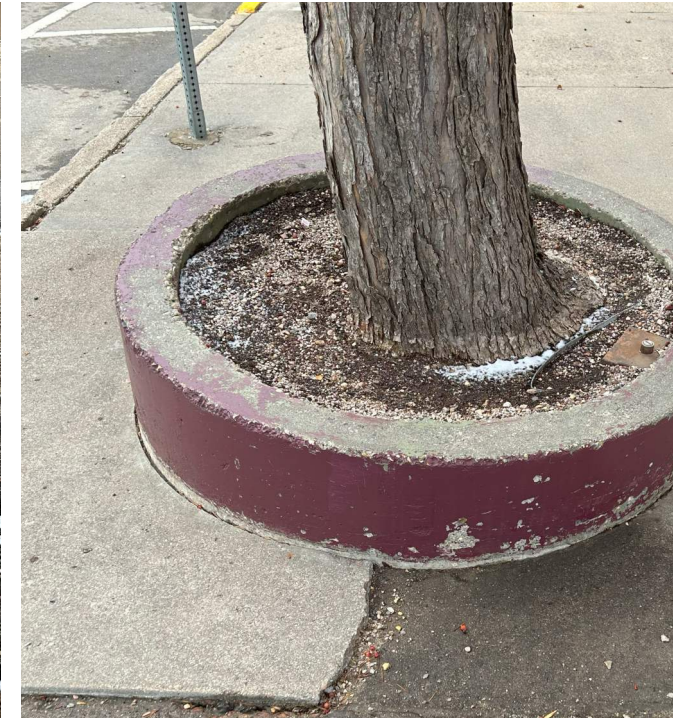
HEAVED PLANTERS/CRACKED WALK
