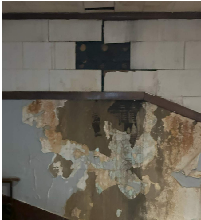
MOISTURE INTRUSION AT ROOF LEAKING
