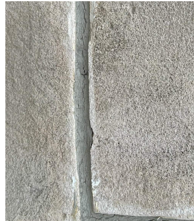
DRY ROT/FAILED SOFT JOINTS AT LIMESTONE
