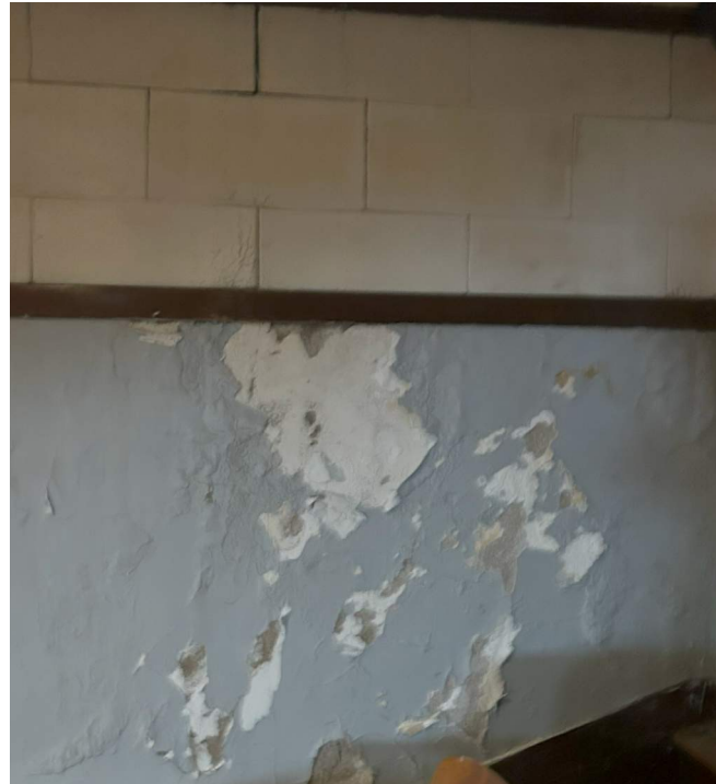
MOISTURE INTRUSION AT ROOF LEAKING
