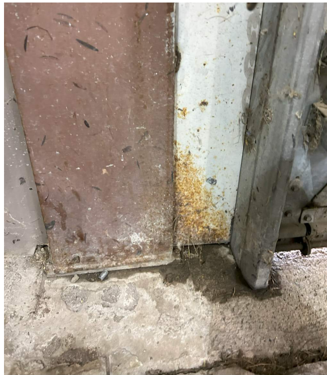
MOISTURE INTRUSION AT BASE OF WALL
