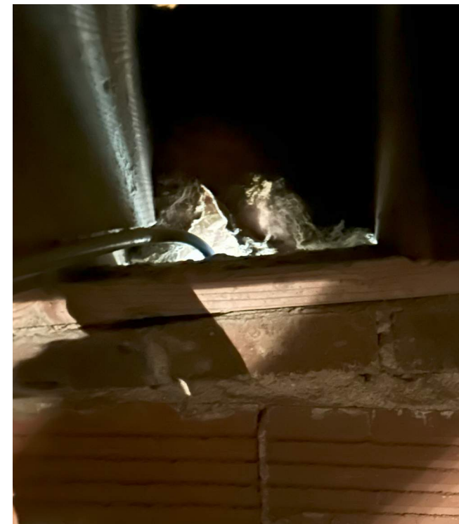
DAYLIGHTING BLEEDING THROUGH IN ATTIC
