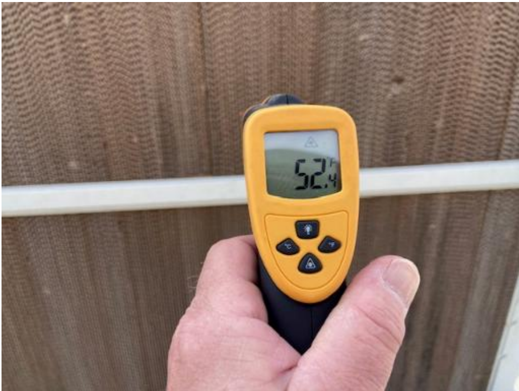
Figure 2 Evaporative cooling tower
