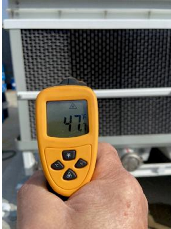
Figure 4 Dry cooling tower
