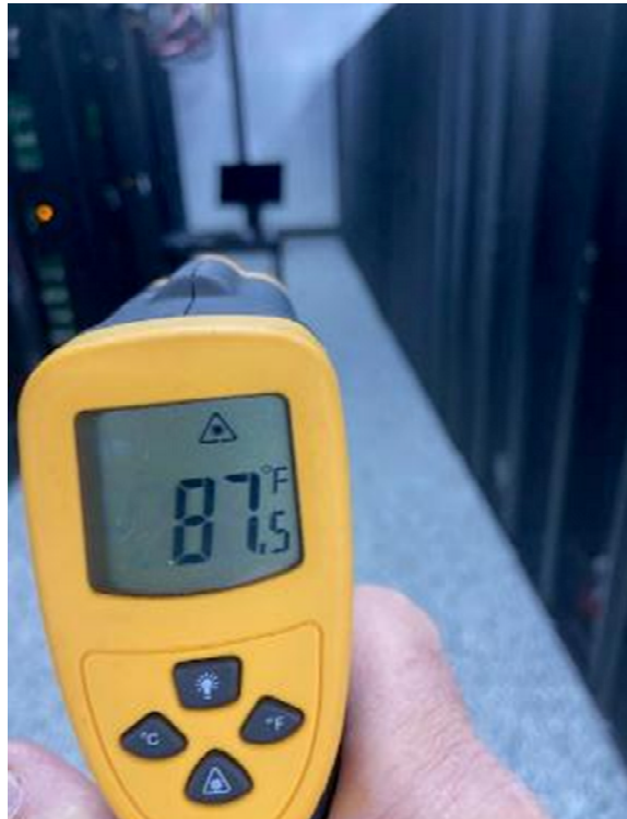
Figure 9 Server Rack air temp
