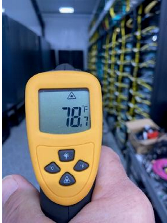
Figure 10 CRAC air temp
