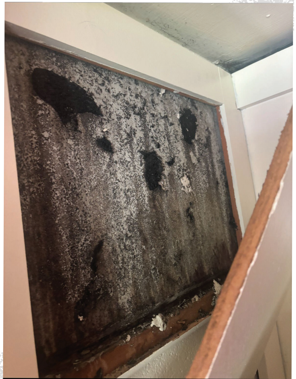
Mold coats the wall of Emma Leo's closet in her 2-bedroom Craighead apartment.
