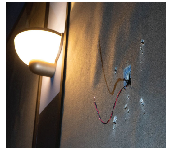
Loose wire seen on the left wall of theater three in The Roxy on Sept. 1.
