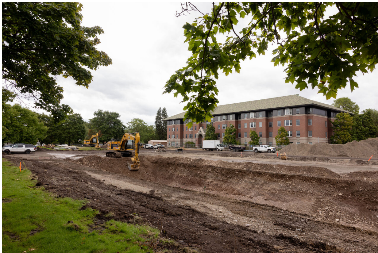
The University of Montana clears room for a new residence hall on Sept. 13, digging up what was formerly parking lot H.
