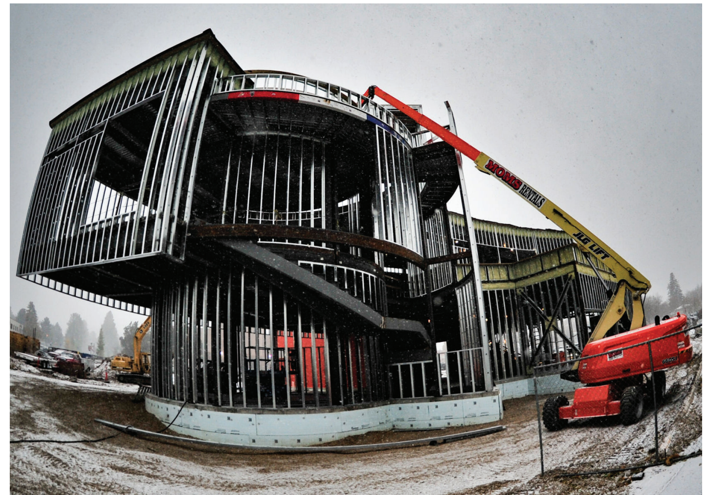
The Missoula Museum of Arts and Culture is under construction and is projected to open Fall of 2023. GRIFFIN ZIEGERT | MONTANA KAIMIN
