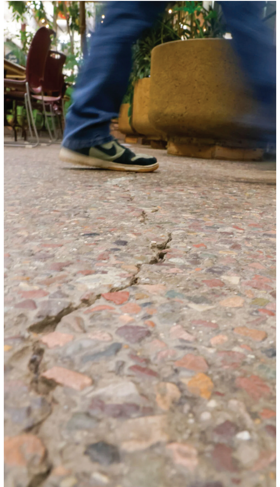
A student walks over the cracked floor of the University Center on April 3. The damage indicates that the ground beneath the UC is shifting, which could impact the glycol heating system, the only source of climate control in the UC atrium. WESTON FUDGE | MONTANA KAIMIN
