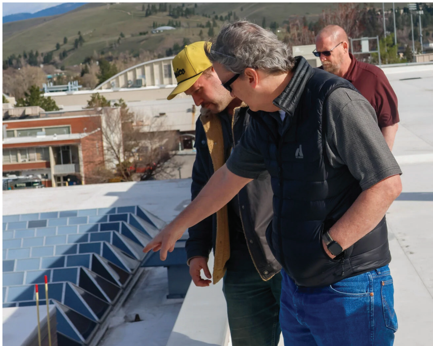
Mike Eglin, architect at the University of Montana, shows Jake Kobza, representing Versico Roofing Systems, sections of the UC roof that need work on April 7 during a contractor bid. Western Montana Roofing, Taylor Bradley Roofing and Ace Roofing were also present. WESTON FUDGE | MONTANA KAIMIN
