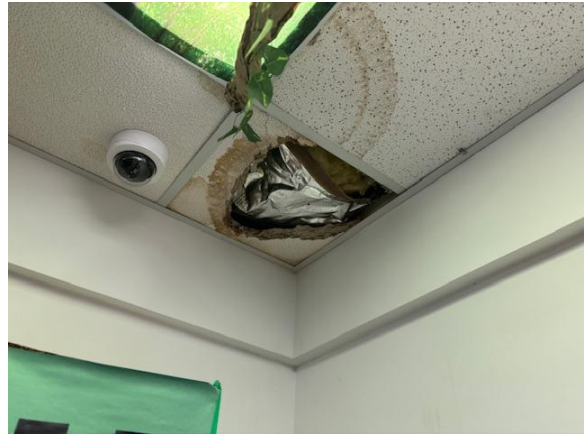
Figure 2 – Water intrusion area – back corner of juvenile area
