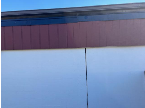
Figure 7 - Poor flashing and sealing
