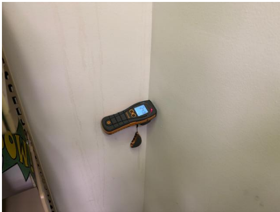
Figure 3 - Elevated moisture in drywall below
