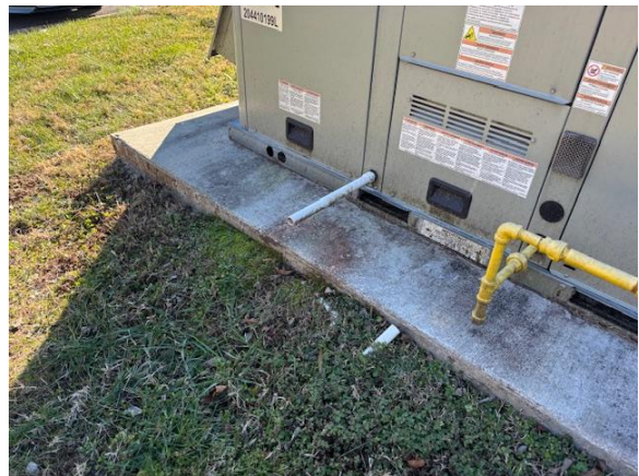
Figure 10 – No condensate trap on HVAC systems
