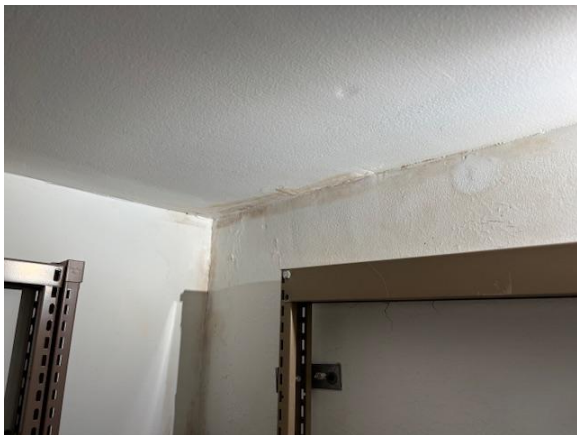
Figure 5 - Water damage in "large print" Section
