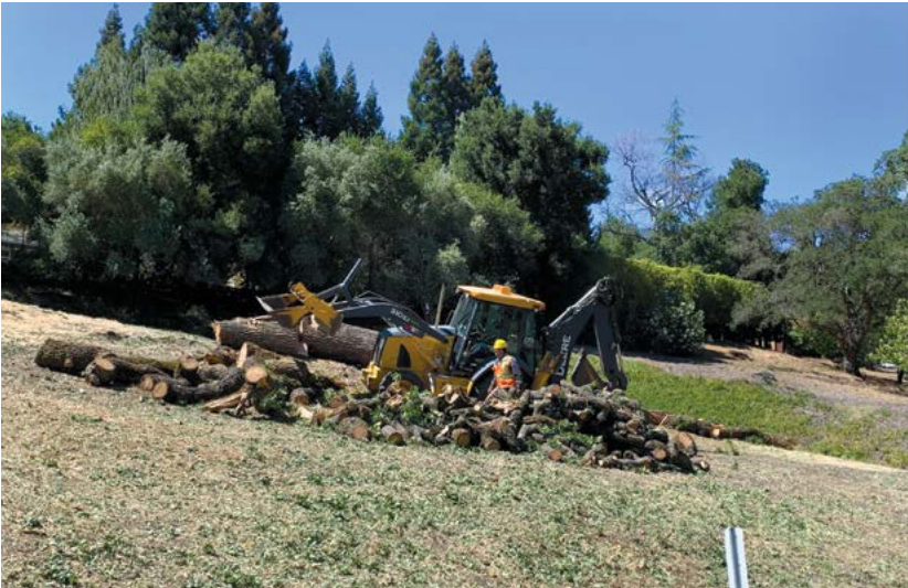
Los Altos Hills town maintenance staff clean up the remains of the fallen tree. PHOTO BY GEORGE CLIFFORD | SPECIAL TO THE TOWN CRIER
