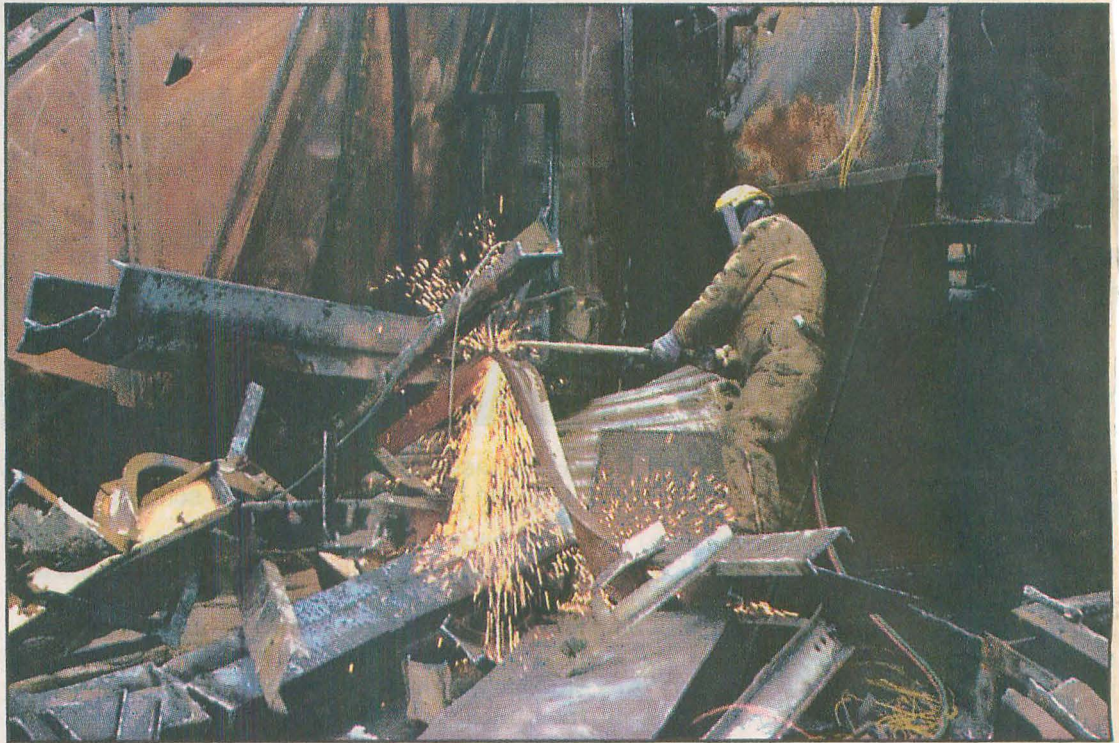
STAFF PHOTO BY CHAD McCLURE An employee of D.H. Griffin Wrecking Co. Inc. begins demolishing Wheland Foundry on Tuesday. The work is expected to take several months.
