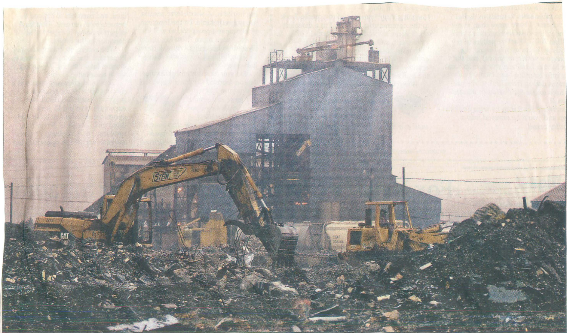
Stein Construction workers break up concrete on the site of the former Wheland Automotive Industries' Broad Street Foundry. U.S. Pipe & Foundry looms in the background.
