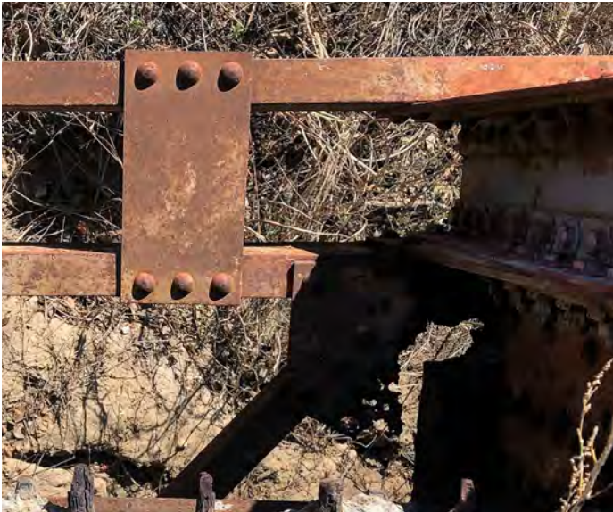
The corrosion is severe, but isolated, in several of the below-deck components such as this gusset plate which has significant section loss.
