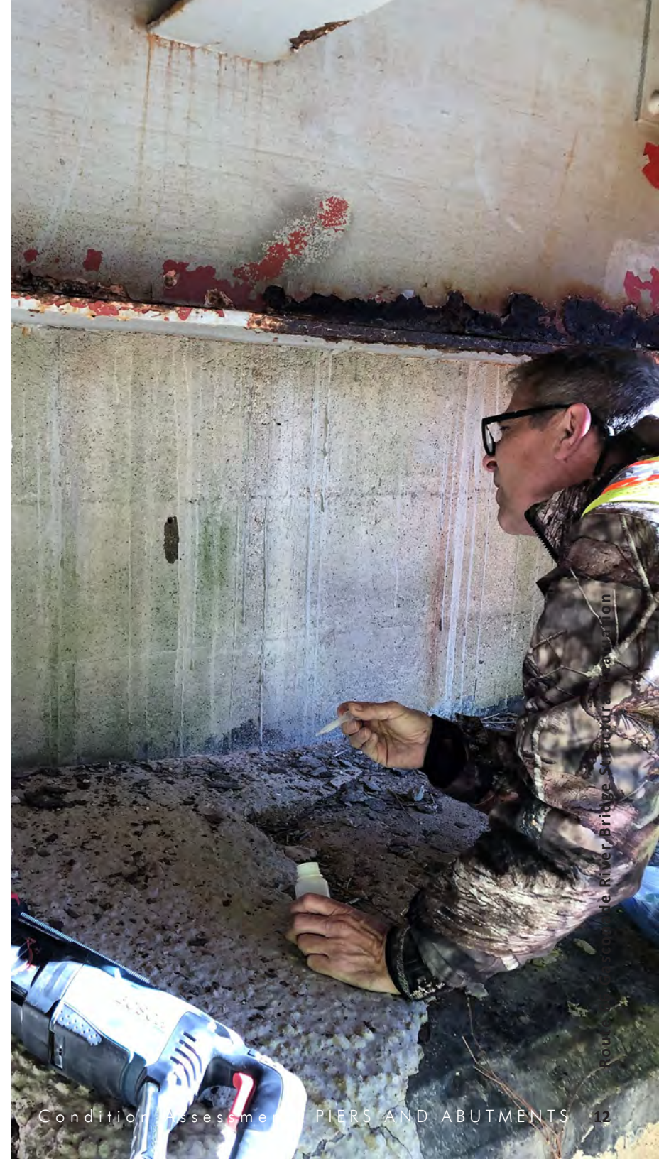
The concrete abutments are in good condition. Our concrete testing found the abutments are lightly reinforced and the depth of carbonation is ½ to 1-inch.
