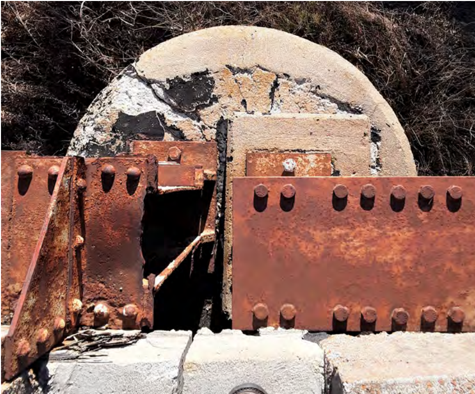
The exposed concrete at the top of the piers exhibit some cracking and deterioration which require repair.
