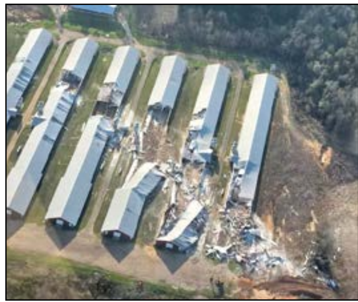
Chicken houses in Wayne County were severely damaged by Tuesday's severe weather. This photo, taken from an airplane by Keith Boyles, was sent to the LL-C by Ken Keyes.
