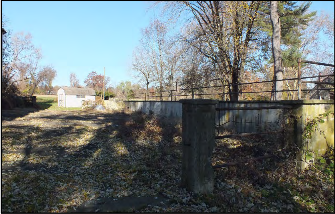
Photograph 21. Area in front of the east elevation of the Pennsylvania Barn, facing north (November 2023).
