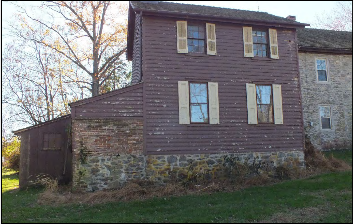
Photograph 9. North elevation (back) of the east addition to the farmhouse, facing south (November 2023).
