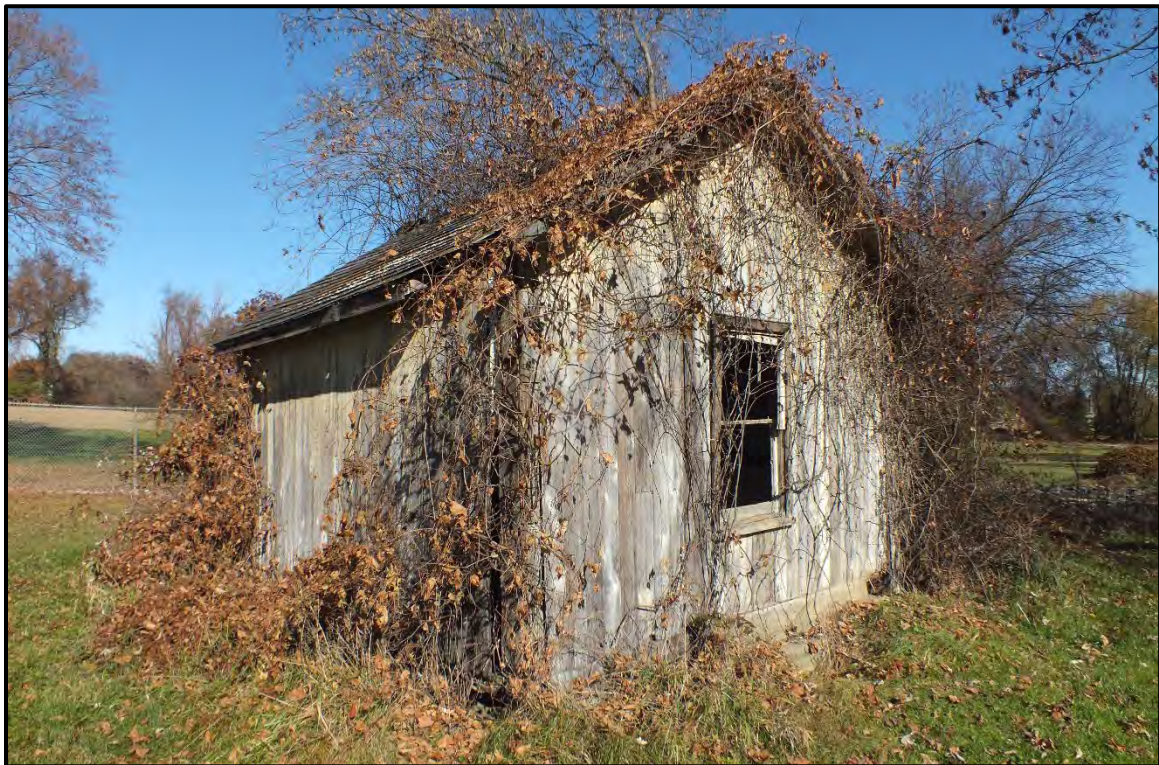
Photograph 32. West elevation (back) and south elevation (side) of the shed, facing north (November 2023).
