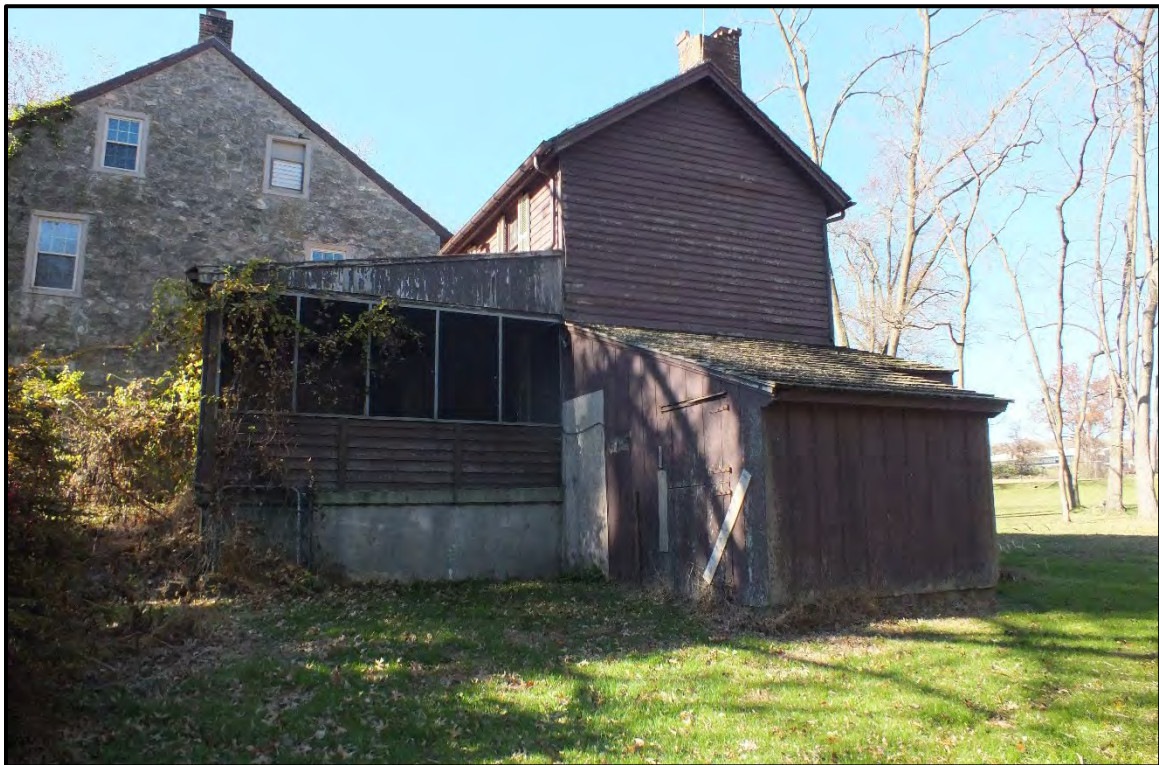
Photograph 8. East elevation (side) of the east addition to the farmhouse, facing northwest (November 2023).
