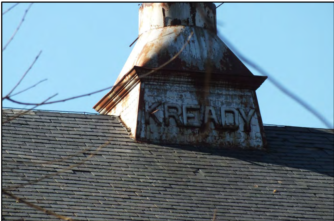
Photograph 20. View of the roof topper on the Pennsylvania Barn, facing southwest (November 2023).
