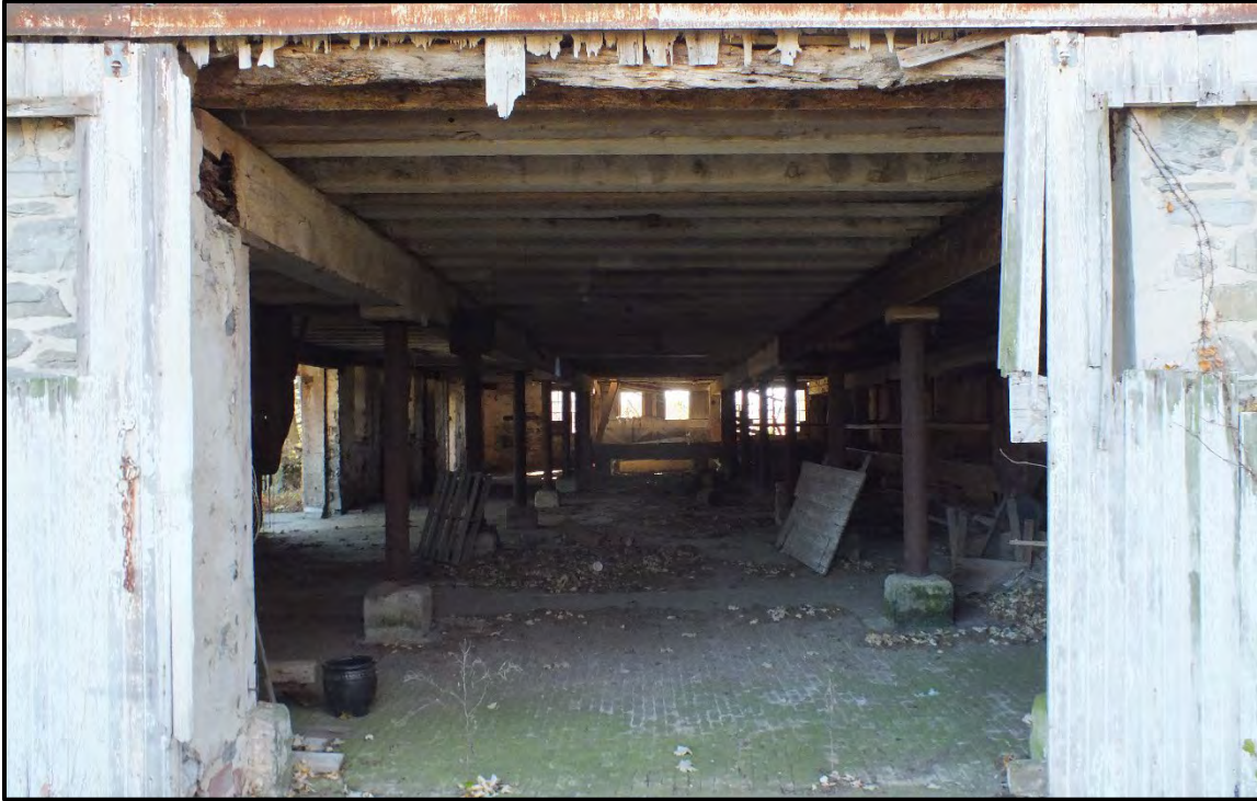
Photograph 23. View of the interior space of the lower level of the Pennsylvania Barn, facing southwest (November 2023).
