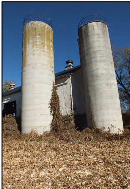
Photograph 28. View of the silos located south of the Pennsylvania Barn, facing north (November 2023).
